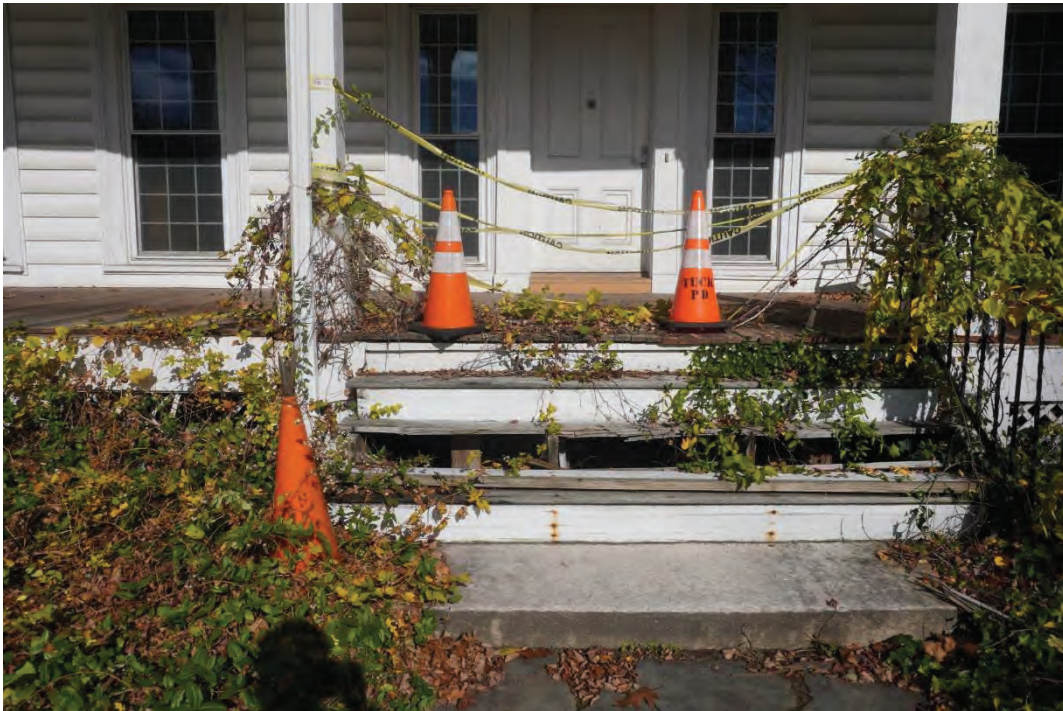
Photo #35: Rear porch stairs deteriorated. No longer usable. Unsafe condition.
