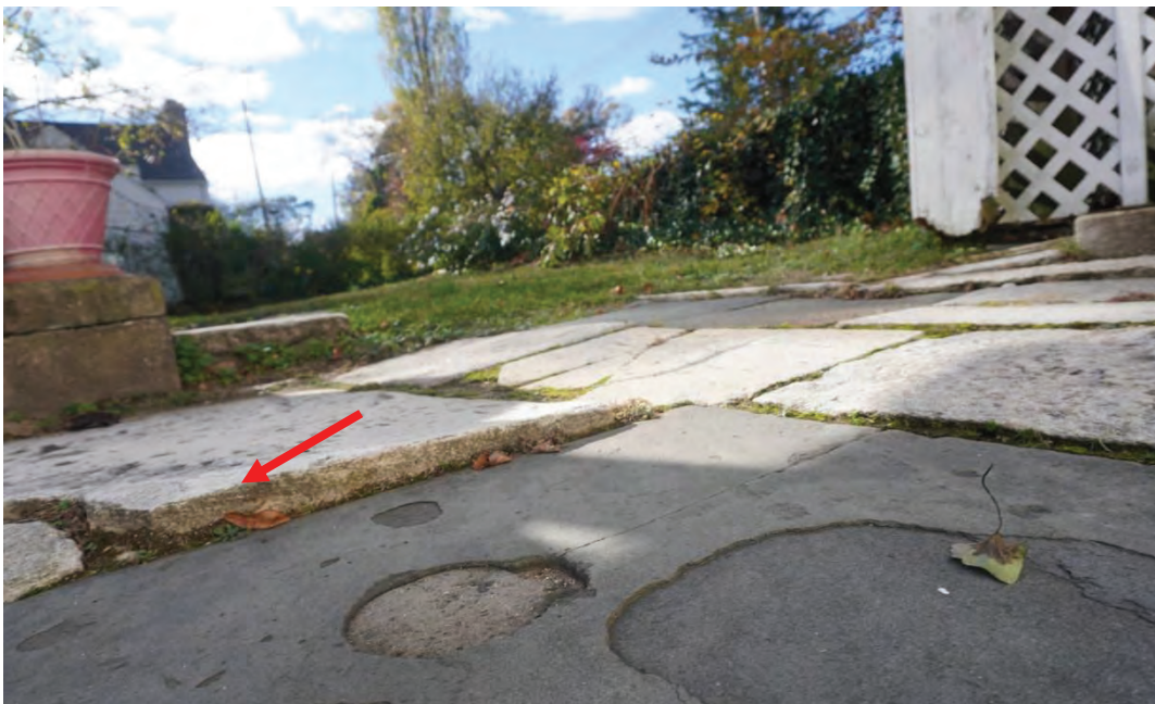
Photo #10: Stone slabs have settled/ heaved creating multiple trip hazards, stone patio rear yard.
