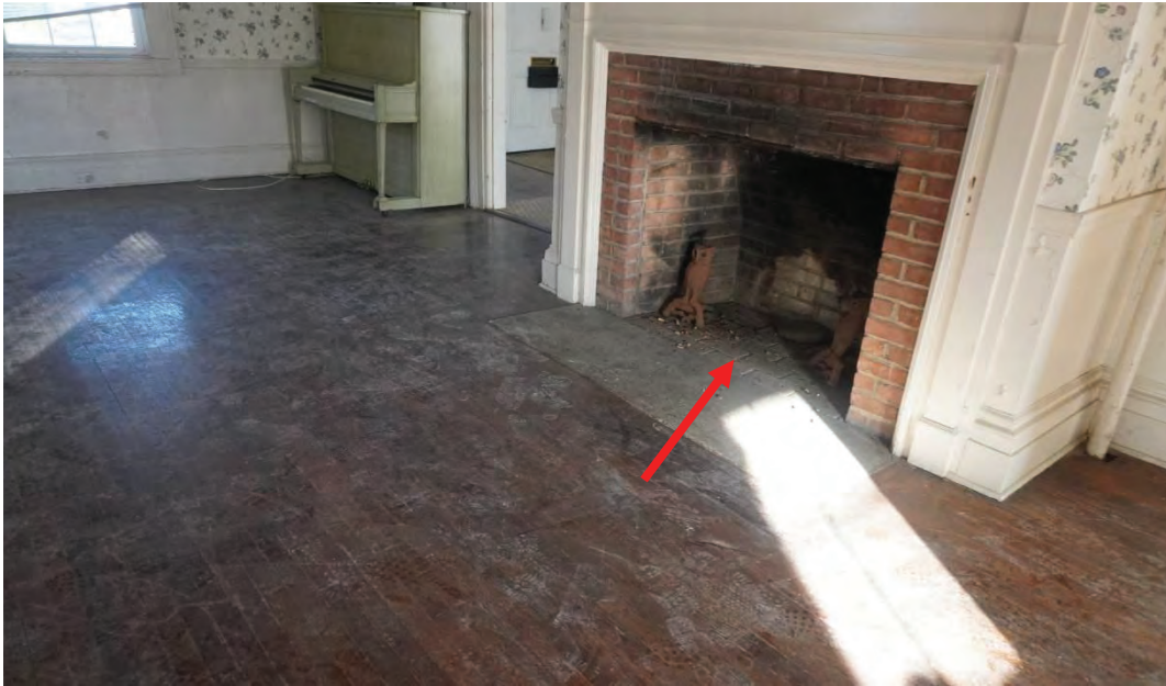
Photo #77: Chimney was added to this location at some unknown point in the past. Presumably when the original west chimney was demoed.
