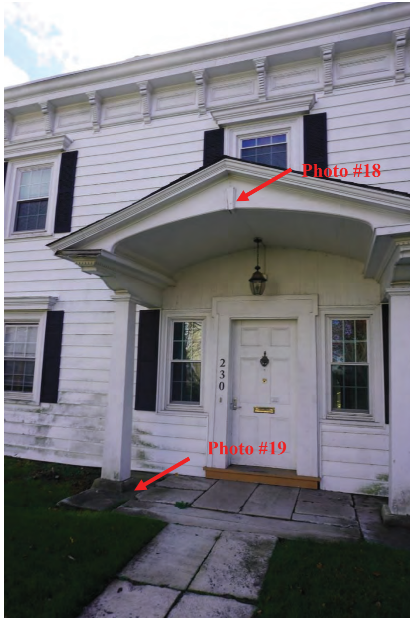
Photo #17: Base of column support for front portico showing signs of differential settlement. Vertical crack running down middle of front portico.
