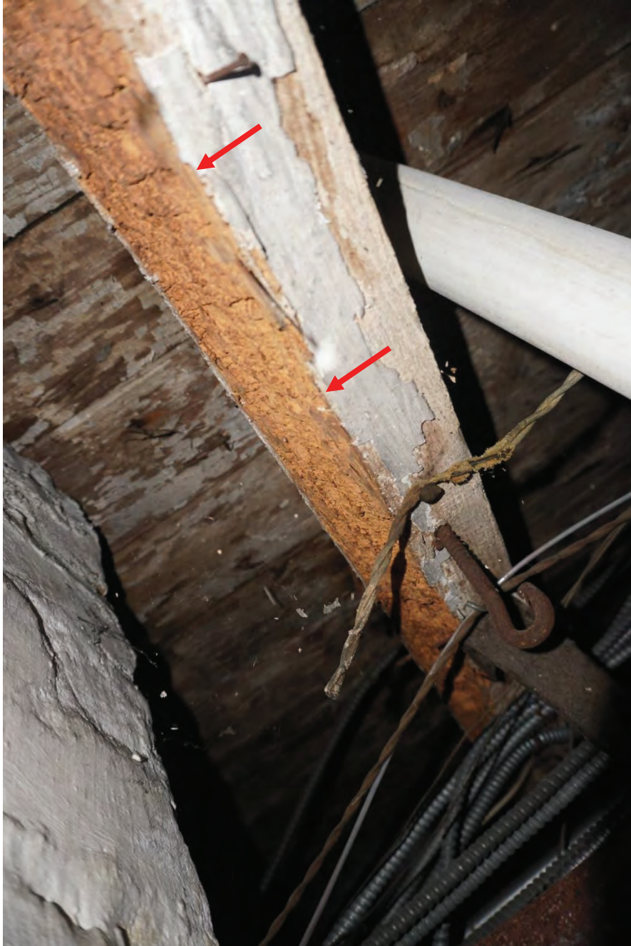
Photo #52: Wood joist observed to have a large extent of termite damage.
