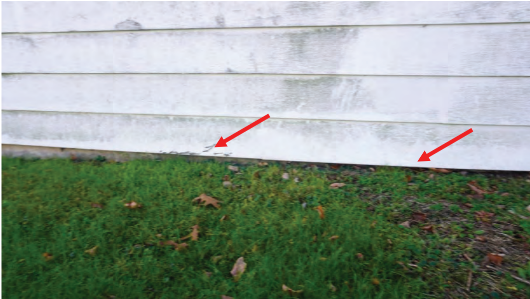
Photo #15: Foundation along front façade of original structure is low and at same level as grading. Water can infiltrate above foundation wall and rot out wood sill beam that runs along top of foundation.
