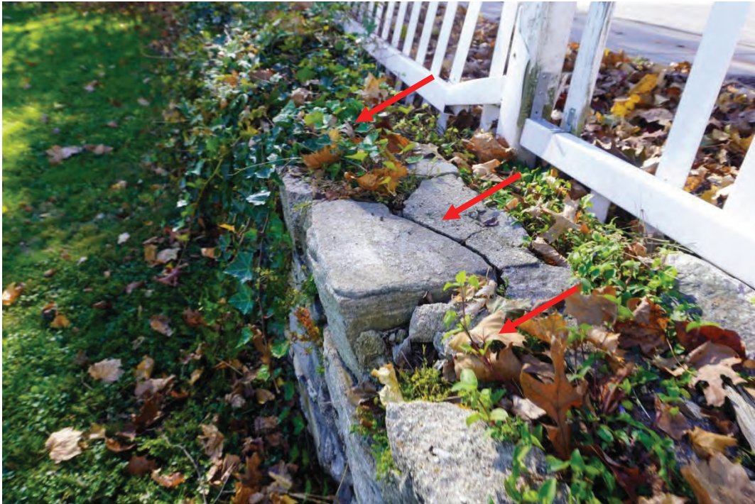
Photo #11: Retaining wall that runs between rear yard and adjacent sidewalk deteriorating throughout. Broken stones and joints between stones have filled with dirt/ organic growths.
