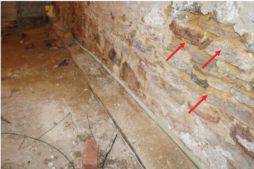
Photo #47: Water infiltrating through foundation is bringing in soil through spaces between dry laid rubble stone walls. Soil piling along inside of foundation walls.
