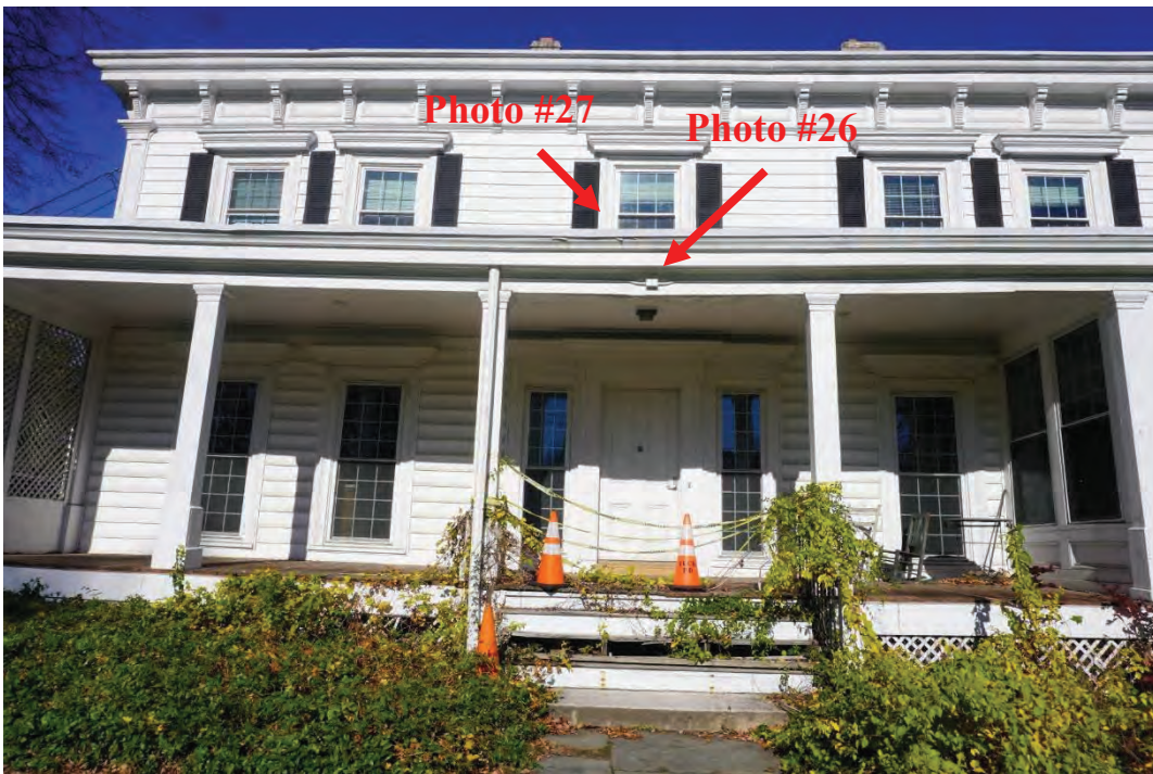
Photo #25: Rear porch roof deflecting over stairs causing water to pool and leaf build up.
