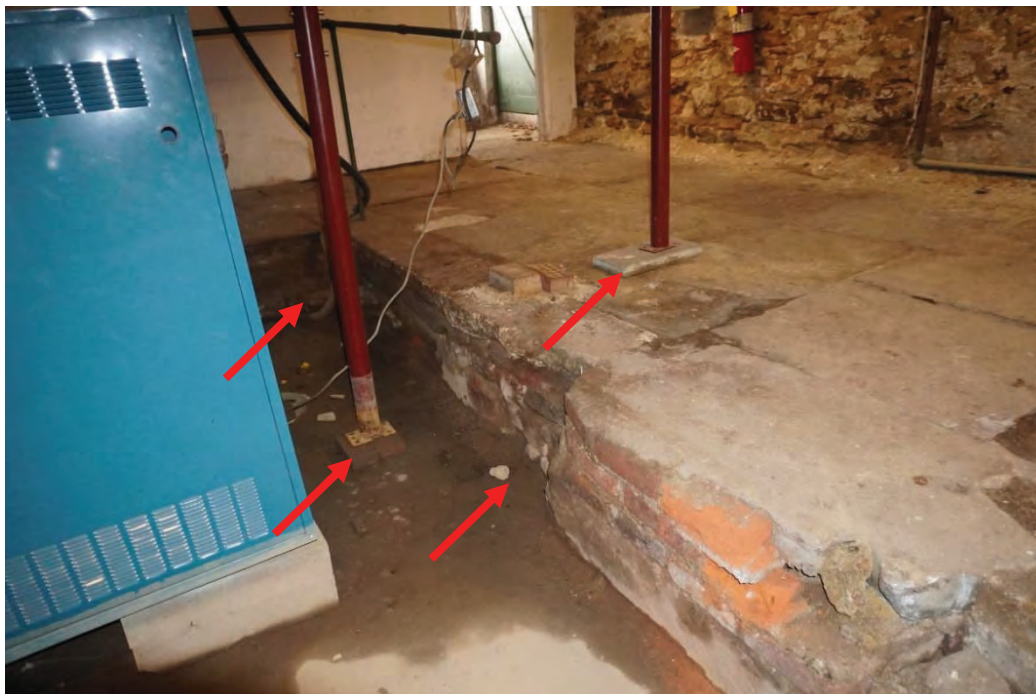
Photo #43: Water infiltration through foundation floor around perimeter of boiler pit. Concrete footings were never poured beneath temporary support columns that were added to prop up both failing girders in the cellar.
