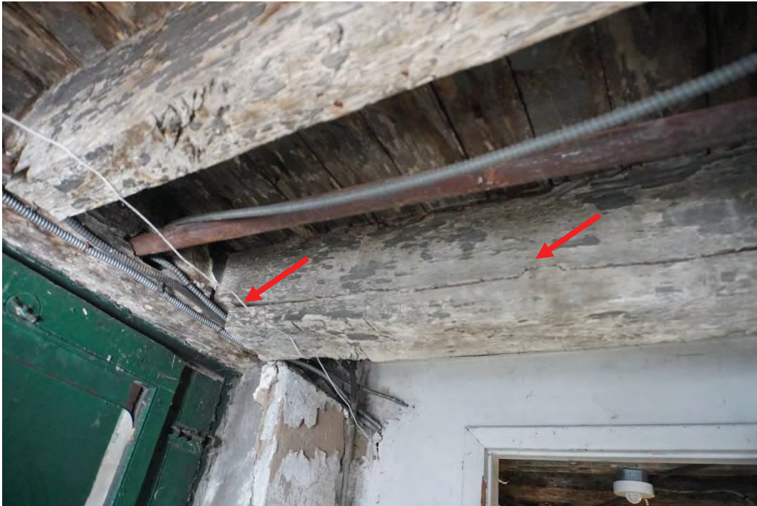
Photo #50: Horizontal crack from shear stress resonating down entire member from notch at end of beam.
