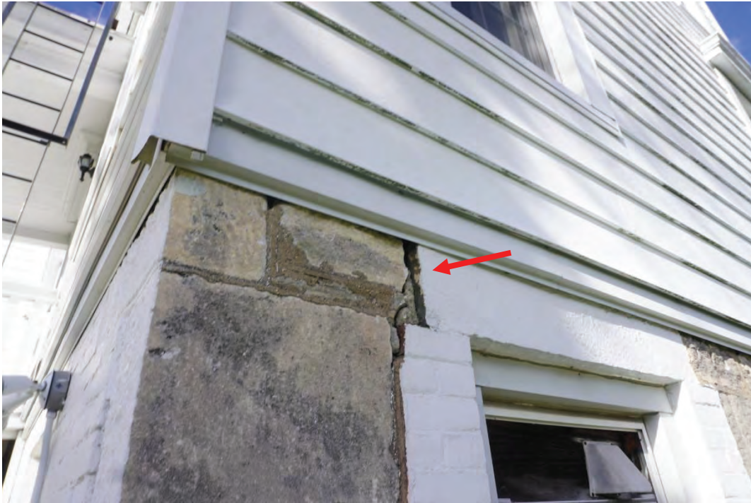
Photo #24: Vertical crack ground level stonework east façade, southeast corner of structure at addition.
