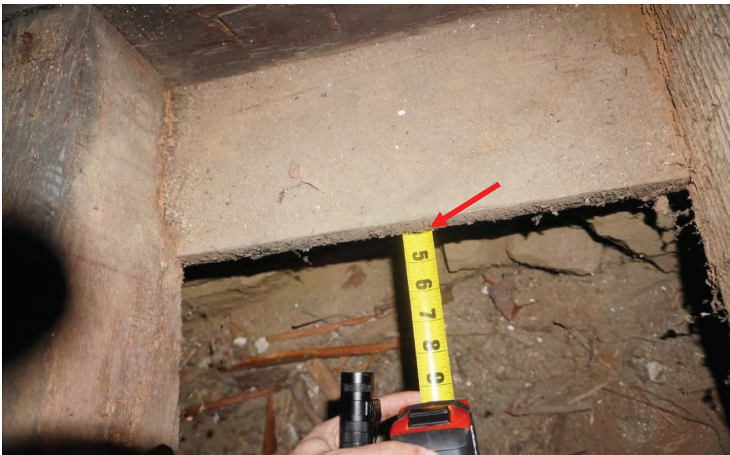
Photo #72: Crawl space joists sit on a 7-inch sill plate that is only bearing 3 inches onto deteriorating foundation wall below. Sill plate has a four-inch unsupported overhang (Probe #1).
