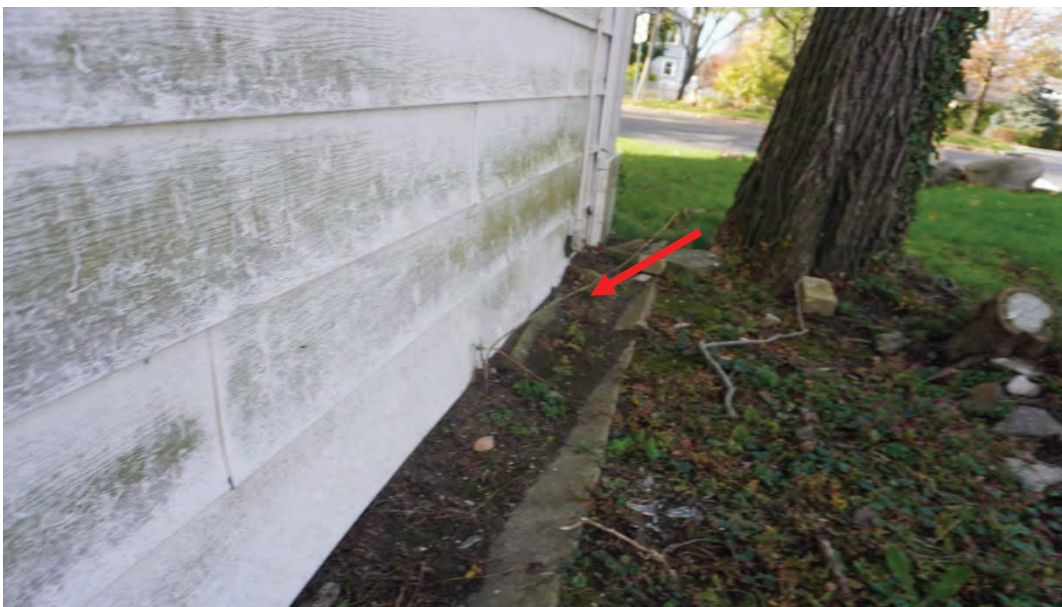
Photo #6: Negative grading front of home between entrance and northwest corner of home. Water pooling up against exterior foundation wall of crawlspace.
