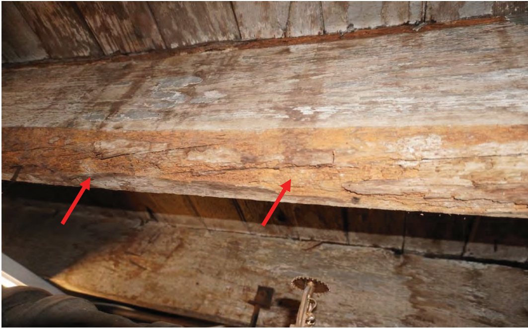
Photo #61: Wood joist observed to have a large extent of termite damage.
