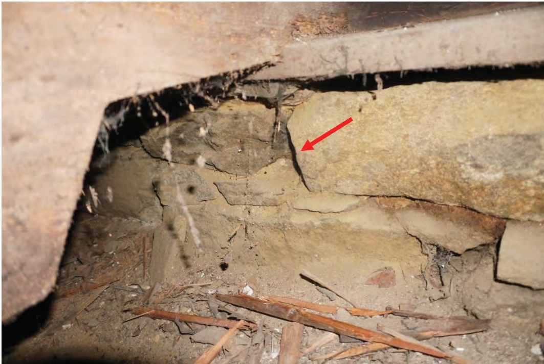
Photo #68: Thin sill plate, joists spanning crawlspace are sitting on, is being supported by a rubble stone foundation wall that is coming apart (Probe #1).
