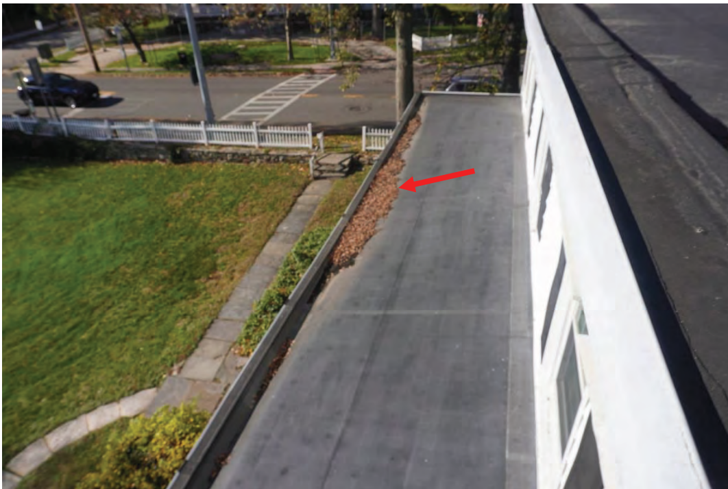
Photo #27: Rear porch roof deflecting over stairs causing water to pool and leaf build up.
