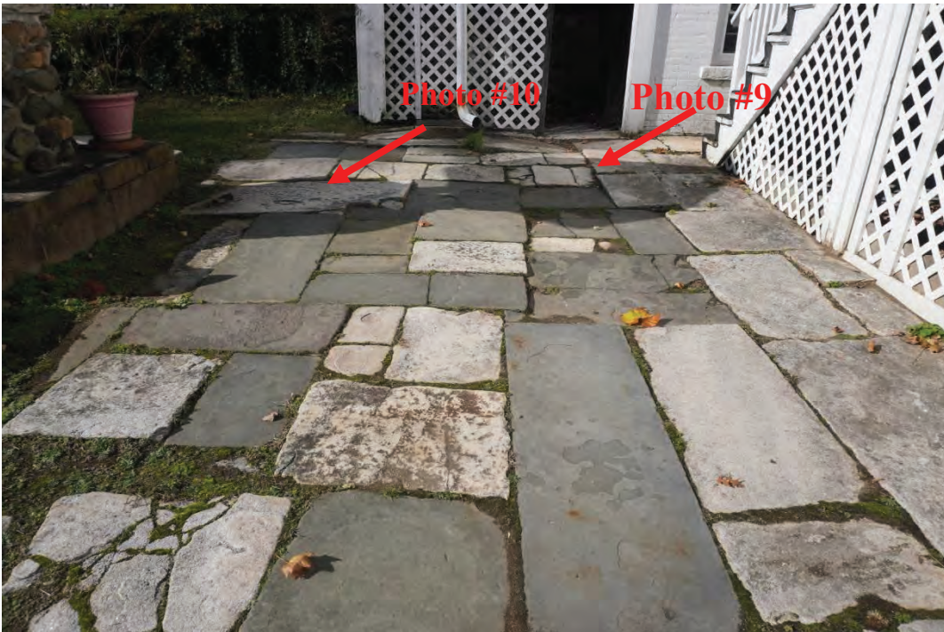
Photo #8: Stone slabs have settled/ heaved creating multiple trip hazards, stone patio rear yard.
