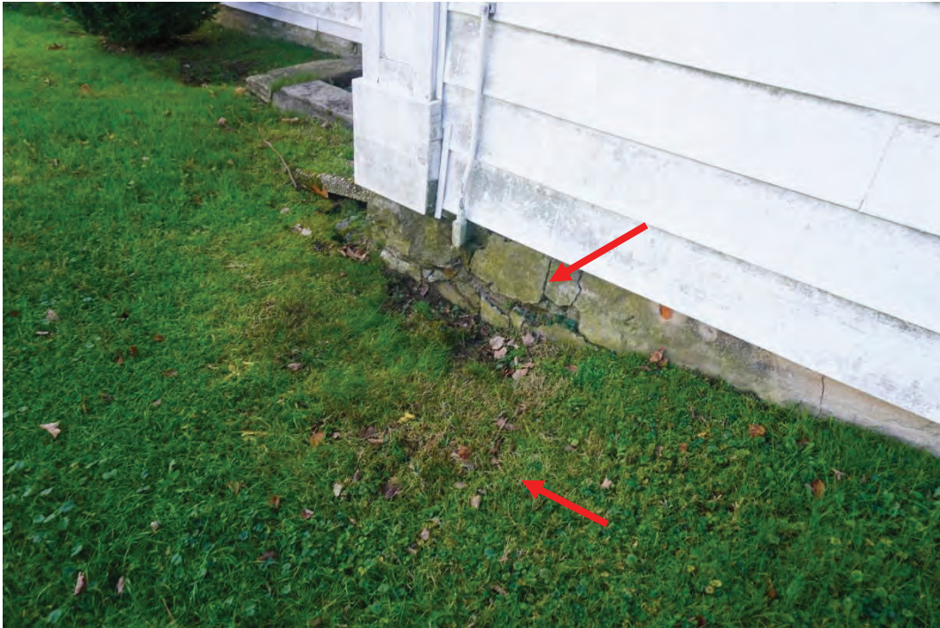
Photo #5: Negative grading front of home between entrance and northeast corner of home. Water pooling up against foundation wall and most likely infiltrating into crawlspace. Signs of foundation deterioration.
