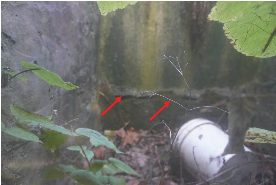
Photo #41: Horizontal crack has formed in concrete window well, north façade.
