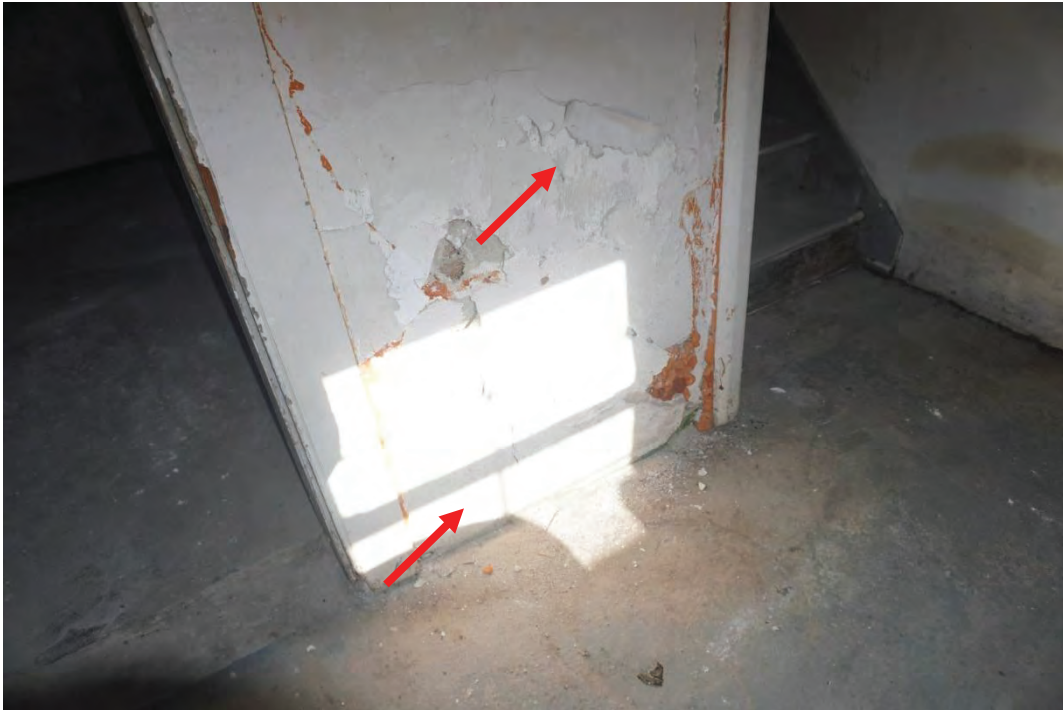
Photo #38: Mold formation and deteriorating damp plaster interior walls at cellar level due to water wicking up through cellar floor.
