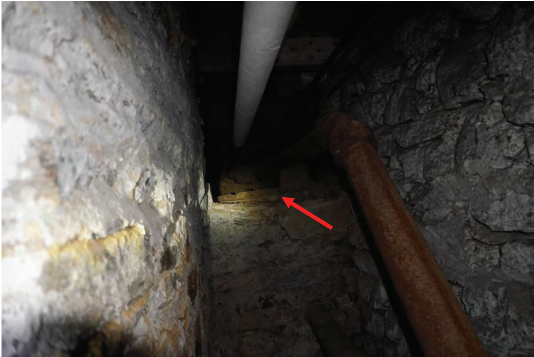
Photo #55: Piping was run into crawlspace through what potentially was an old window (second location) in original foundation wall.
