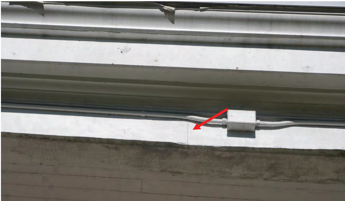
Photo #26: Rear porch roof deflecting over stairs causing water to pool and leaf build up.
