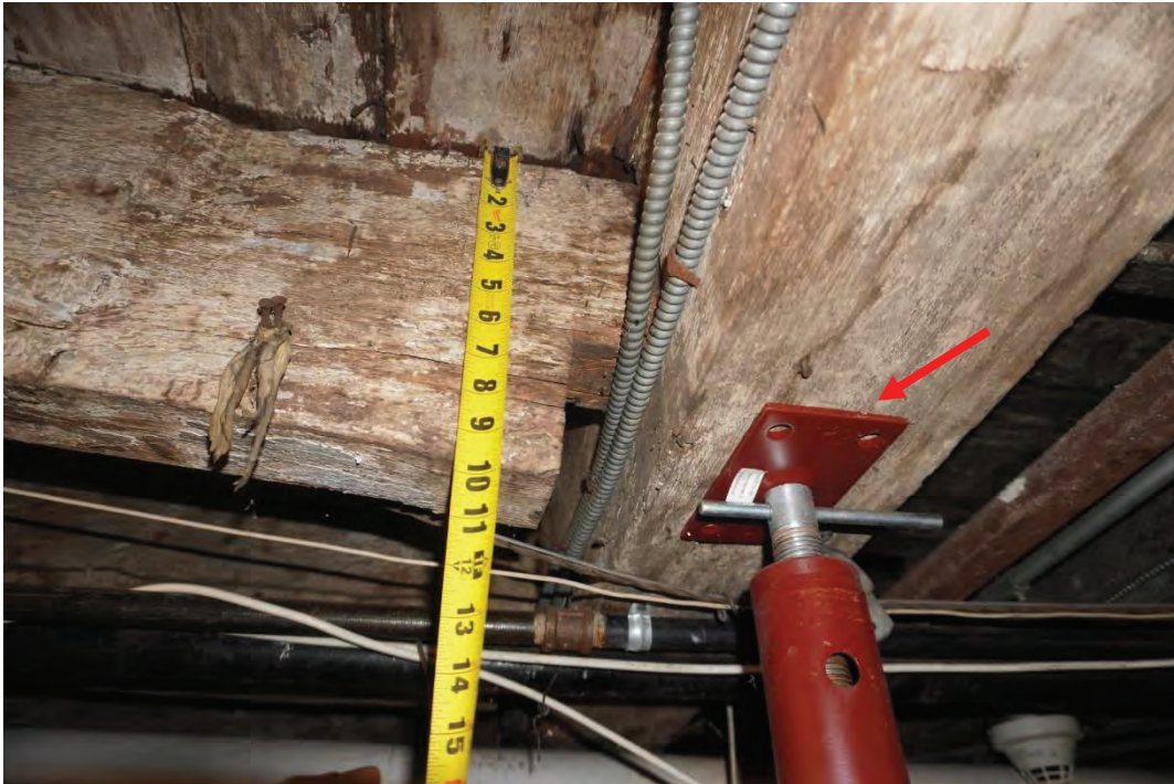
Photo #59: Temporary support column being used to hold failing 9-1/2"x9-1/4" girder in boiler room. Column not mechanically attached to girder above and does not have a proper footing.
