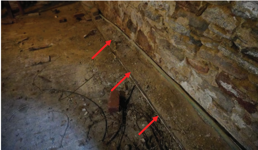
Photo #46: Water infiltrating through foundation is bringing in soil through spaces between dry laid rubble stone walls. Soil piling along inside of foundation walls.
