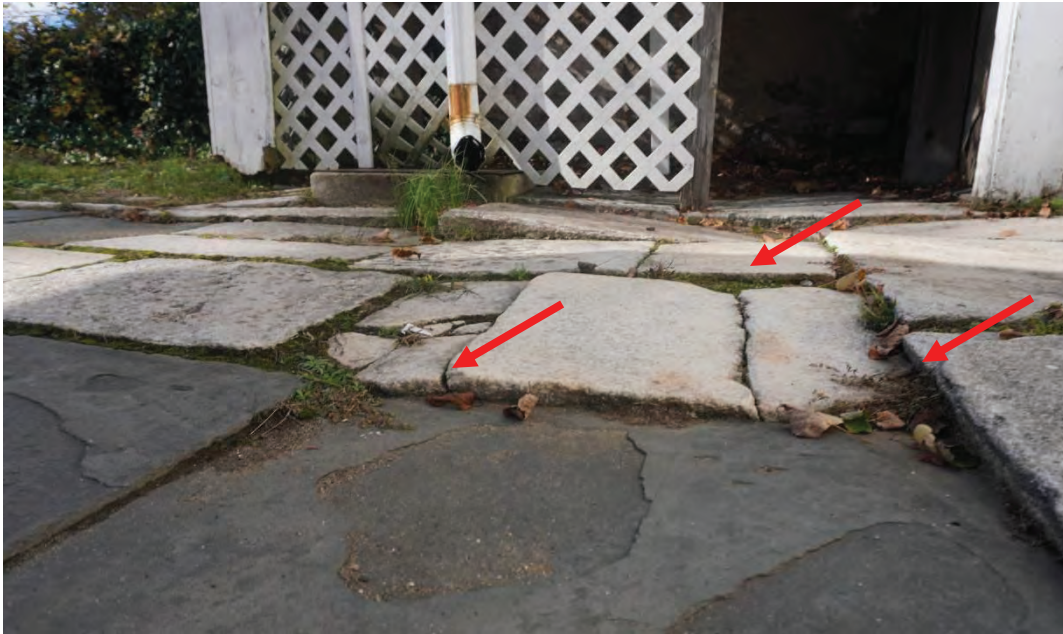
Photo #9: Stone slabs have settled/ heaved creating multiple trip hazards, stone patio rear yard.
