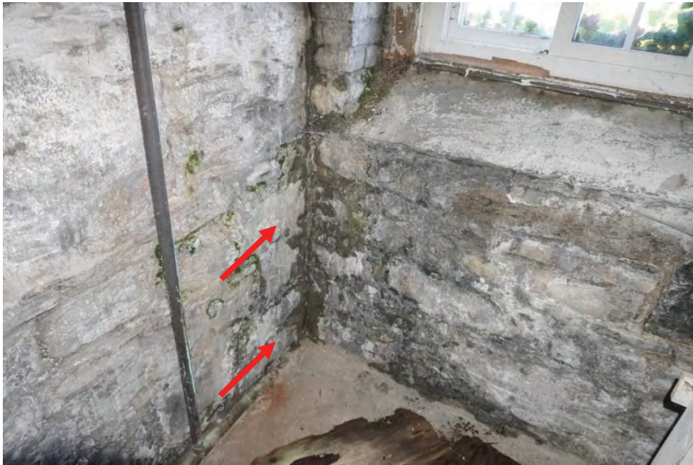
Photo #36: Water intrusion foundation wall, northeast corner of home at extension.
