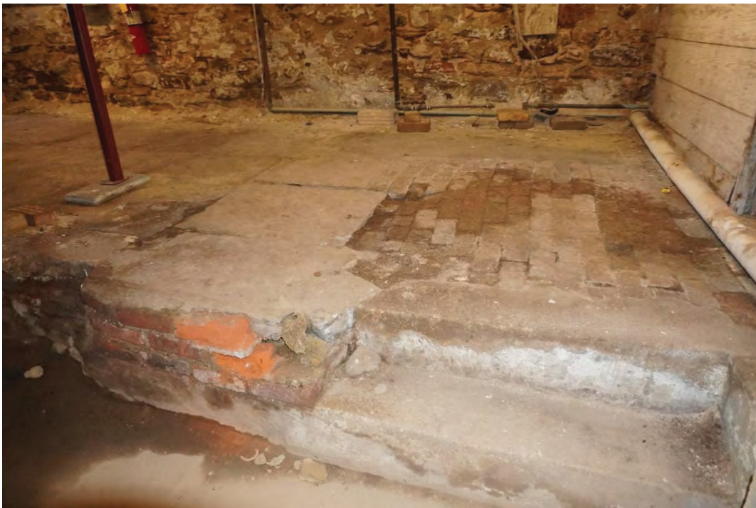
Photo #45: Cellar floor observed to be composed of bricks with a cement stucco layer that is deteriorating.
