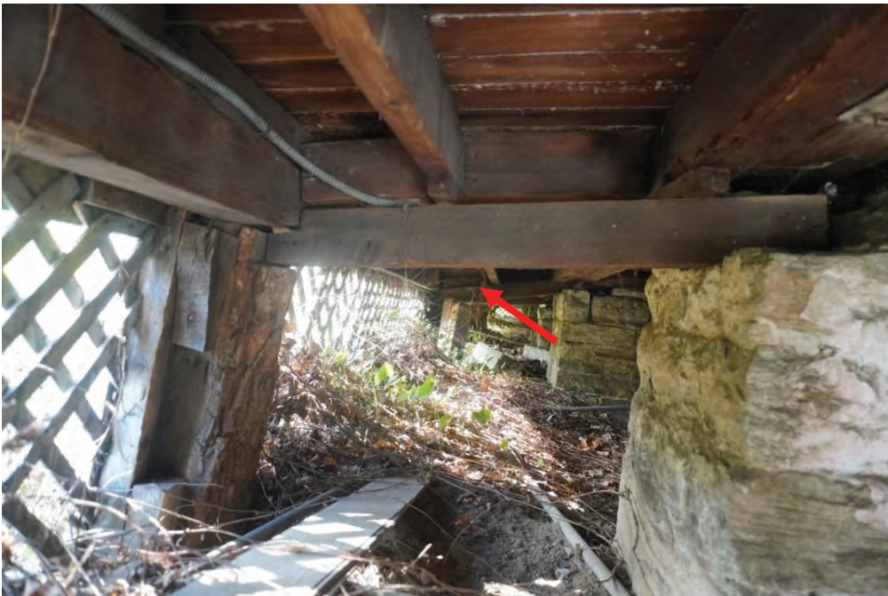
Photo #33: Rear porch was extended to be made wider at some unknown time in the past.
