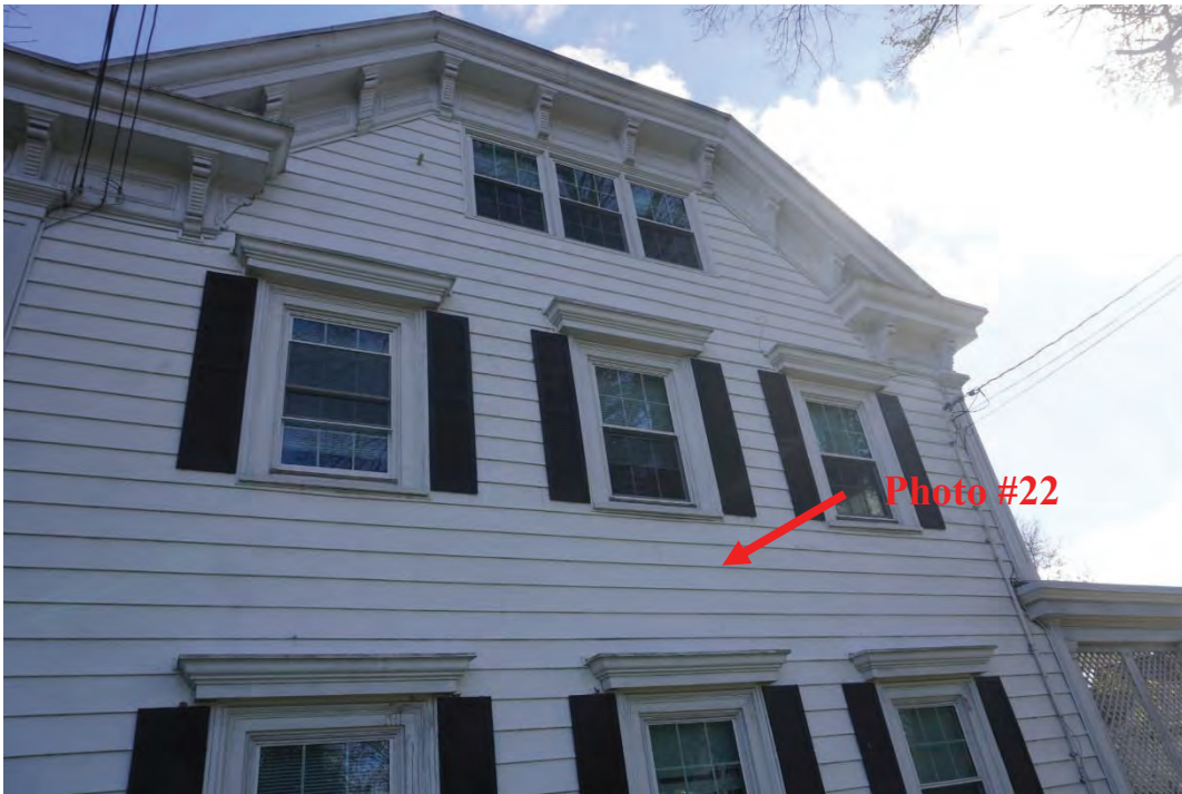
Photo #21: Bulge noticed between first and second floors, west façade of home. Cause unknown. Further investigation required.
