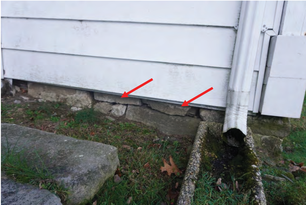
Photo #20: Exposed exterior side of rumble foundation deteriorating. No mortar between stones.
