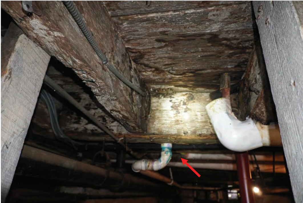
Photo #63: Plumbing pipe drilled directly through main girder in the vertical direction, west end of cellar.
