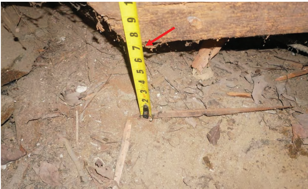
Photo #74: Wood joists in crawlspace are sitting 7 inches above exposed dirt beneath crawlspace. Crawlspace is inaccessible. Crawlspace foundation most likely does not extend below the frost line (Probe #1). Further investigation required.
