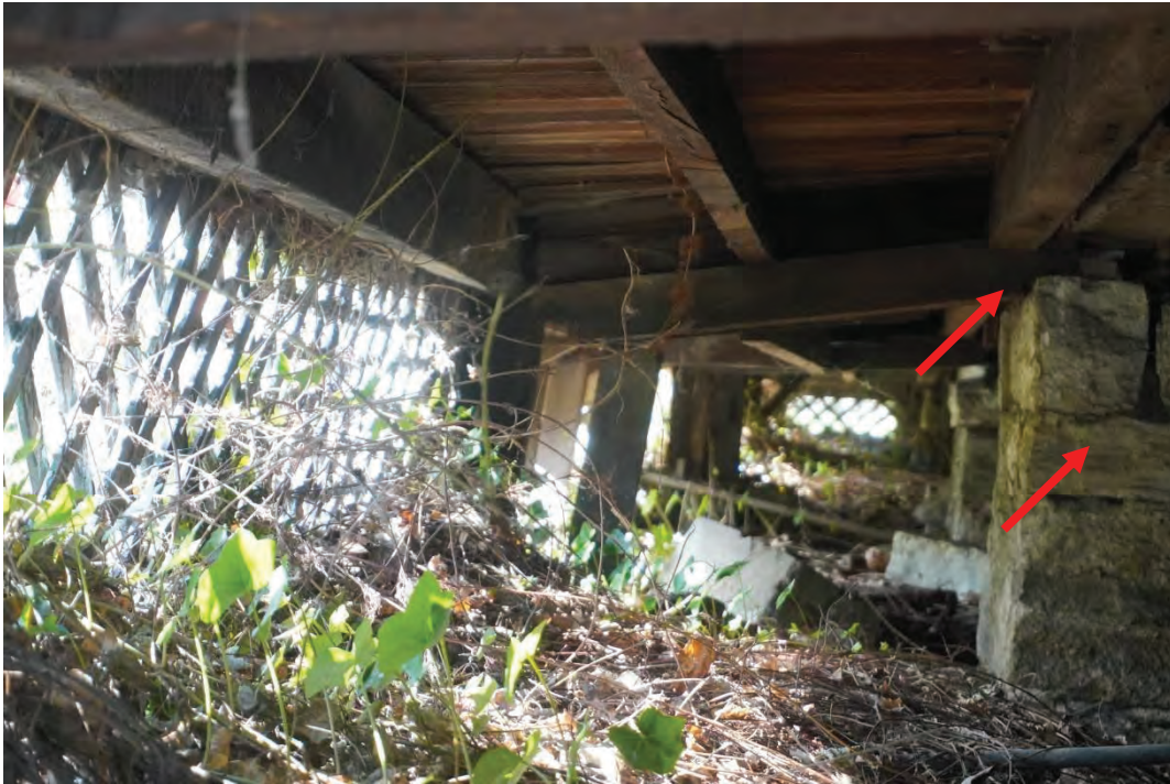
Photo #34: Rear porch sitting on stone pillars that are showing signs of deterioration.
