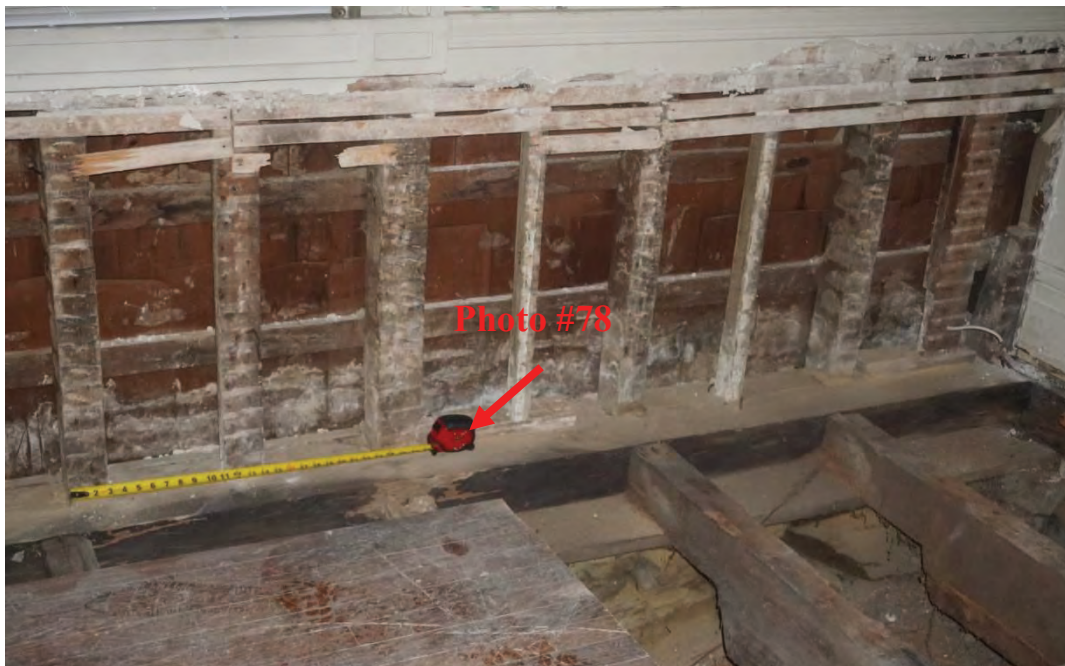
Photo #78: Vertical exterior framing members spaced at approximately 10 to 11 inches apart along west façade sitting on sill beam (Probe #1).
