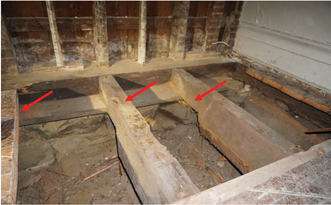
Photo #67: Joists spanning crawlspace sit on a thin sill plate which is not a standard timber framing technique. Typically, wood joists would be notched into the sill beam with use of a mortise and tenon connections (Probe #1).
