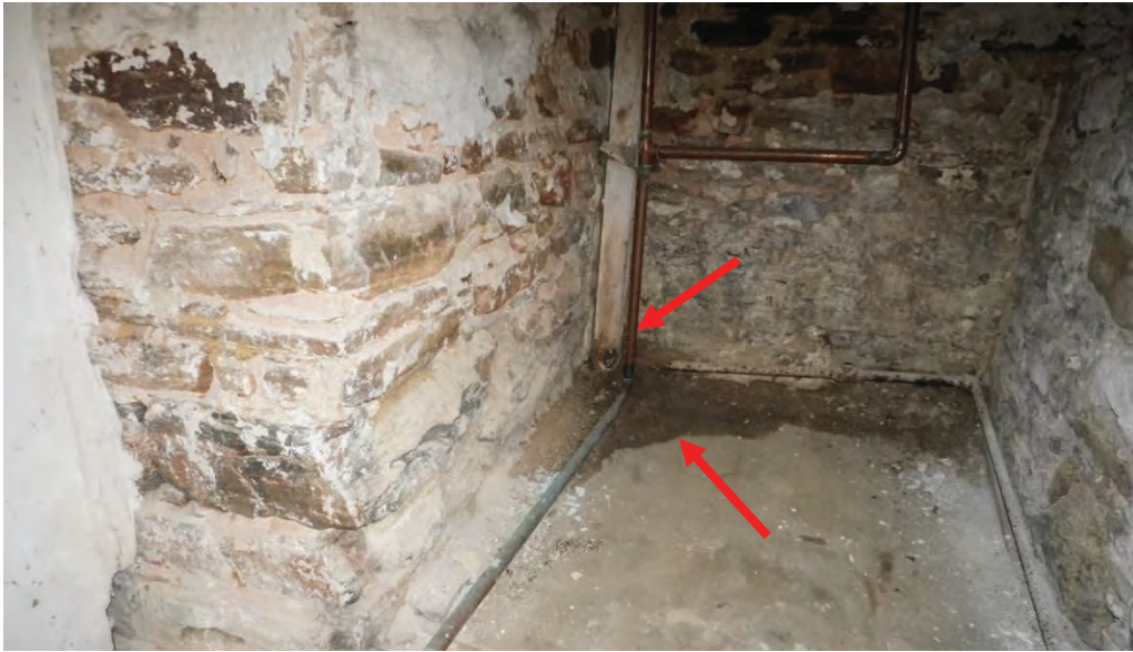
Photo #42: Water infiltration at base of inner, original foundation wall. Water is rotting base of wood support post. Crawlspace that spans the front side of the home is located on the other side of this wall.
