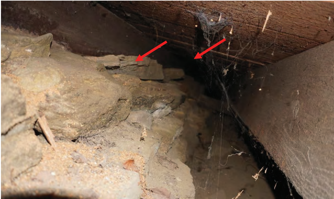
Photo #73: Exterior foundation along north side of home below sill beam is deteriorating and observed to have displaced. (Probe #1)
