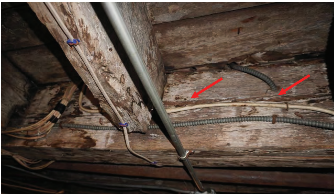
Photo #60: Large horizontal crack in 9-1/2"x9-1/4" girder in boiler radiating from mortise-and-tenon joint connections.
