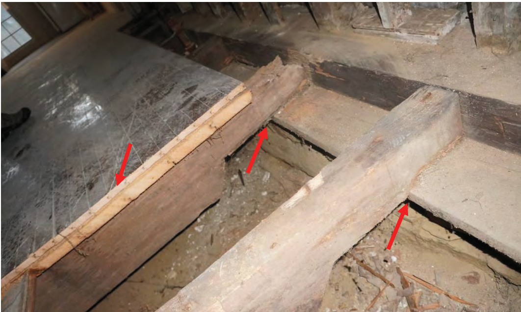
Photo #70: Original floorboards above crawlspace have been removed. New wood flooring directly attached to joists. Crawl space joists sitting on an improperly supported sill plate (Probe#1).
