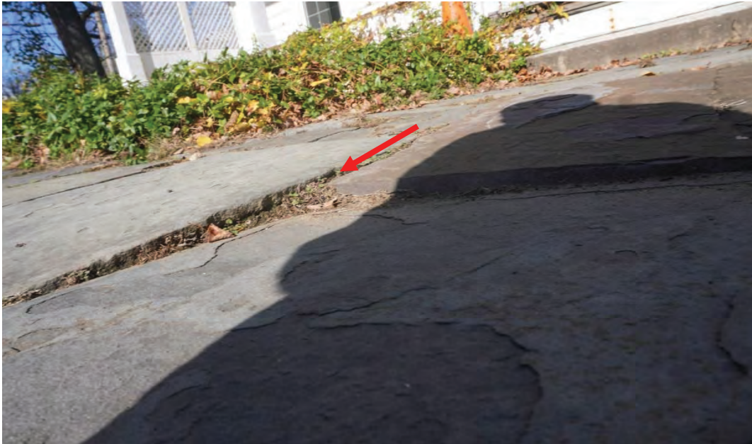
Photo #7: Stone slabs have settled/heaved creating multiple trip hazards, stone walkway rear yard.
