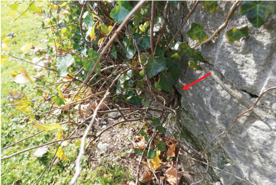
Photo #3: Retaining wall that runs from between front entrance and driveway is deteriorating throughout. Roots/ large weeds growing through joints of walls multiple locations.
