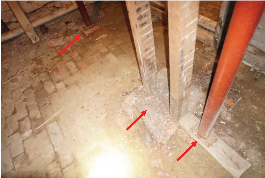
Photo #44: Concrete footings were never poured beneath temporary support columns that were added to prop of both failing girders in the cellar.
