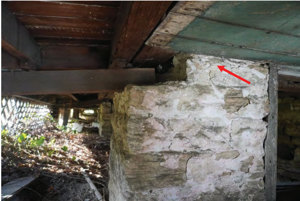
Photo #32: Rear porch sitting on stone pillars that are showing signs of deterioration.
