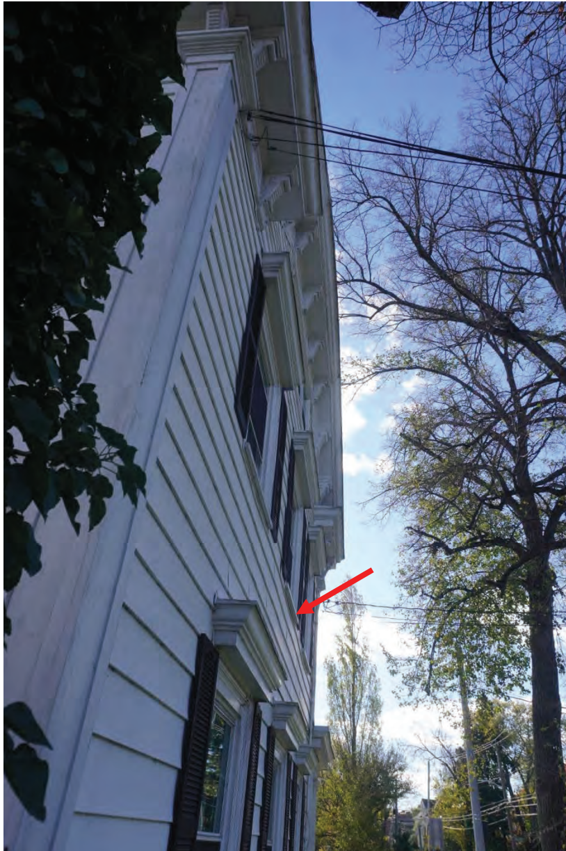
Photo #22: Bulge noticed between first and second floors, west façade of home. Cause unknown. Further investigation required.
