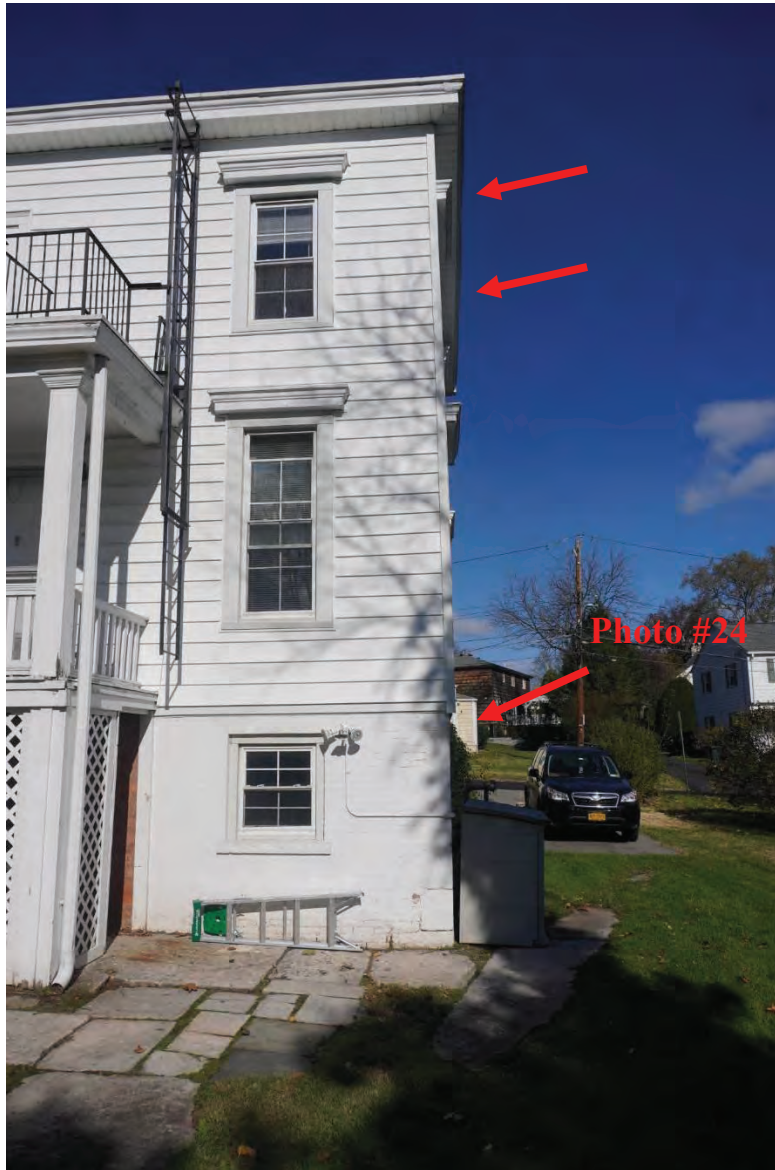
Photo #23: Southeast corner of structure showing signs of inwards movement towards the top. Cause unknown. Further investigation required.
