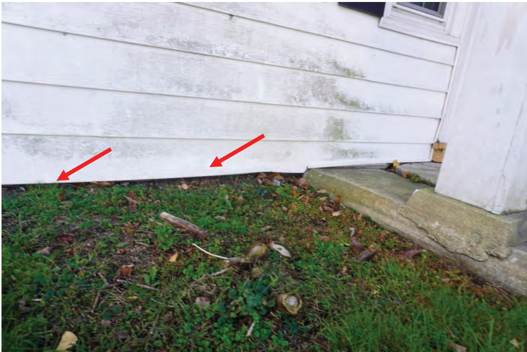
Photo #16: Foundation along front façade of original structure is low and at same level as grading. Water can infiltrate above foundation wall and rot out wood sill beam that runs along top of foundation.
