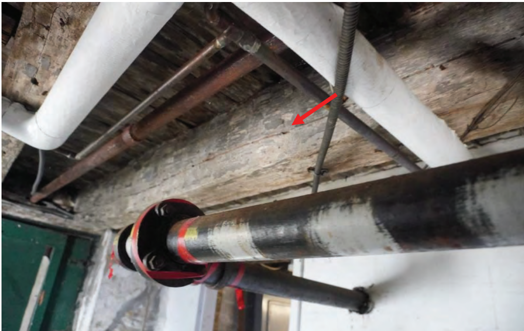
Photo #51: Horizontal crack from shear stress resonating down entire member from notch at end of beam.
