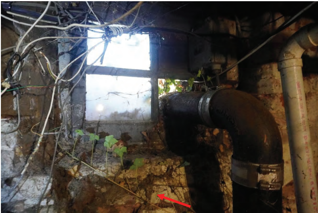
Photo #56: Dirt and soil infiltrating around window in cellar at west foundation wall.
