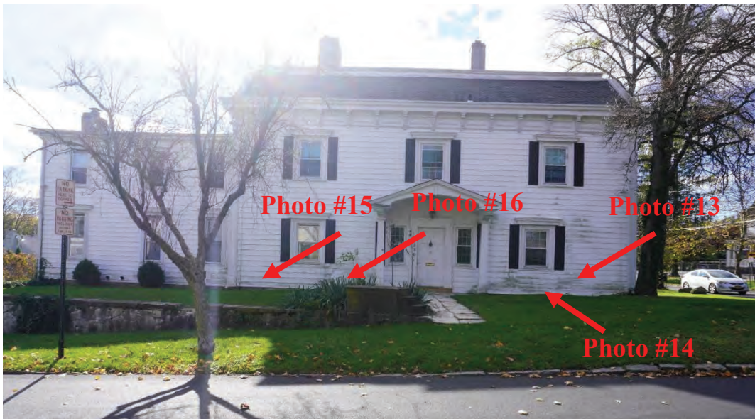
Photo #12: Foundation along front façade of original structure is low and at same level as grading. Water can infiltrate above foundation wall and rot out wood sill beam that runs along top of foundation.
