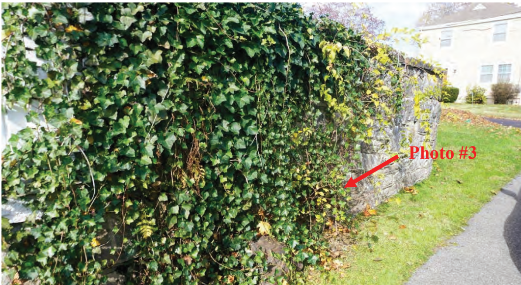
Photo #2: Retaining wall that runs from between front entrance and driveway is deteriorating throughout. Roots/ large weeds growing through joints of walls multiple locations.
