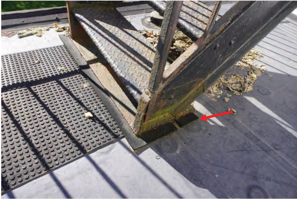
Photo #30: Exterior metal stair egress just sitting on roofing membrane and not attached to structure.
