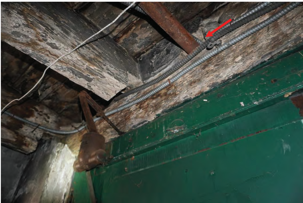
Photo #49: Pipe penetration drilled through door header leading out to rear yard.
