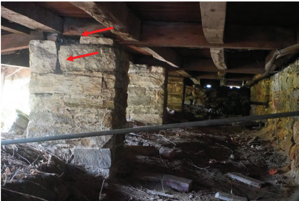
Photo #31: Rear porch sitting on stone pillars that are showing signs of deterioration.
