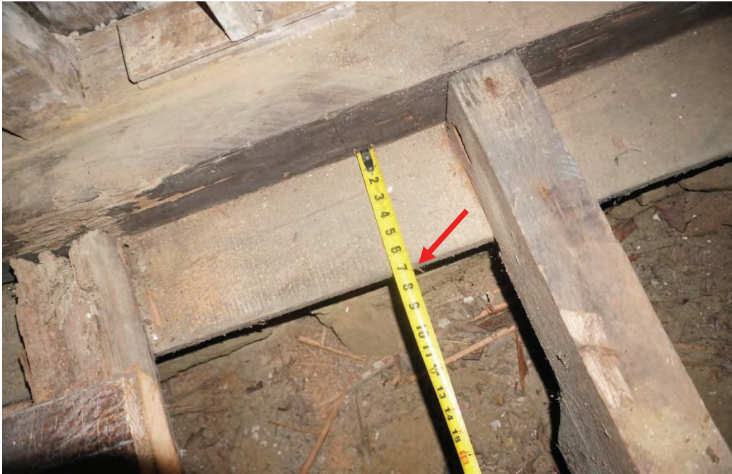
Photo #71: Crawl space joists sit on a 7-inch sill plate that is only bearing 3 inches onto deteriorating foundation wall below. Sill plate has a four-inch unsupported overhang (Probe #1).
