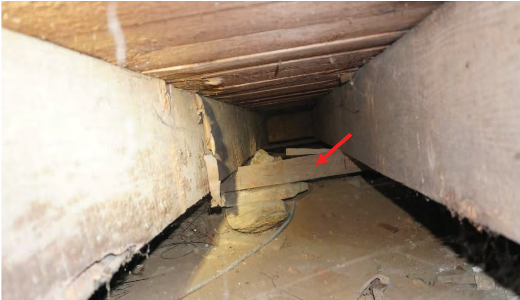
Photo #75: Wood joists spanning crawl space are being inadequately supported at midspans by wood members that are balanced above unstable pieces of stone (Probe #1).
