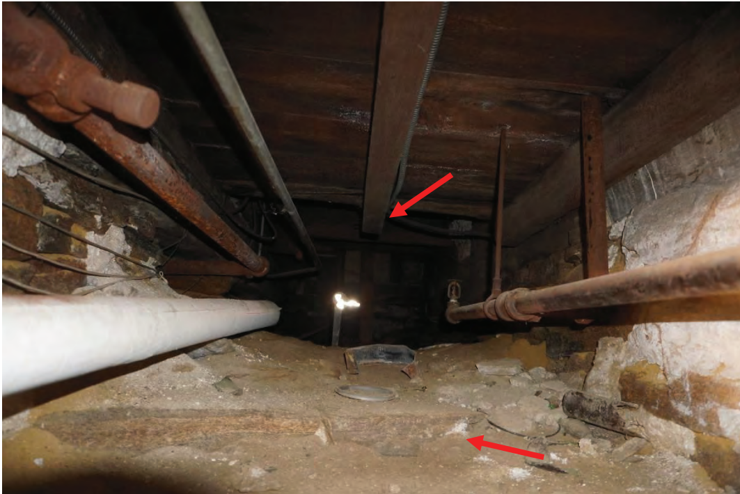
Photo #53: Joists connections in crawlspace observed to be coming apart. Piping was run into crawlspace through what potentially was an old window in original foundation wall.
