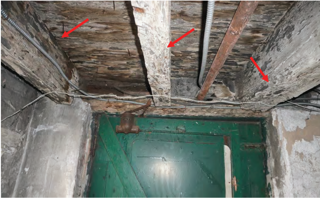
Photo #48: Two 10x3 beams spaced 16 inches apart on left are spanning 19 feet. The reason 6"x9-1/4" beam on right is sized larger than other joists is unclear. It is uncommon for such a large member to be sitting on a door header.
