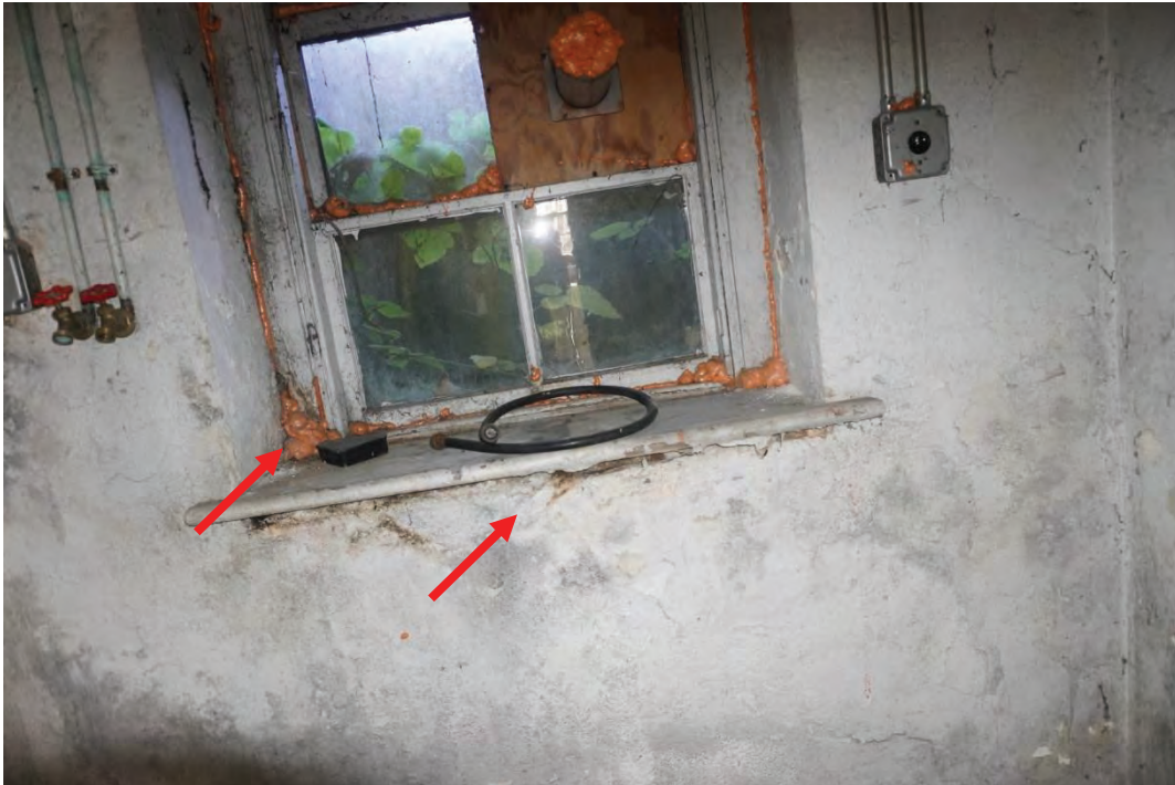
Photo #40: Water infiltration around cellar window, north façade of home at window well.
