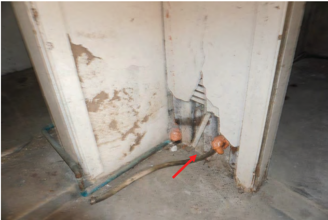
Photo #39: Mold formation and deteriorating damp plaster interior walls at cellar level due to water wicking up through cellar floor.
