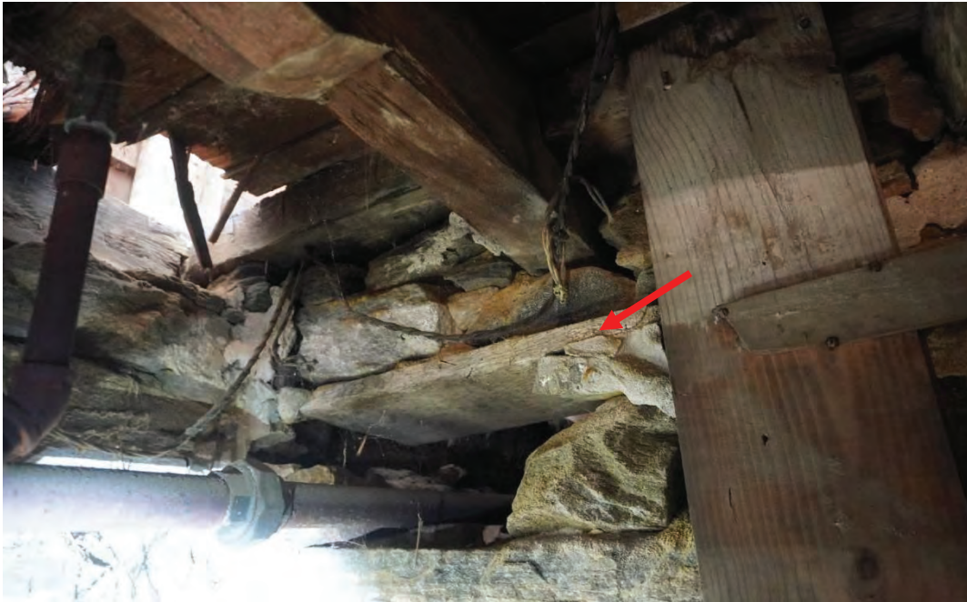
Photo #65: Joist with inadequate support resting on foundation wall that is deteriorated and that has been damaged to make a pipe penetration into crawlspace.
