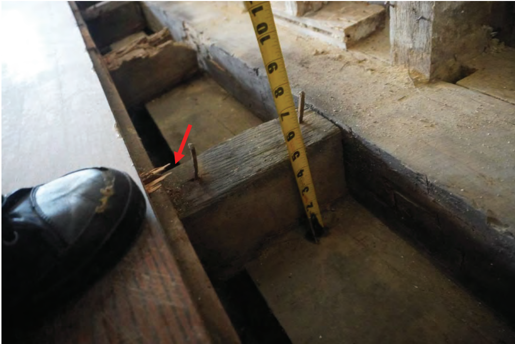
Photo #69: Original floorboards above crawlspace have been removed. New wood flooring directly attached to joists. Crawl space joists sitting on an improperly supported sill plate.
