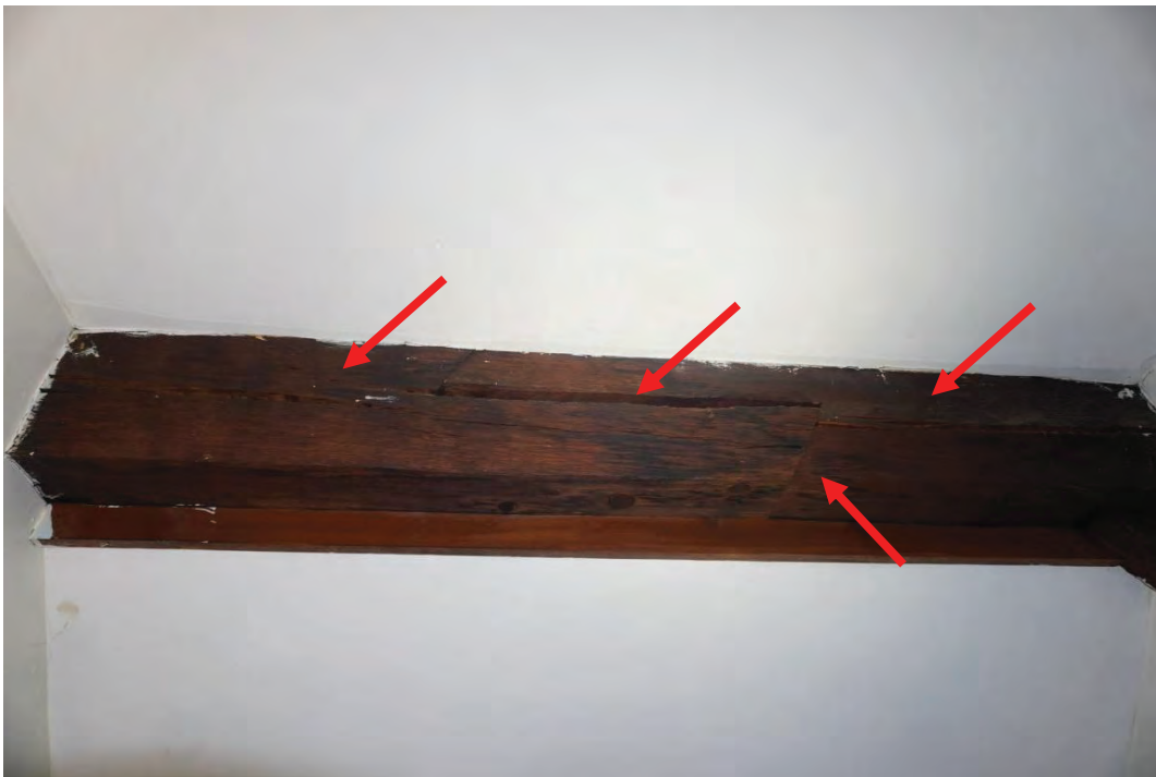
Photo #118: Roof support beam observed to be coming apart.
