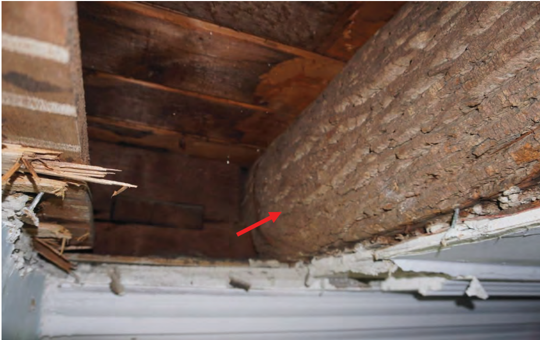
Photo #89: Ceiling joist that was never fully scored into a square framing member and still has bark exterior (Probe #4).
