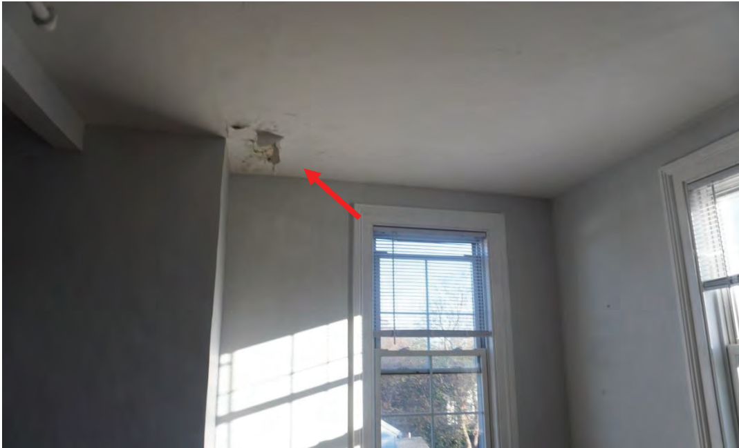
Photo #107: Water damage adjacent to east exterior wall of addition. Cause unknown, further investigation required.
