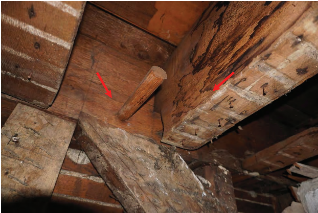
Photo #96: Mortise and tenon connection between a bracing member and interior girder being held in place with a wooden peg. (Probe #5)
