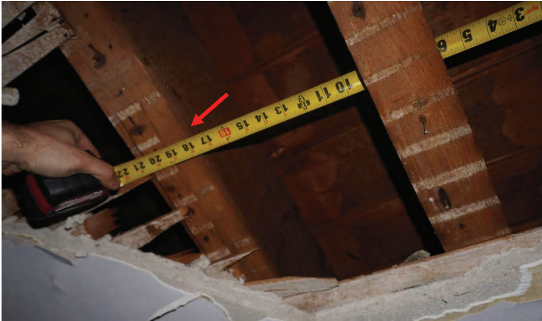
Photo #85: Joists above faux soffit are running north to south and are spaced at 18” inches apart. All other floor joists observed in the original structure above the ground level are running perpendicular to these joists (Probe #3). Further investigation required.
