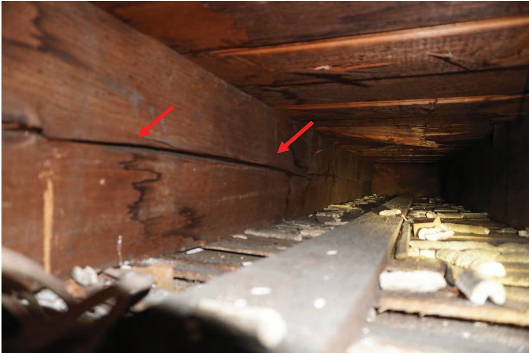
Photo #91: Large shrinkage crack that runs entire floor joist (Probe #4).
