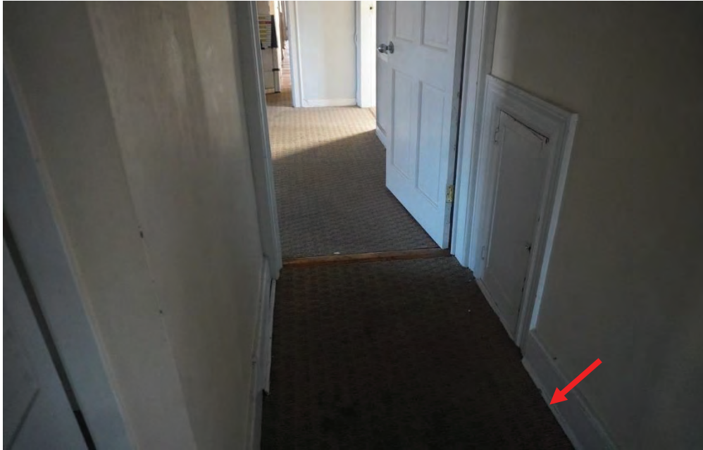
Photo #99: Depression in second floor hallway. Most likely due to weight of walls and bathroom added in this area. Further investigation would be required to figure out exact cause.
