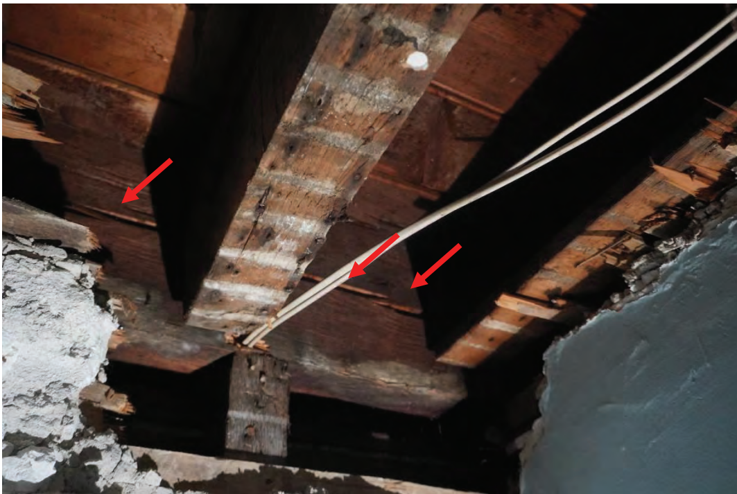
Photo #92: Interior girder running north to south is splitting along the mortise and tenon joint connections (Probe #4).
