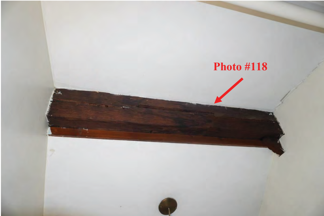
Photo #117: Roof support beam observed to be coming apart.
