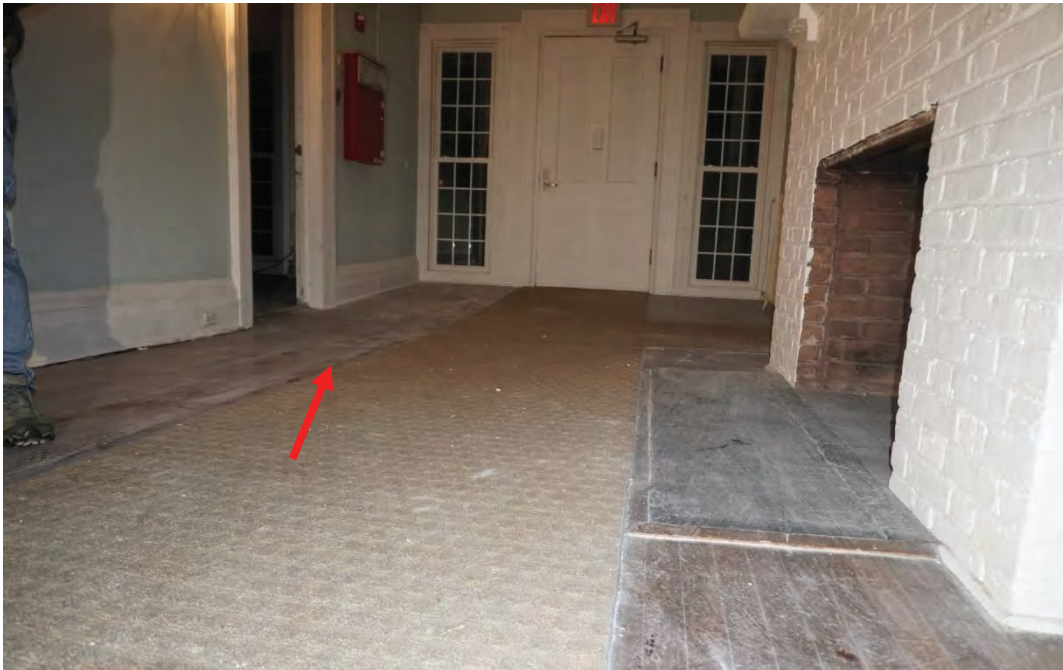
Photo #86: Large floor depression adjacent to load bearing wall 1 st floor. This area is directly above girder that is failing in the boiler area and being propped up with temporary columns. Staircase to go up to the second floor was originally located somewhere in this room.
