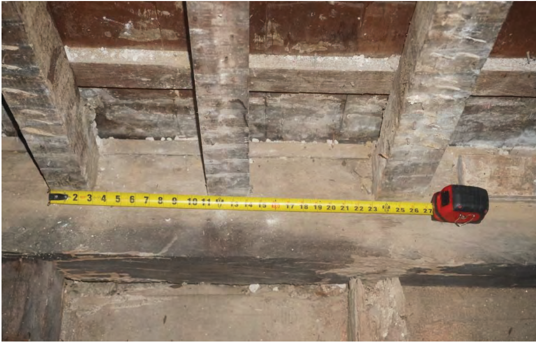
Photo #79: Vertical exterior framing members spaced at approximately 10 to 11 inches apart along west façade sitting on sill beam (Probe #1).
