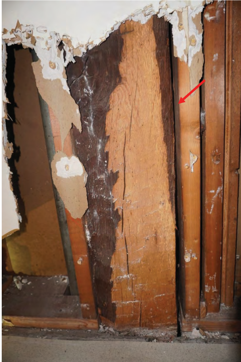
Photo #111: Post in attic space has moved out of place. Mortise and tenon joint that was connecting post to girder below has failed allowing member to rotate (Probe #10).
