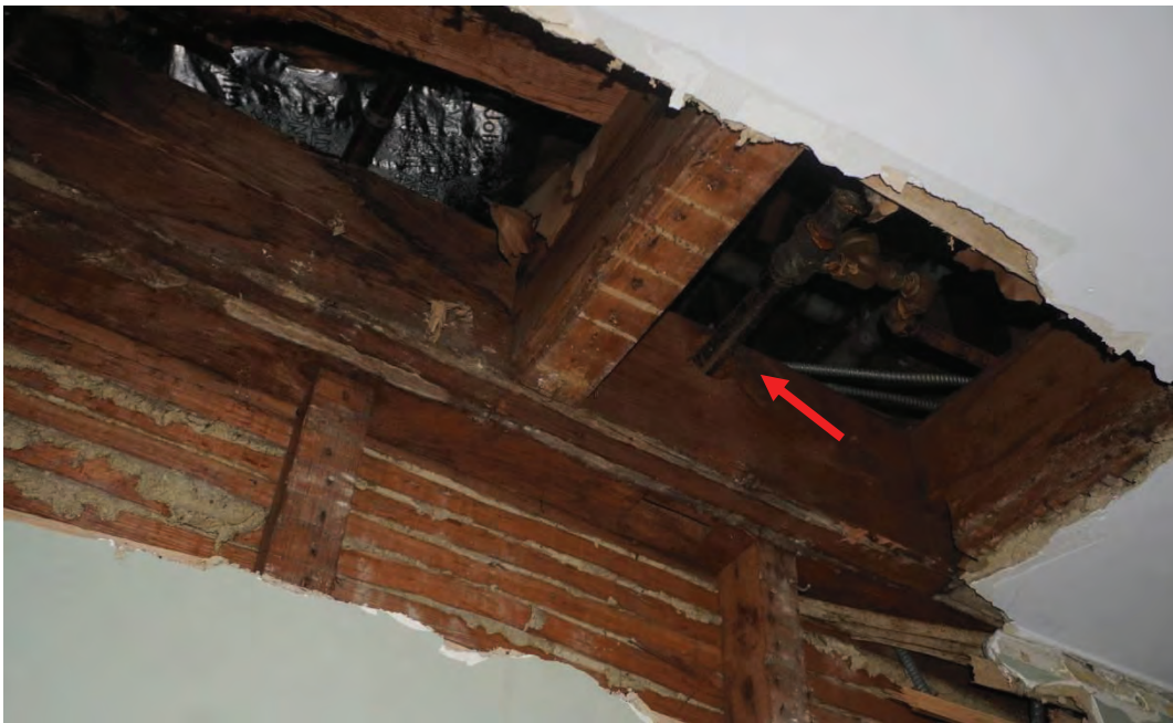
Photo #100: Floor joists supporting attic above observed at second floor level are oriented east to west. Large hole drilled through girder for pipe penetration (Probe #7).
