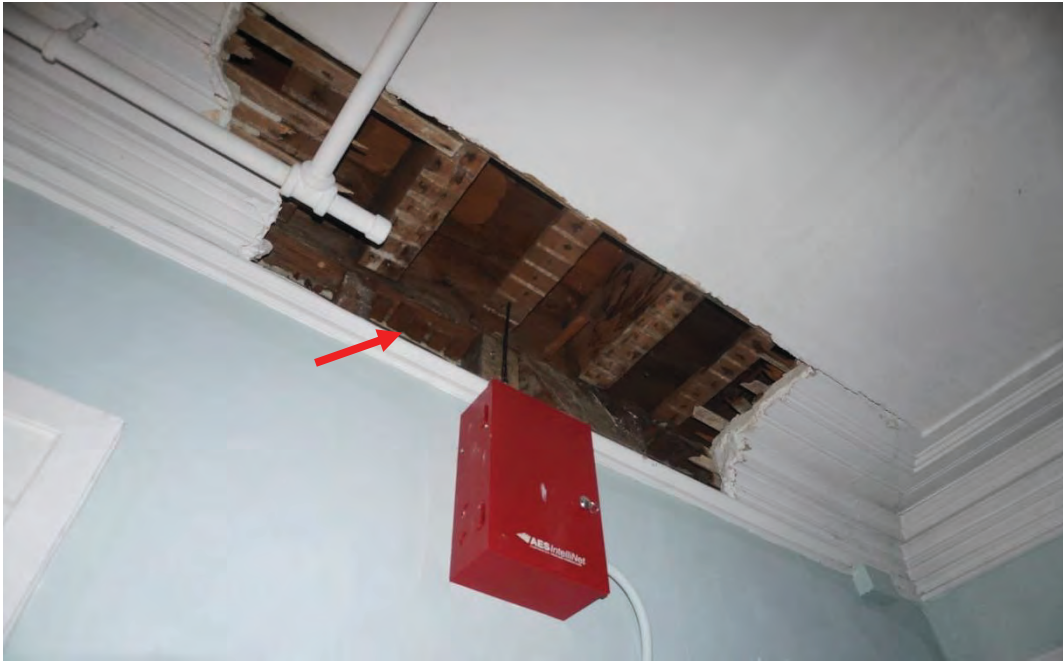
Photo #95: Interior girder that is showing signs of deflection. Girder is directly above girder that is failing in the boiler room area and is being propped up with temporary columns (Probe #5).
