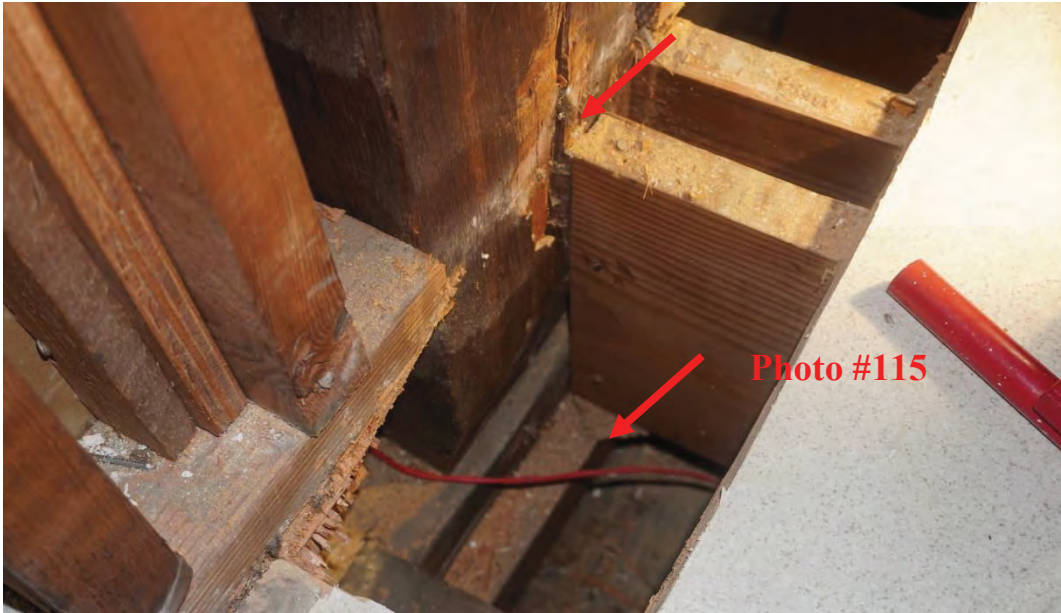
Photo #115: Vertical crack that has opened more towards the bottom observed, attic post. Unclear why this has occurred. Further investigation required. New wood joists have been installed going east to west bearing on wood ledge that has been nailed into girder. It is unclear why this was done. Further investigation required (Probe #12).
