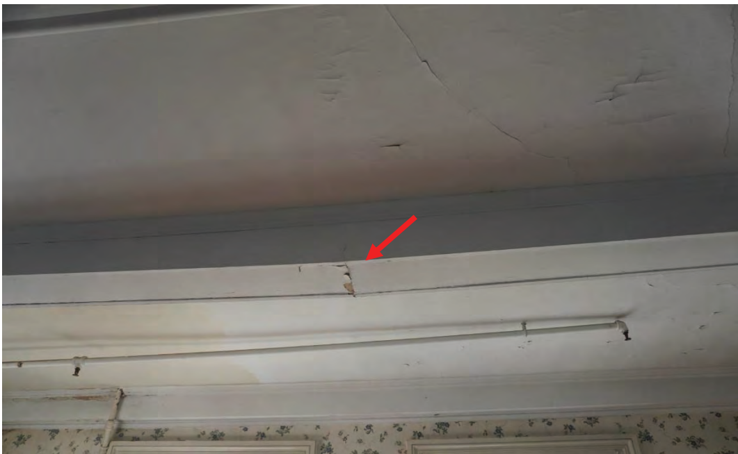
Photo #84: Soffit was opened up to further investigate crack. When soffit at this location was opened up it was empty inside and was just apparently there for aesthetic purposes (Probe #3).
