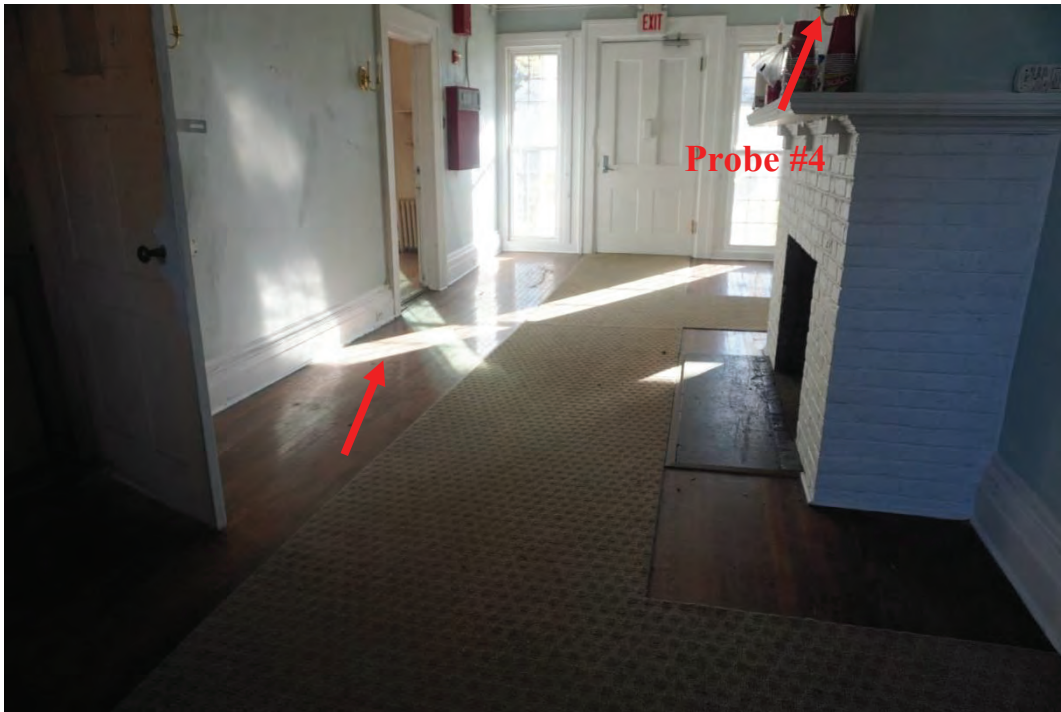
Photo #87: Large floor depression adjacent to load bearing wall 1 st floor. This area is directly above girder that is failing in the boiler area and being propped up with temporary columns. Staircase to go up to the second floor was originally located somewhere in this room.
