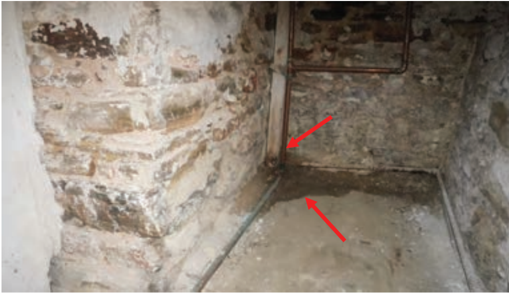
Photo #42: Water infiltration at base of inner, original foundation wall. Water is rotting base of wood support post. Crawlspace that spans the front side of the home is located on the other side of this wall.
