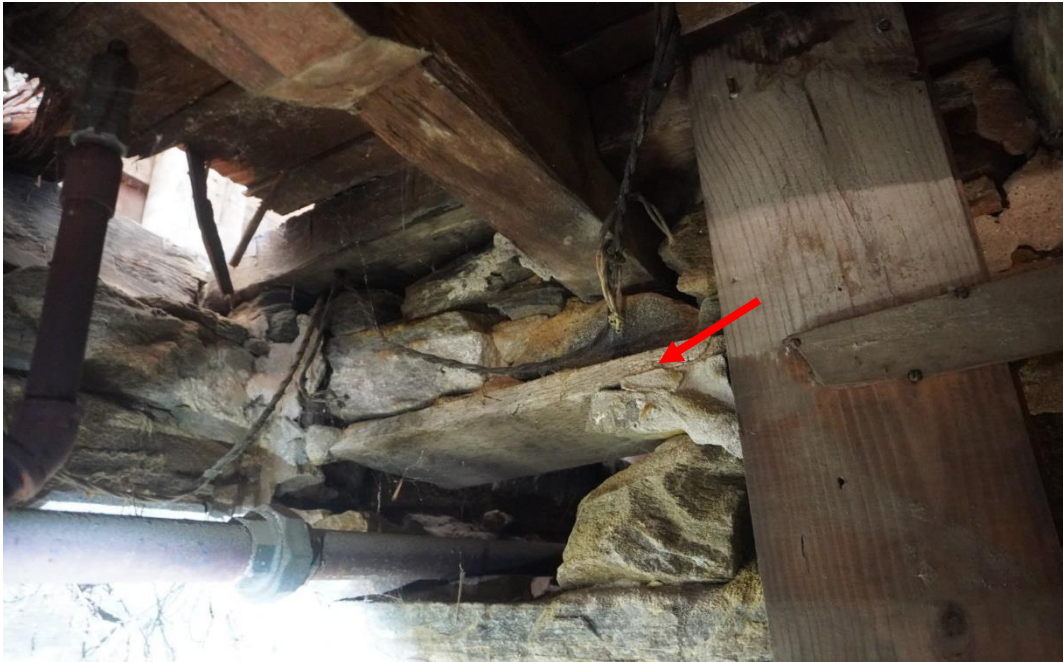
Photo #65: Joist with inadequate support resting on foundation wall that is deteriorated and that has been damaged to make a pipe penetration into crawlspace.
