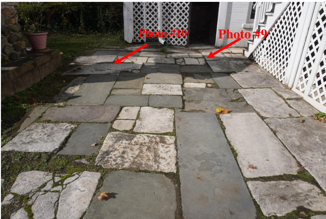
Photo #8: Stone slabs have settled/ heaved creating multiple trip hazards, stone patio rear yard.
