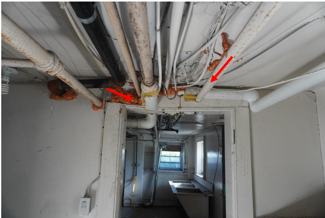
Photo #66: Multiple penetrations have been made through a door header that is observed to be failing. There is a wall on the first-floor level directly above this header.
