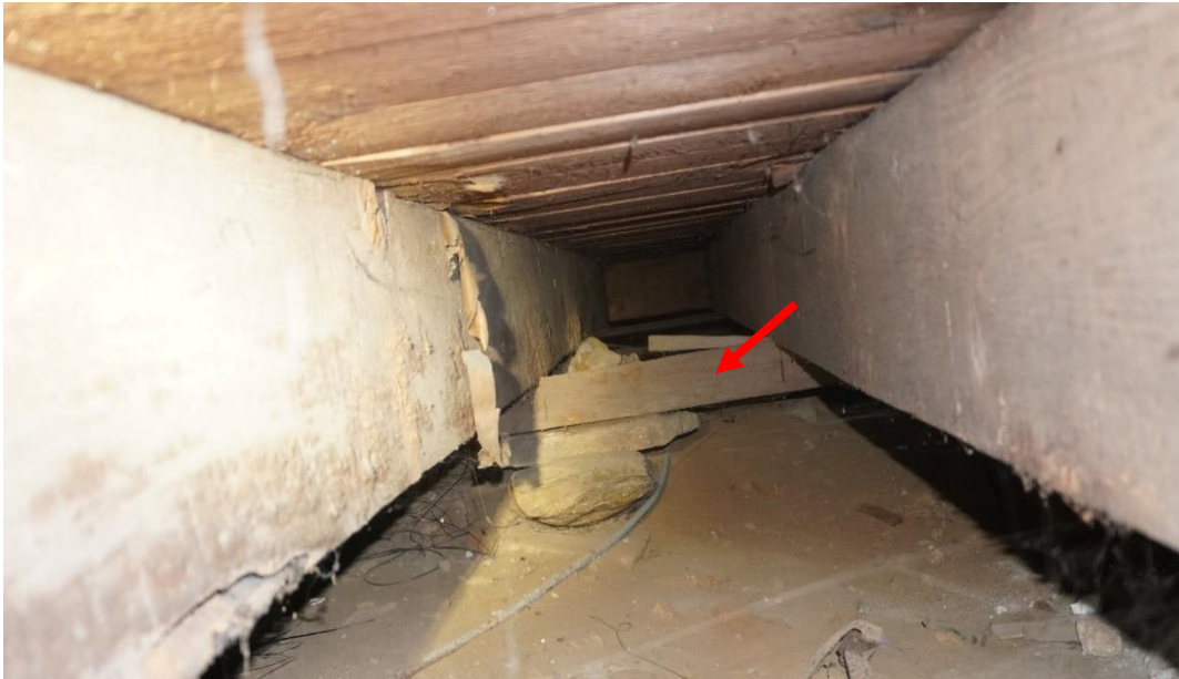
Photo #75: Wood joists spanning crawl space are being inadequately supported at midspans by wood members that are balanced above unstable pieces of stone (Probe #1).
