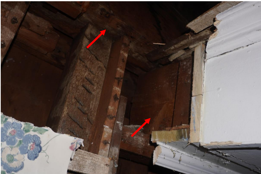
Photo #82: Ceiling soffit contains a support beam that runs east to west below the spandrel beam. Beam running east to west supports joists above at midspan. This is an atypical configuration that was most likely a modification and not part of the original timber framing design (Probe #2).
