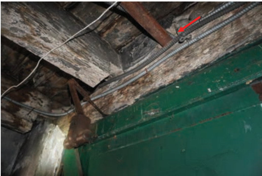
Photo #49: Pipe penetration drilled through door header leading out to rear yard.
