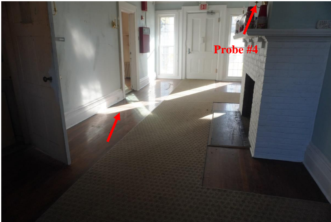
Photo #87: Large floor depression adjacent to load bearing wall 1 st floor. This area is directly above girder that is failing in the boiler area and being propped up with temporary columns. Staircase to go up to the second floor was originally located somewhere in this room.
