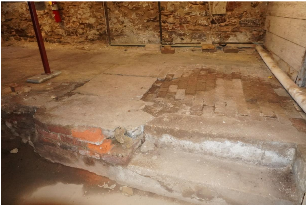
Photo #45: Cellar floor observed to be composed of bricks with a cement stucco layer that is deteriorating.
