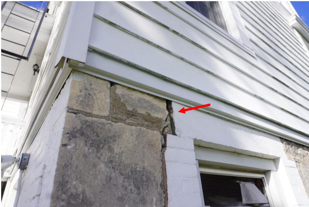
Photo #24: Vertical crack ground level stonework east façade, southeast corner of structure at addition.
