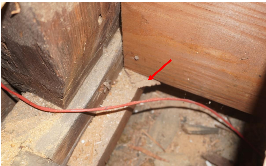
Photo #116: New wood joists have been installed going east to west bearing on wood ledge that has been nailed into girder. It is unclear why this was done. Further investigation required (Probe #12).
