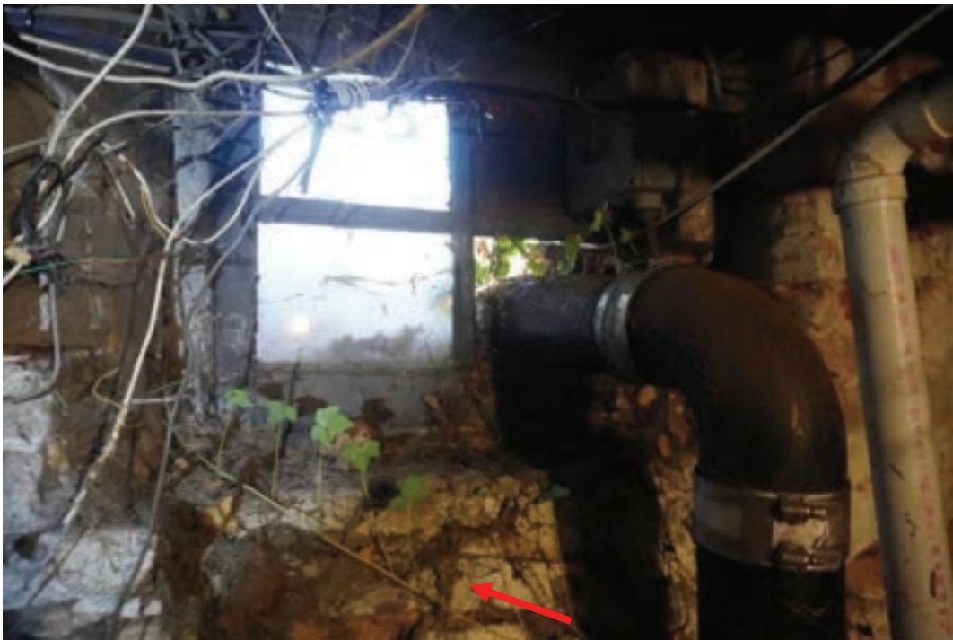
Photo #56: Dirt and soil infiltrating around window in cellar at west foundation wall.
