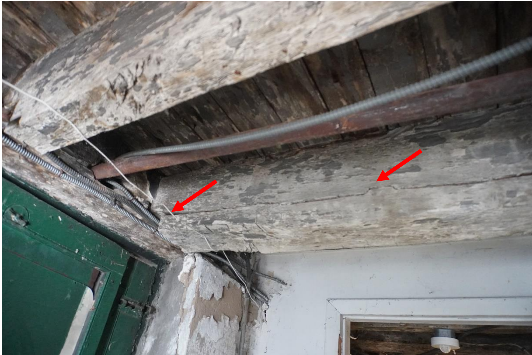
Photo #50: Horizontal crack from shear stress resonating down entire member from notch at end of beam.
