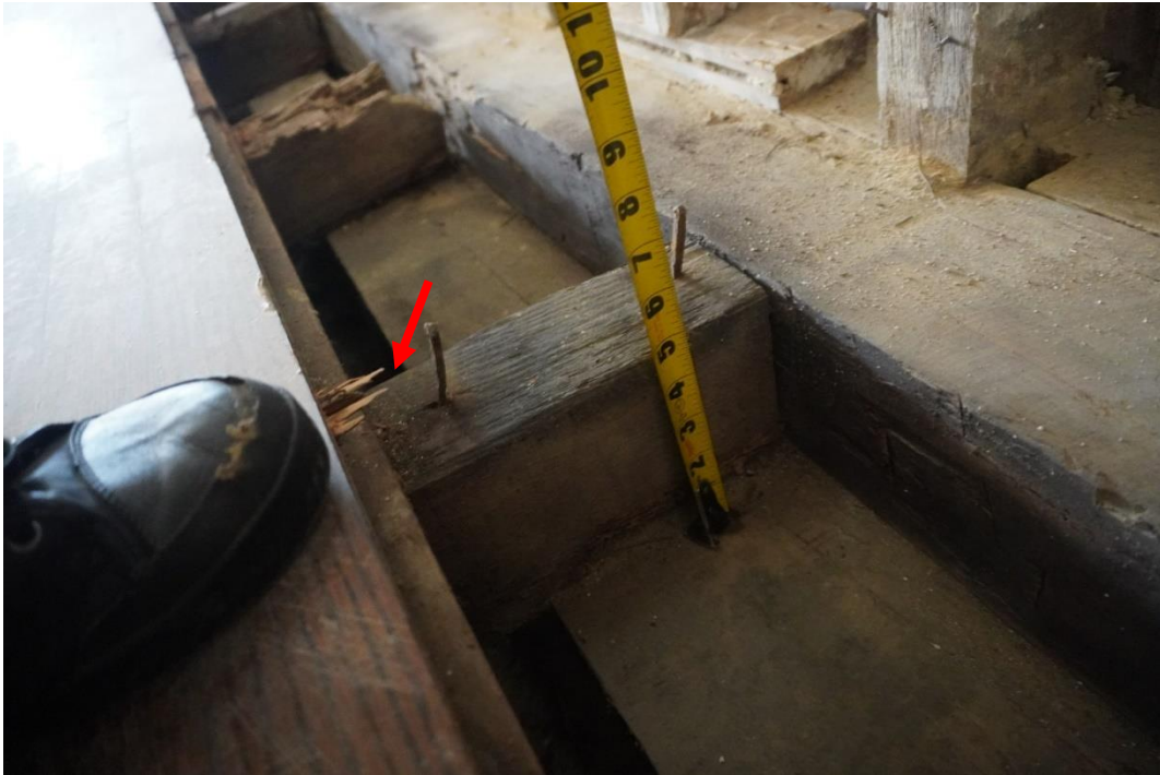
Photo #69: Original floorboards above crawlspace have been removed. New wood flooring directly attached to joists. Crawl space joists sitting on an improperly supported sill plate.
