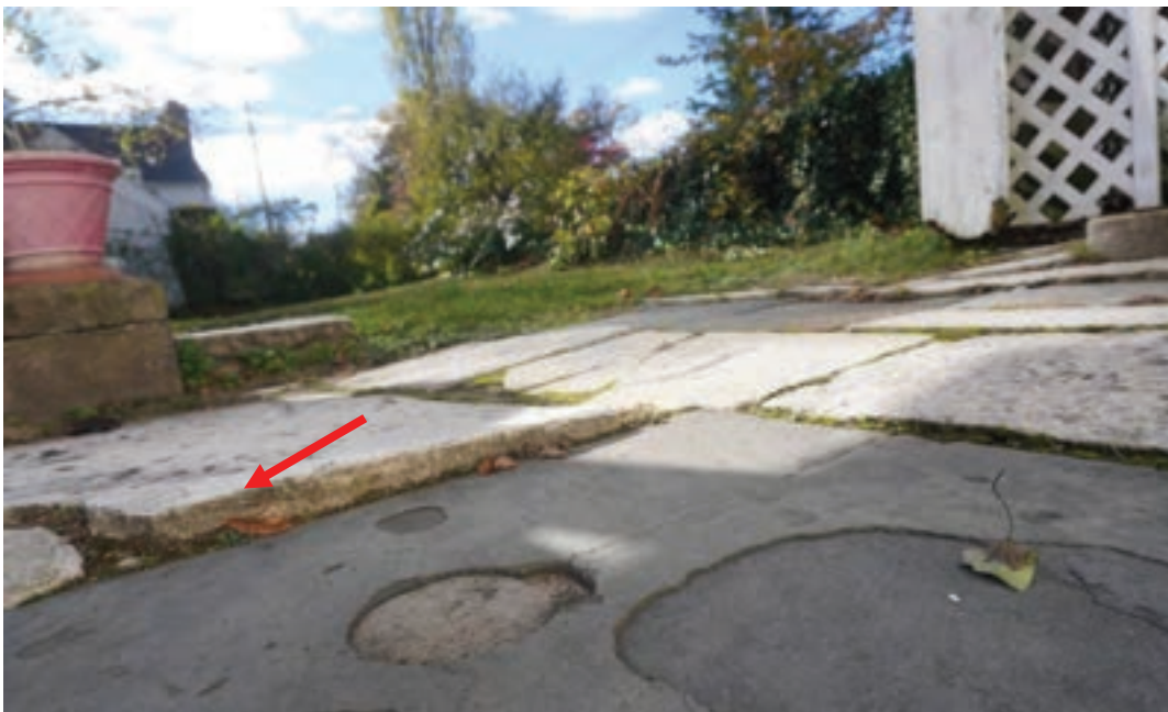
Photo #10: Stone slabs have settled/ heaved creating multiple trip hazards, stone patio rear yard.
