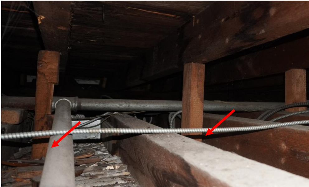
Photo #109: View facing northeast in roof void between 2 nd floor ceiling joists and roof joists in the addition. Roof joists do not align with ceiling joists and are being supported at midspan with blocking that is resting right onto plaster ceiling (Probe #9).
