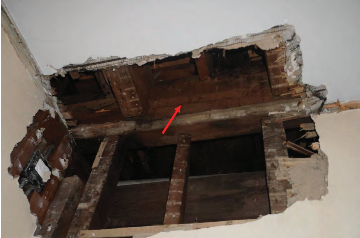
Photo #103: New joists running east to west have been installed at higher level than original joists and are resting on a 2x4 wood ledges that have been nailed to girder to support attic floor above. It is unclear why these joists were installed. Most likely to add additional space for piping below showers and toilets in attic. Further investigation required. Original joists left in place and still supporting ceiling below (Probe #8).
