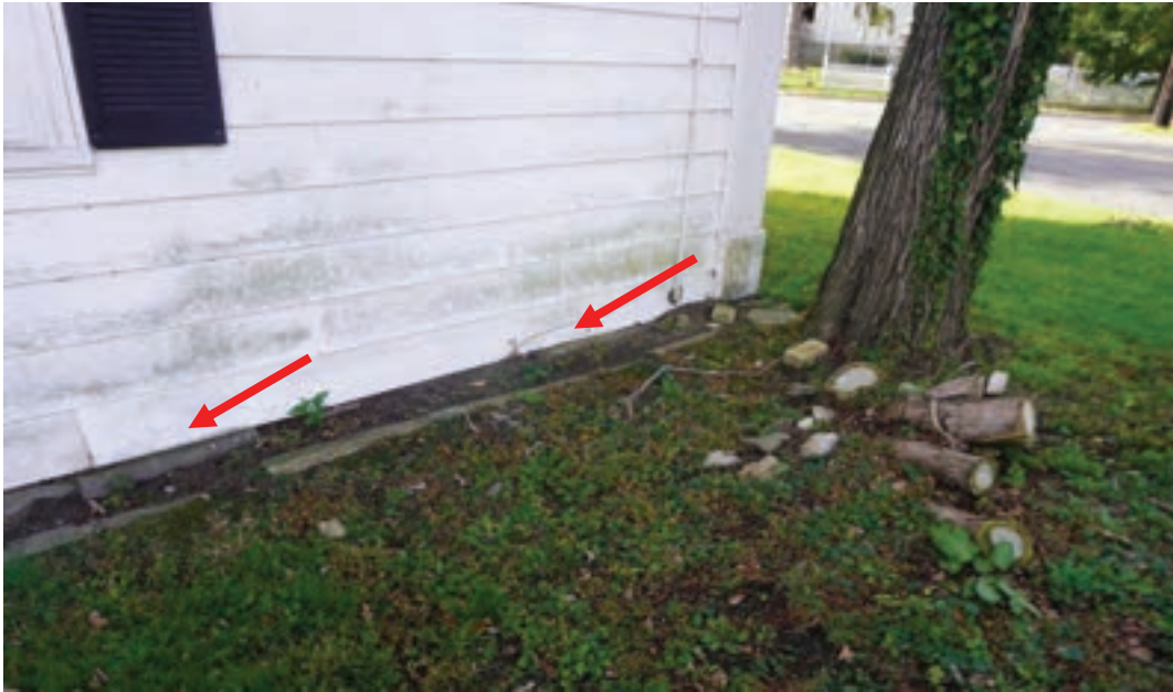
Photo #13: Foundation along front façade of original structure is low and at same level as grading. Water can infiltrate above foundation wall and rot out wood sill beam that runs along top of foundation. once again condition can easily be regraded if infiltration is occurring
