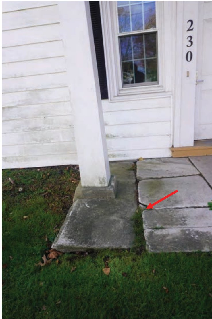
Photo #19: Base of column support for front portico showing signs of differential settlement.
