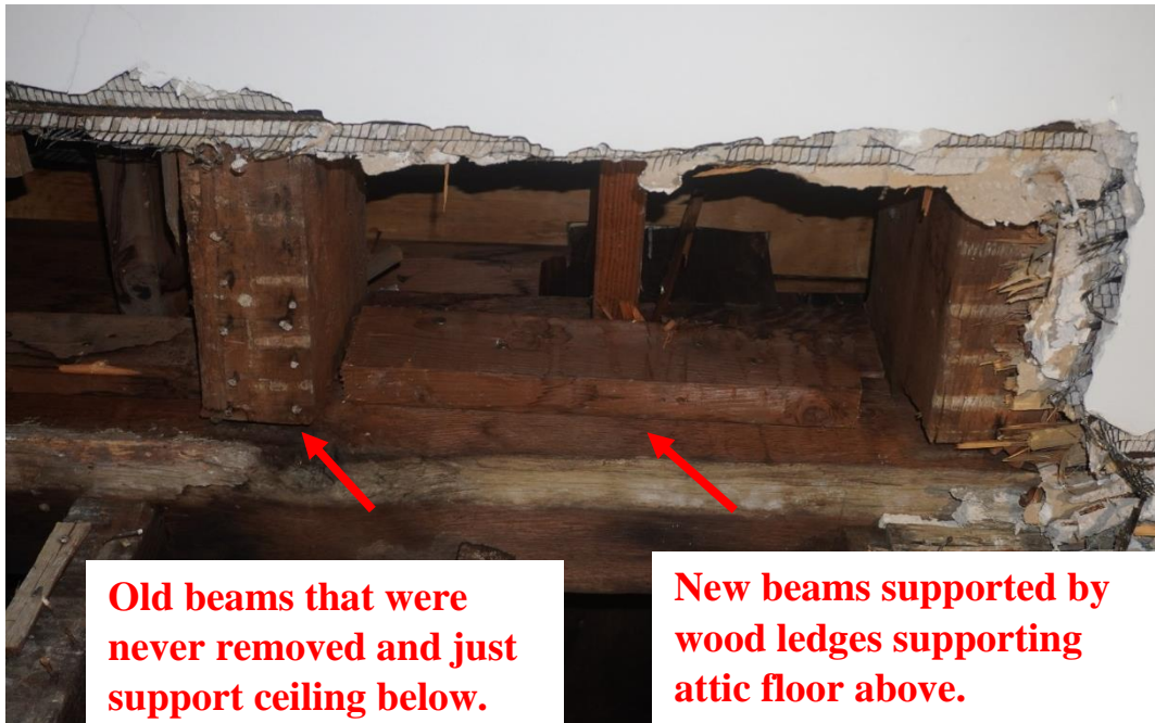
Photo #105: New joists running east to west have been installed at higher level than original joists and are resting on a wood ledge 2x4s that have been nailed to girder to support attic floor above (Probe #8).
