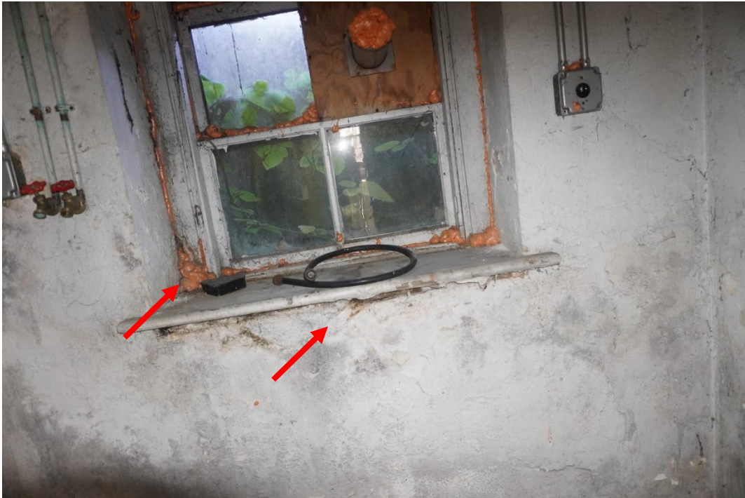
Photo #40: Water infiltration around cellar window, north façade of home at window well.
