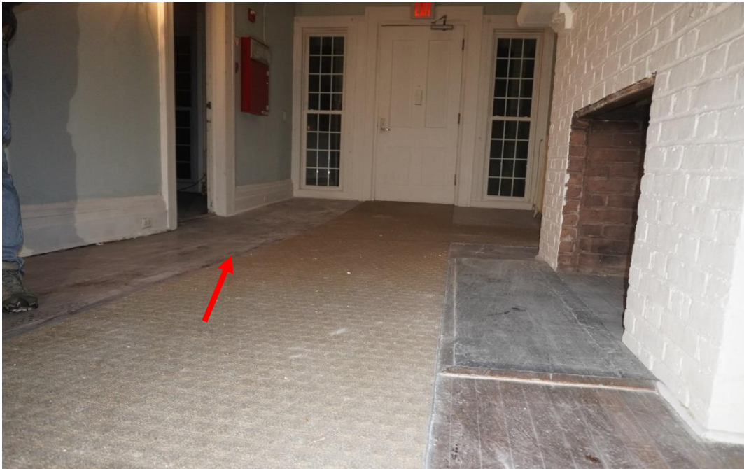
Photo #86: Large floor depression adjacent to load bearing wall 1 st floor. This area is directly above girder that is failing in the boiler area and being propped up with temporary columns. Staircase to go up to the second floor was originally located somewhere in this room.
