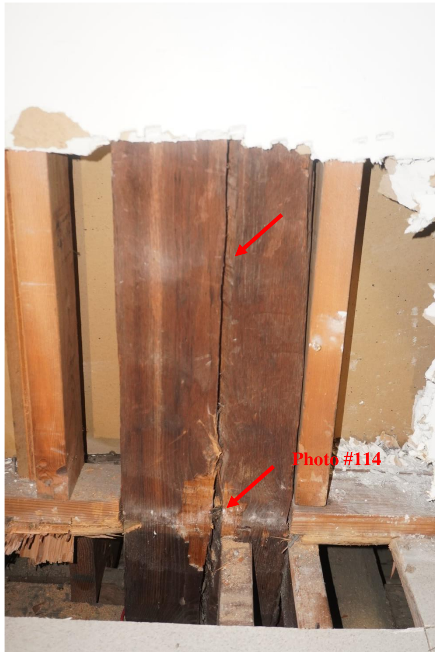
Photo #114: Vertical crack that has opened more towards the bottom observed, attic post Unclear why this has occurred. Further investigation required (Probe #12).
