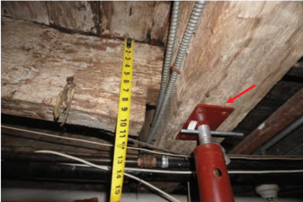
Photo #59: Temporary support column being used to hold failing 9-1/2"x9-1/4" girder in boiler room. Column not mechanically attached to girder above and does not have a proper footing. not an uncommon "temporary" repair when certain loads (piano?) are added above or floor feels bouncy. As noted, can be made permanent with designed footing and connection.
