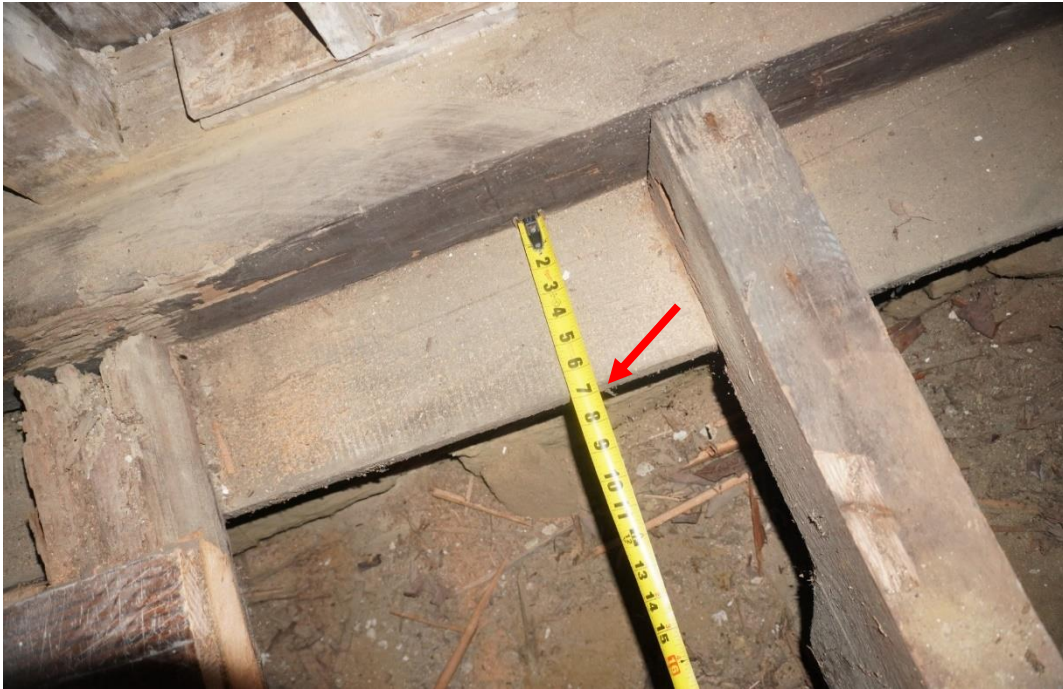
Photo #71: Crawl space joists sit on a 7-inch sill plate that is only bearing 3 inches onto deteriorating foundation wall below. Sill plate has a four-inch unsupported overhang (Probe #1).
