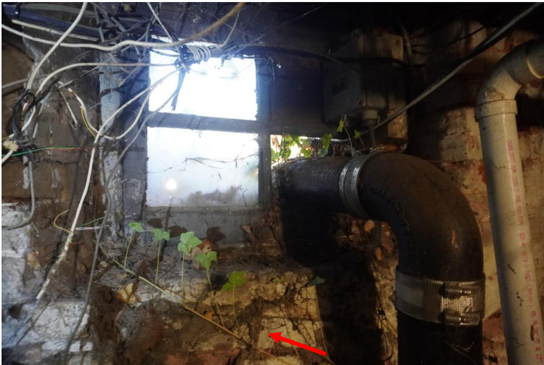
Photo #56: Dirt and soil infiltrating around window in cellar at west foundation wall.
