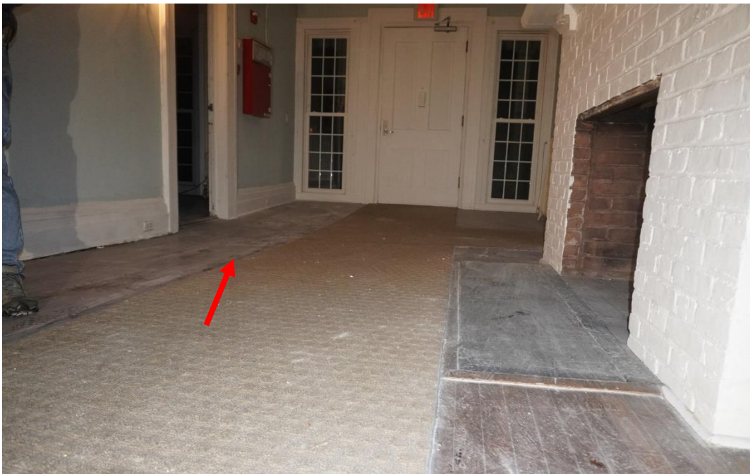
Photo #86: Large floor depression adjacent to load bearing wall 1 st floor. This area is directly above girder that is failing in the boiler area and being propped up with temporary columns. Staircase to go up to the second floor was originally located somewhere in this room.
