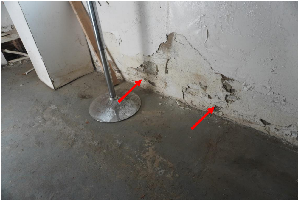
Photo #37: Water intrusion foundation, south wall of home at extension.
