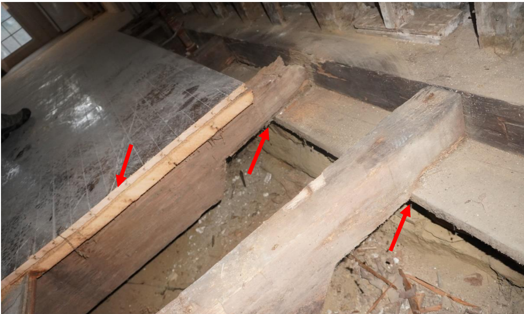
Photo #70: Original floorboards above crawlspace have been removed. New wood flooring directly attached to joists. Crawl space joists sitting on an improperly supported sill plate (Probe#1).
