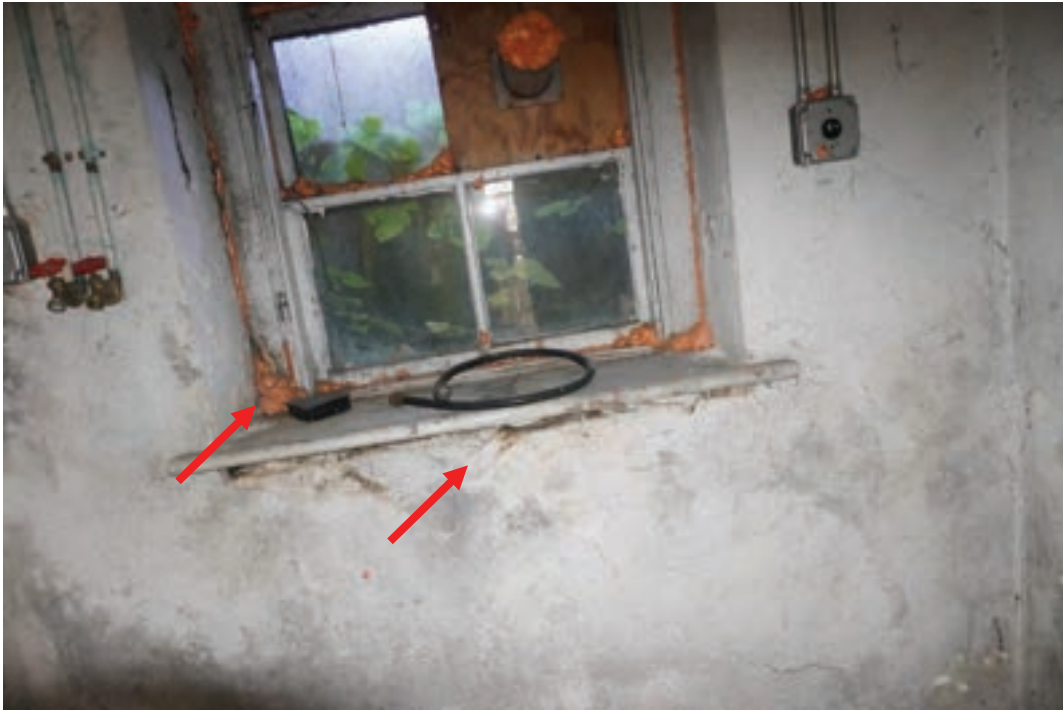
Photo #40: Water infiltration around cellar window, north façade of home at window well. maintain exterior; clear window well of organics
