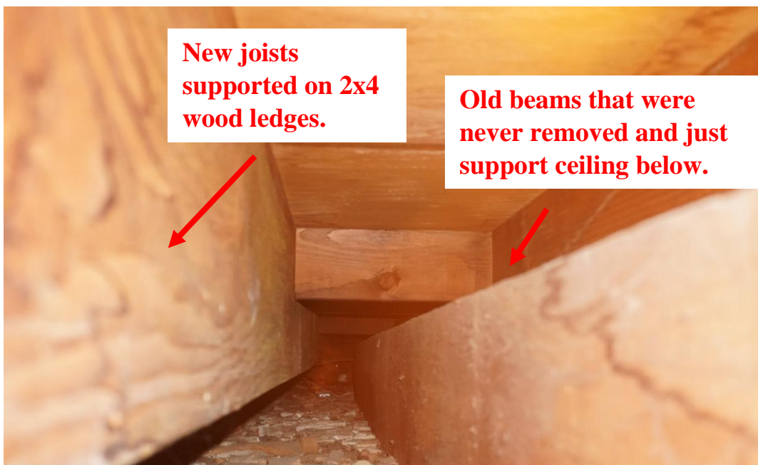
Photo #106: New joists running east to west have been installed at higher level than original joists and are resting on a wood ledge 2x4s that have been nailed to girder to support attic floor above (Probe #8). (Probe #8)
