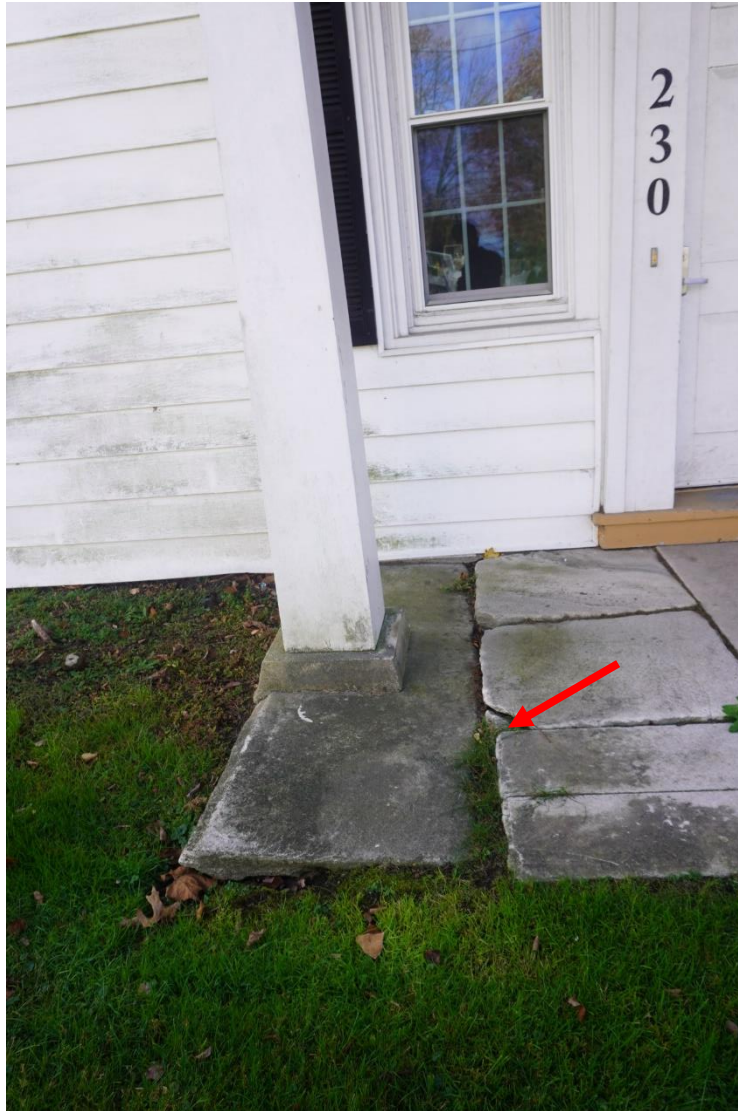
Photo #19: Base of column support for front portico showing signs of differential settlement.
