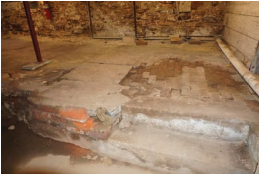
Photo #45: Cellar floor observed to be composed of bricks with a cement stucco layer that is deteriorating.
