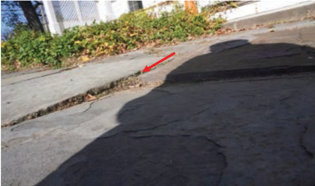
Photo #7: Stone slabs have settled/heaved creating multiple trip hazards, stone walkway rear yard.
