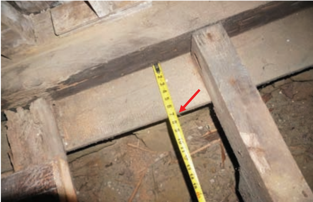
Photo #71: Crawl space joists sit on a 7-inch sill plate that is only bearing 3 inches onto deteriorating foundation wall below. Sill plate has a four-inch unsupported overhang (Probe #1).
