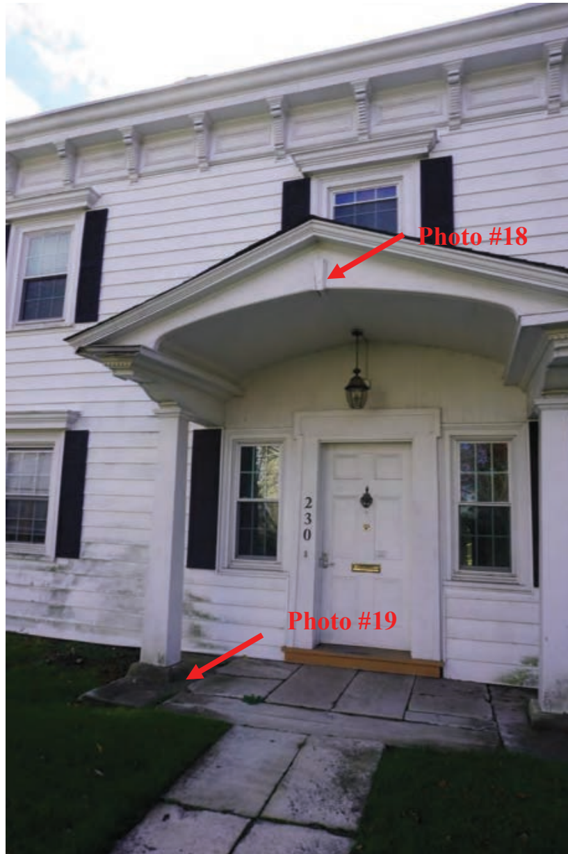
Photo #17: Base of column support for front portico showing signs of differential settlement. Vertical crack running down middle of front portico.
