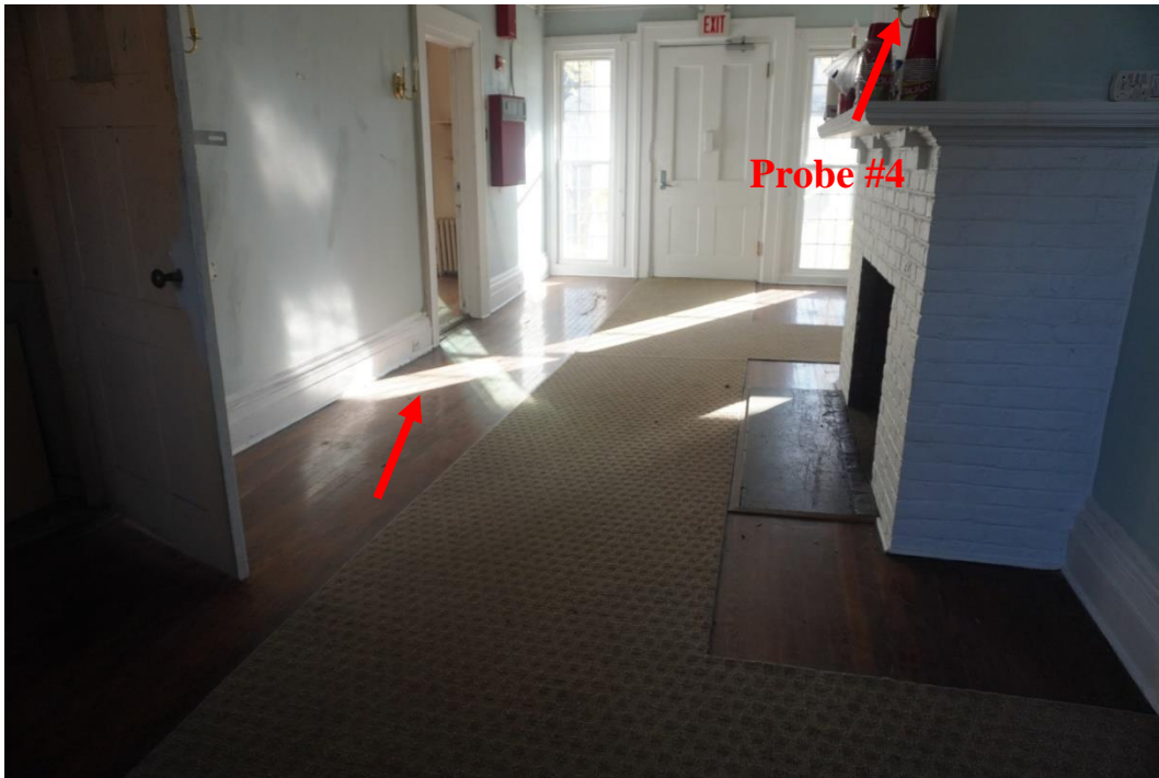
Photo #87: Large floor depression adjacent to load bearing wall 1 st floor. This area is directly above girder that is failing in the boiler area and being propped up with temporary columns. Staircase to go up to the second floor was originally located somewhere in this room.
