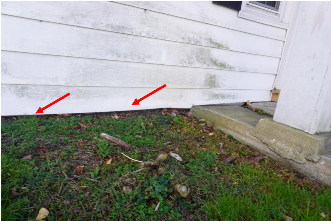
Photo #16: Foundation along front façade of original structure is low and at same level as grading. Water can infiltrate above foundation wall and rot out wood sill beam that runs along top of foundation.
