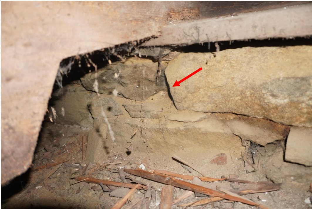
Photo #68: Thin sill plate, joists spanning crawlspace are sitting on, is being supported by a rubble stone foundation wall that is coming apart (Probe #1).
