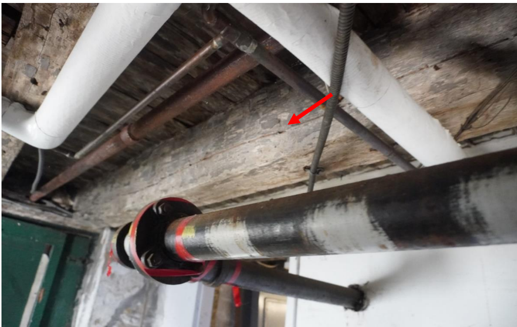
Photo #51: Horizontal crack from shear stress resonating down entire member from notch at end of beam.
