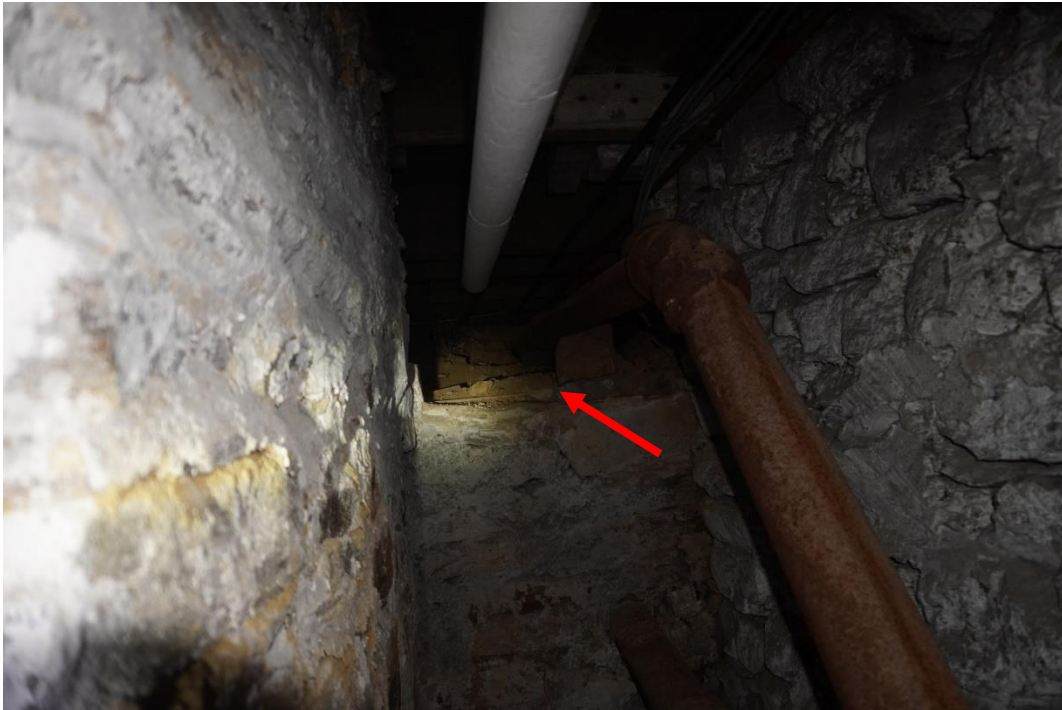
Photo #55: Piping was run into crawlspace through what potentially was an old window (second location) in original foundation wall.
