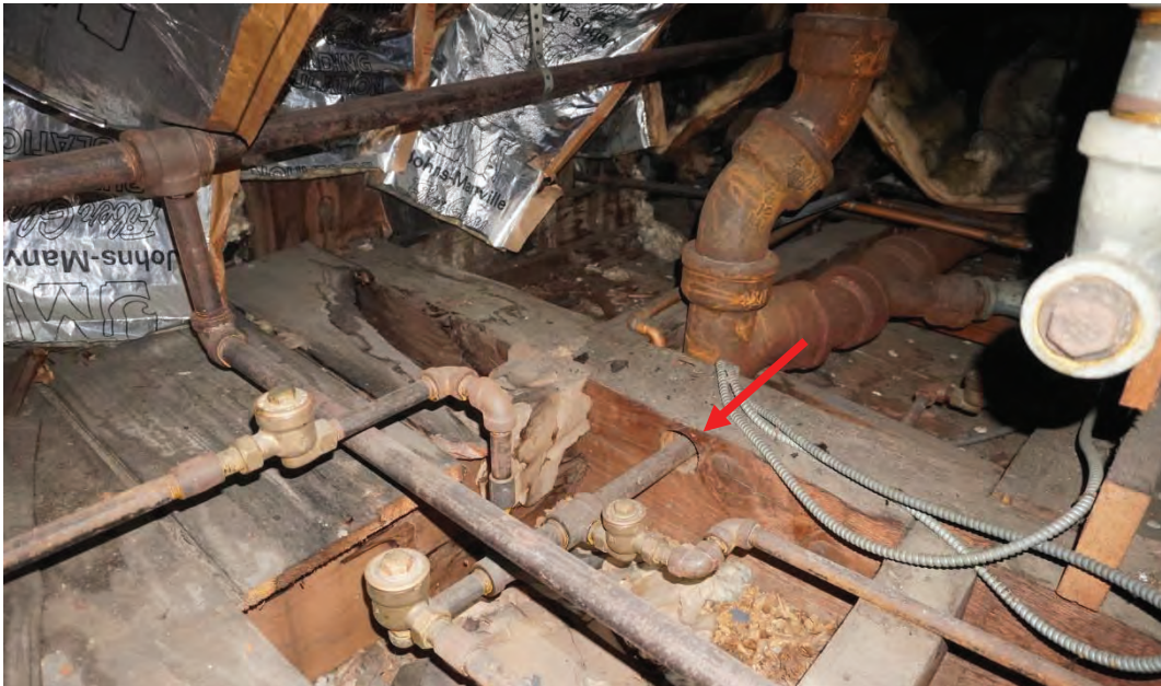
Photo #110: Pipe penetration drilled through girder drilled above its neutral axis. Observed in unfinished attic area, north side of original structure.
