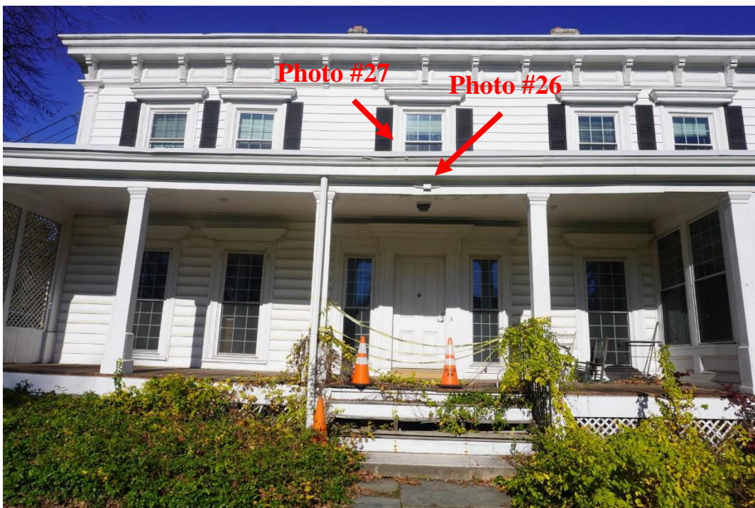
Photo #25: Rear porch roof deflecting over stairs causing water to pool and leaf build up.
