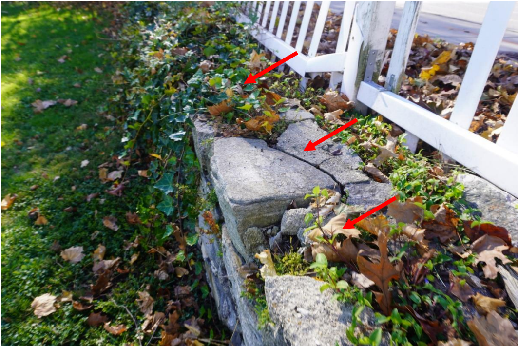
Photo #11: Retaining wall that runs between rear yard and adjacent sidewalk deteriorating throughout. Broken stones and joints between stones have filled with dirt/ organic growths.
