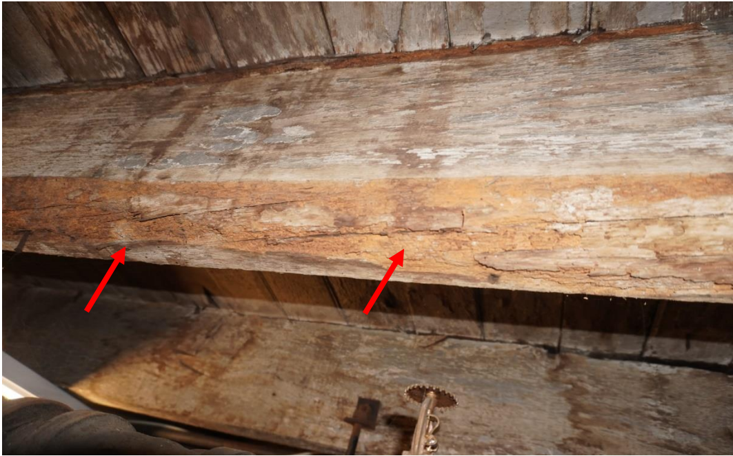
Photo #61: Wood joist observed to have a large extent of termite damage.
