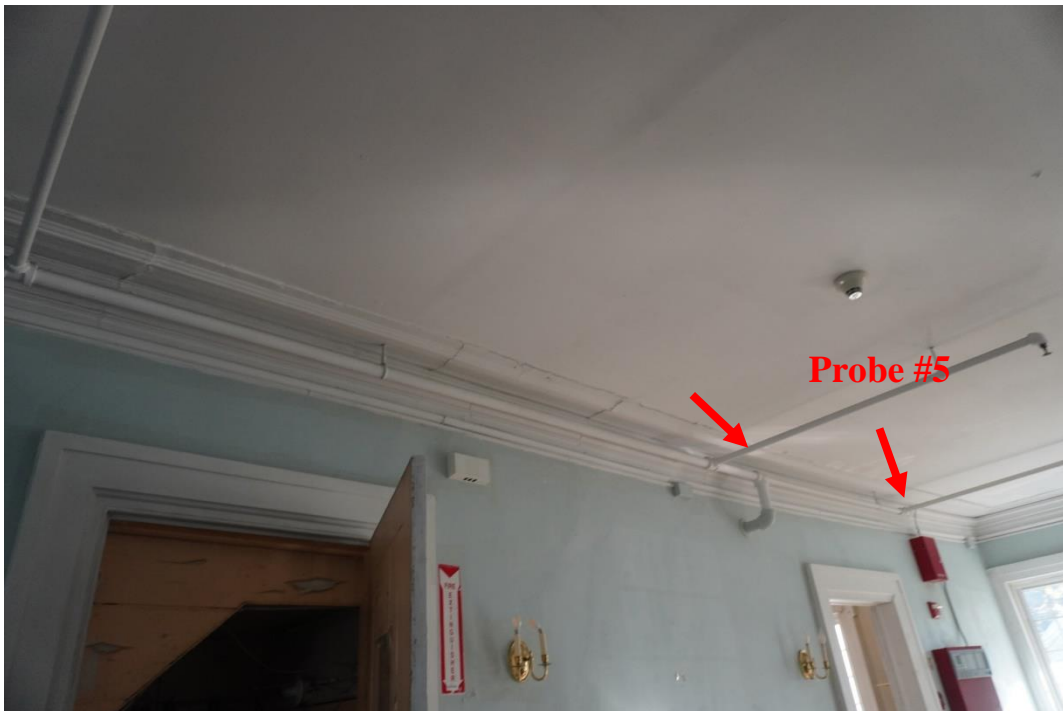
Photo #94: Wall containing girder beam showing signs of deflection. This girder is directly above girder that is failing in the boiler room area and is being propped up with temporary columns (Probe #5).
