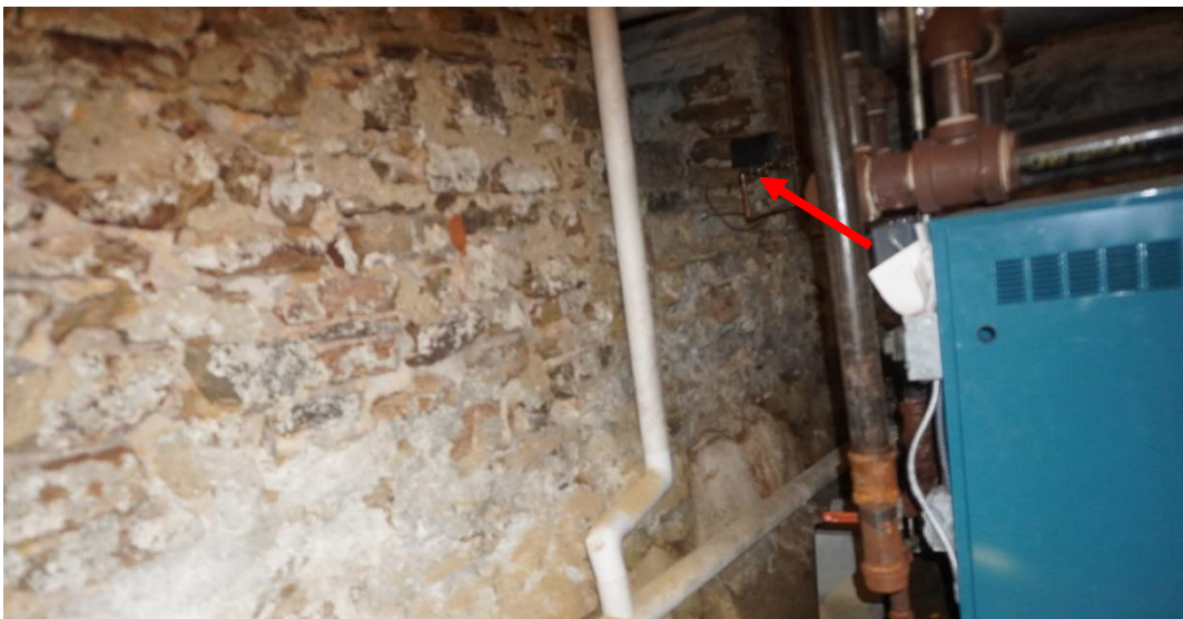
Photo #54: Piping was run into crawlspace through what potentially was an old window in original foundation wall.
