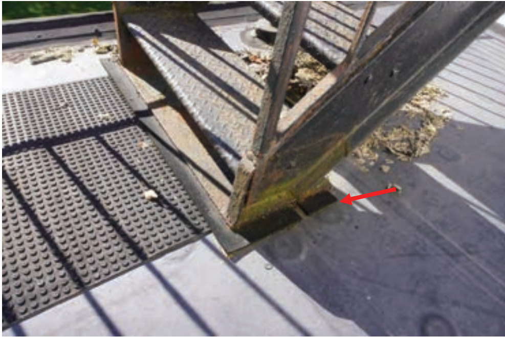
Photo #30: Exterior metal stair egress just sitting on roofing membrane and not attached to structure.
