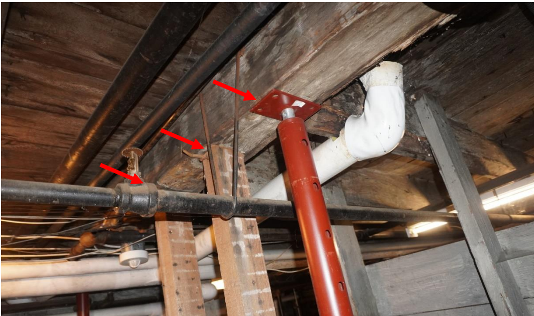
Photo #64: Temporary support columns being used to hold failing 6-3/4"x10-1/2" girder in place west end of cellar. Columns are not mechanically attached to girder above and do not have proper footings.
