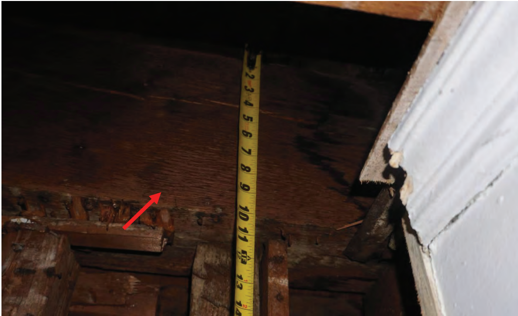
Photo #81: 10x7 Exterior spandrel beam running north to south 1 st floor ceiling level along west exterior wall. (Probe #2)
