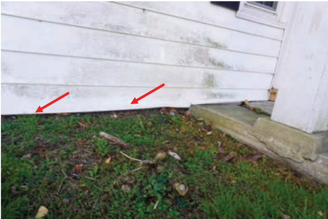
Photo #16: Foundation along front façade of original structure is low and at same level as grading. Water can infiltrate above foundation wall and rot out wood sill beam that runs along top of foundation.
