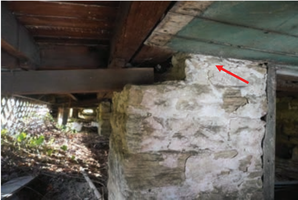
Photo #32: Rear porch sitting on stone pillars that are showing signs of deterioration. sacrificial lime coating can be redone and repointing undertaken as required.
