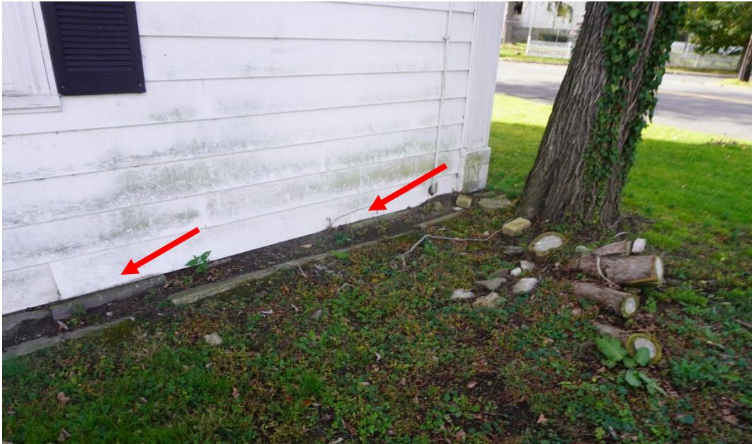
Photo #13: Foundation along front façade of original structure is low and at same level as grading. Water can infiltrate above foundation wall and rot out wood sill beam that runs along top of foundation.
