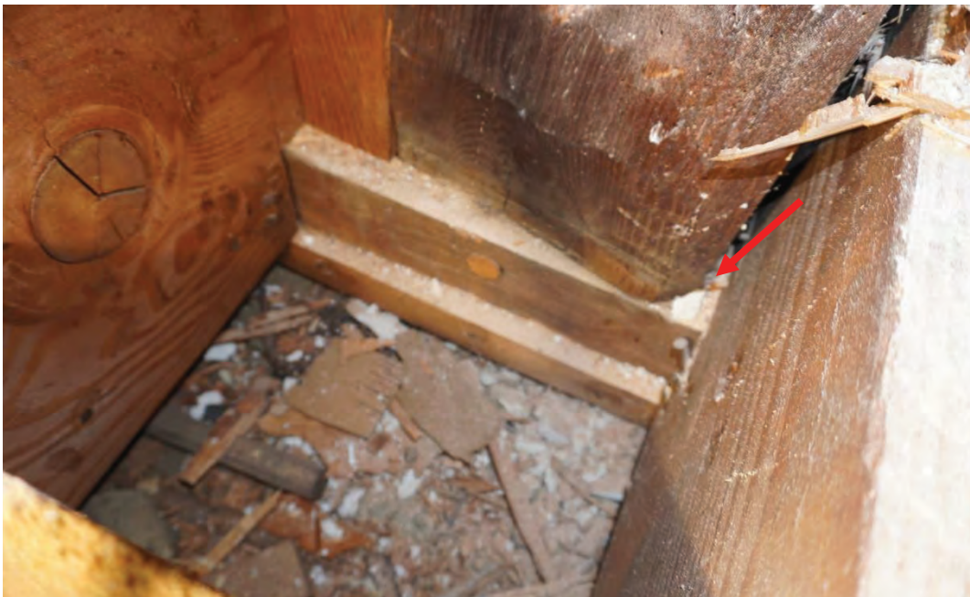
Photo #113: Post in attic space has moved out of place. Mortise and tenon joint that was connecting post to girder below has failed allowing member to rotate (Probe #11).
