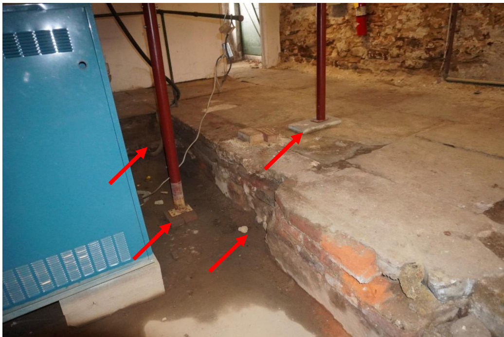
Photo #43: Water infiltration through foundation floor around perimeter of boiler pit. Concrete footings were never poured beneath temporary support columns that were added to prop up both failing girders in the cellar.
