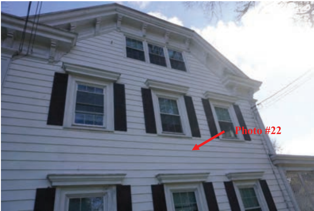
Photo #21: Bulge noticed between first and second floors, west façade of home. Cause unknown. Further investigation required.
