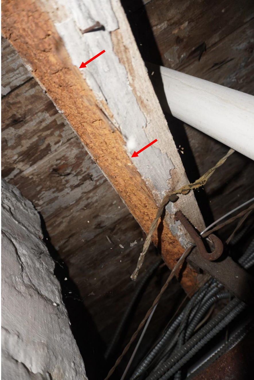
Photo #52: Wood joist observed to have a large extent of termite damage.
