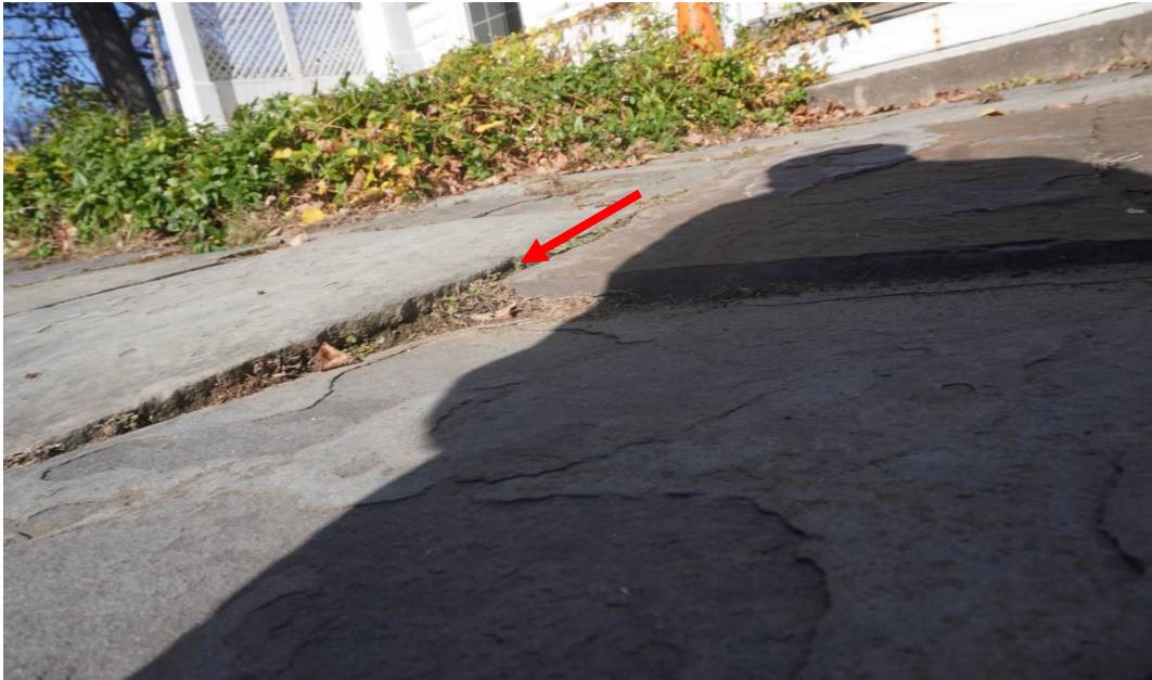
Photo #7: Stone slabs have settled/heaved creating multiple trip hazards, stone walkway rear yard.
