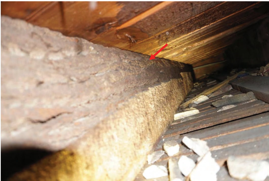
Photo #90: Ceiling joist that was never fully scored into a square framing member and still has bark exterior (Probe #4).
