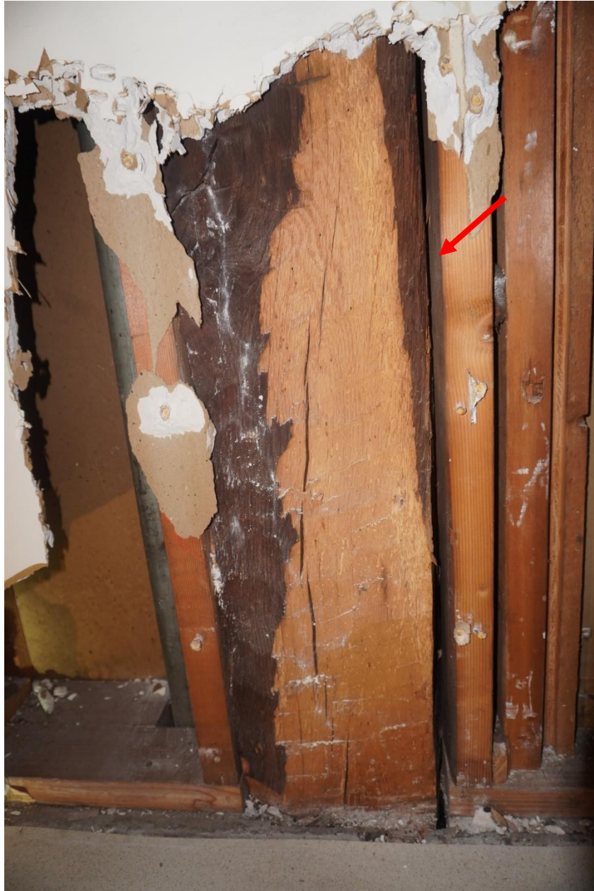
Photo #111: Post in attic space has moved out of place. Mortise and tenon joint that was connecting post to girder below has failed allowing member to rotate (Probe #10).
