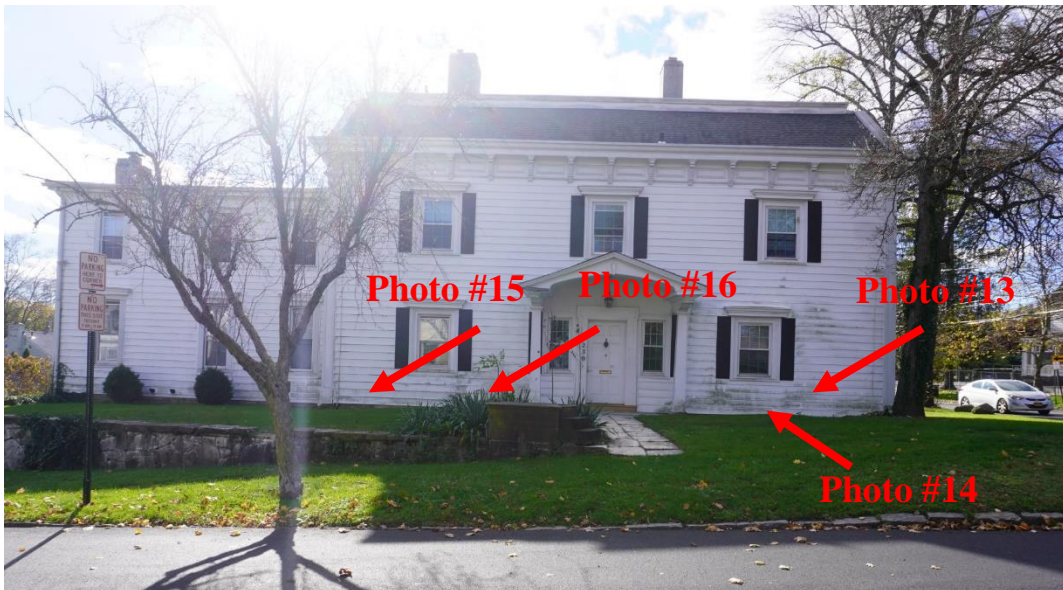
Photo #12: Foundation along front façade of original structure is low and at same level as grading. Water can infiltrate above foundation wall and rot out wood sill beam that runs along top of foundation.
