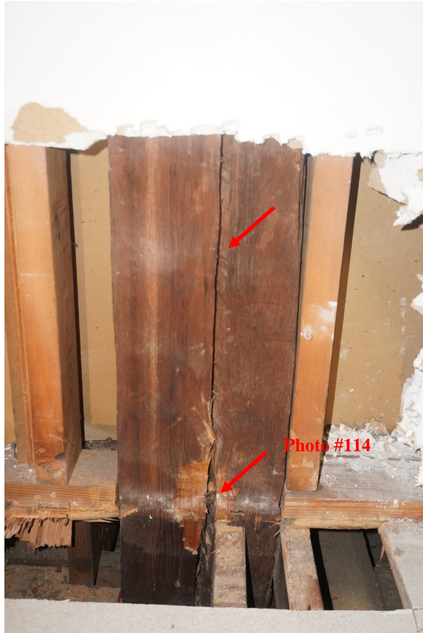
Photo #114: Vertical crack that has opened more towards the bottom observed, attic post Unclear why this has occurred. Further investigation required (Probe #12).
