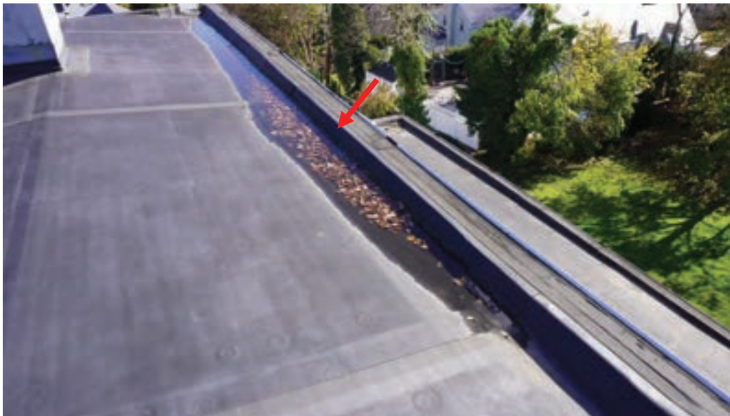
Photo #29: Roof structure has deflected causing water to pool. Roofing membrane observed to be fairly new.
