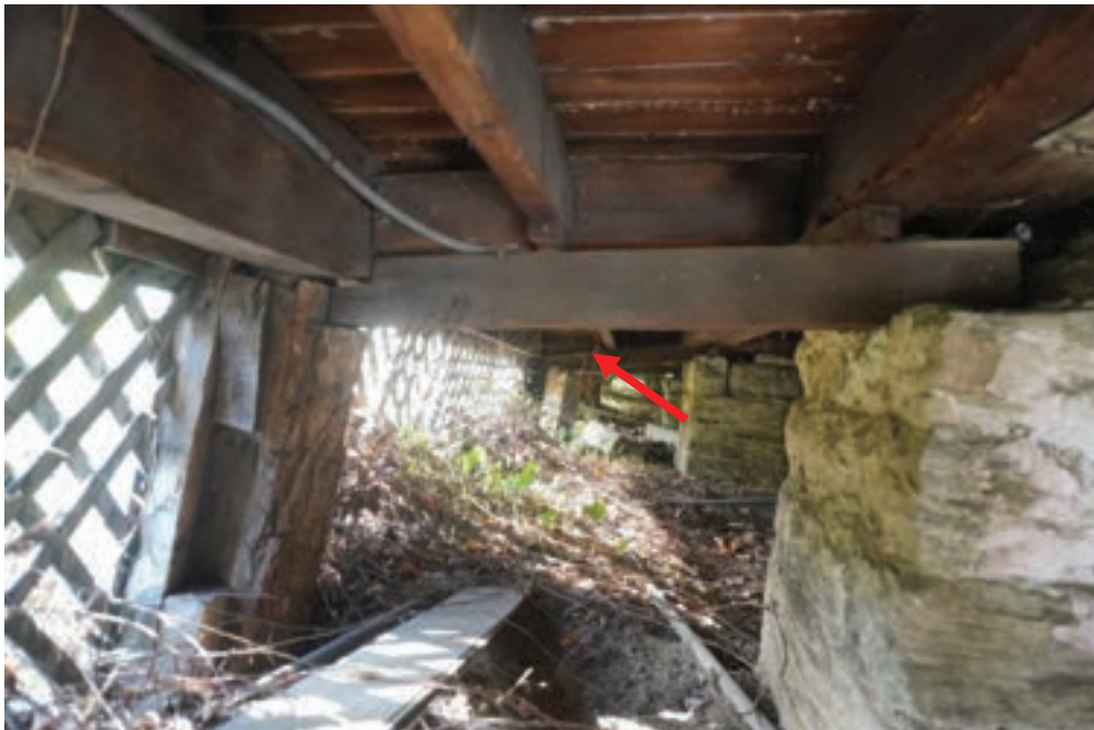
Photo #33: Rear porch was extended to be made wider at some unknown time in the past.
