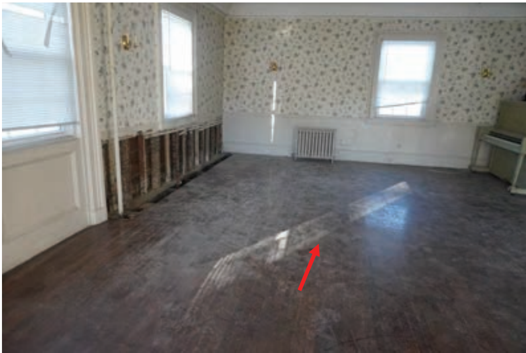
Photo #76: Location of west chimney that was relocated at some point in the past. Foundation still in place and can be observed in cellar below.
