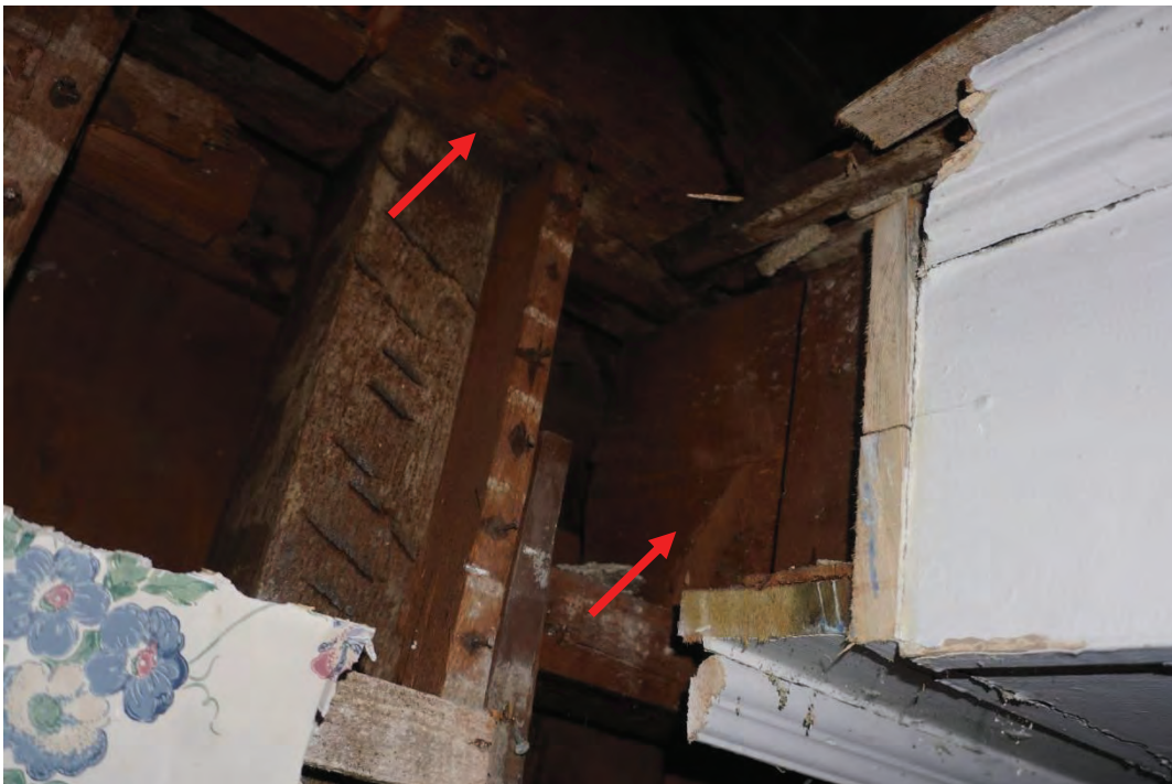
Photo #82: Ceiling soffit contains a support beam that runs east to west below the spandrel beam. Beam running east to west supports joists above at midspan. This is an atypical configuration that was most likely a modification and not part of the original timber framing design (Probe #2).
