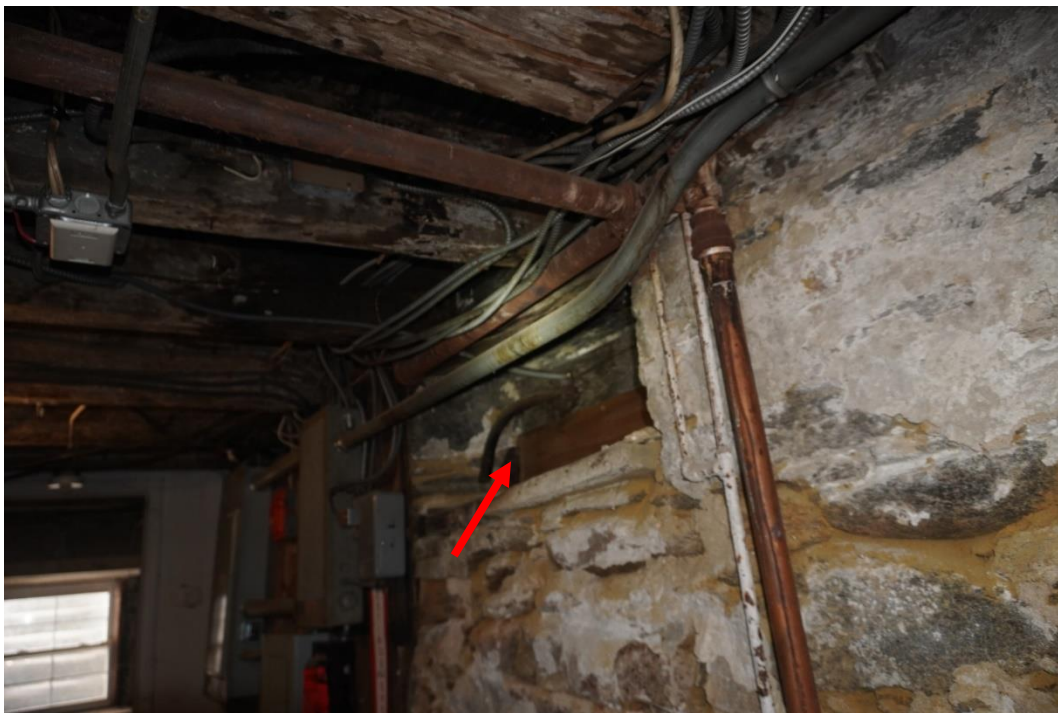
Photo #58: Cellar window at boiler room south foundation wall has been covered up when porch was added to the rear of the home.
