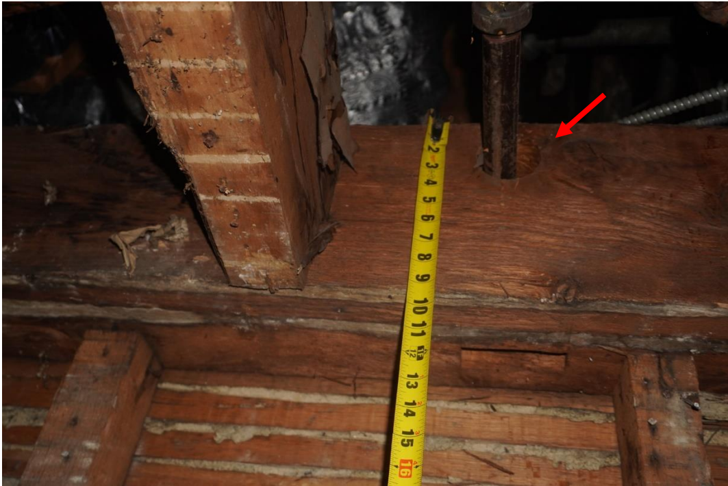
Photo #101: Floor joists supporting attic above observed at second floor level are oriented east to west. Large hold drilled through girder for pipe penetration (Probe #7).
