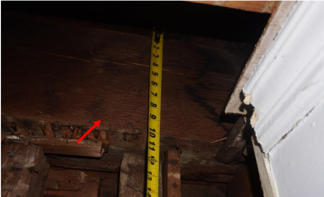
Photo #81: 10x7 Exterior spandrel beam running north to south 1 st floor ceiling level along west exterior wall. (Probe #2)
