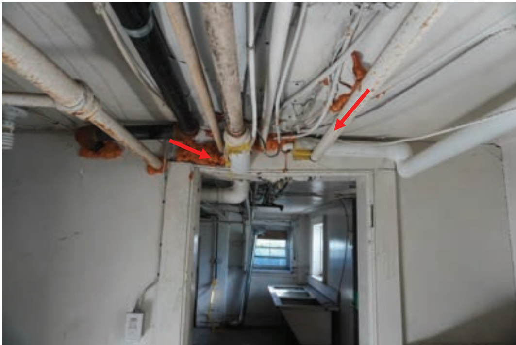
Photo #66: Multiple penetrations have been made through a door header that is observed to be failing. There is a wall on the first-floor level directly above this header.
