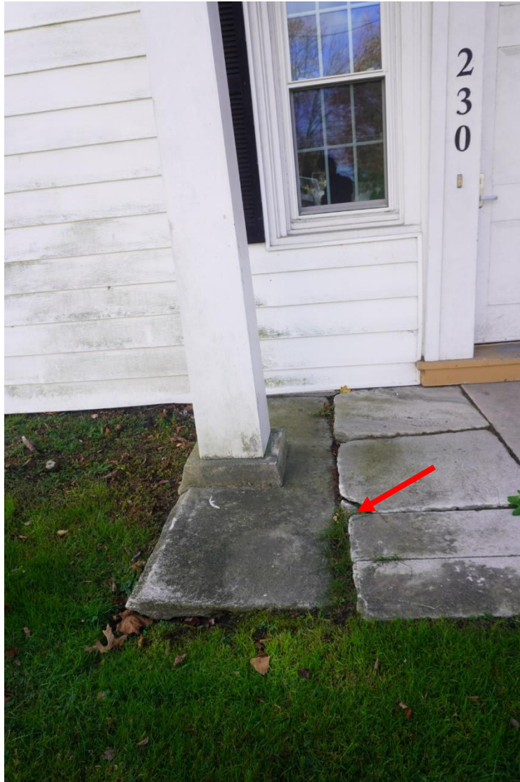
Photo #19: Base of column support for front portico showing signs of differential settlement.
