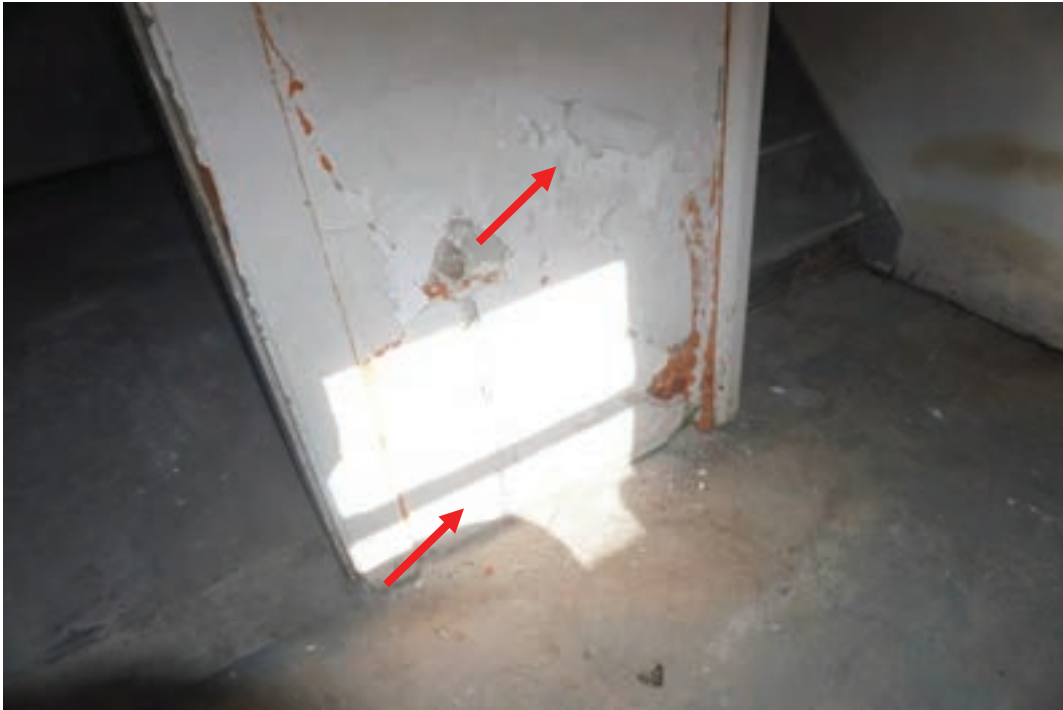
Photo #38: Mold formation and deteriorating damp plaster interior walls at cellar level due to water wicking up through cellar floor.
