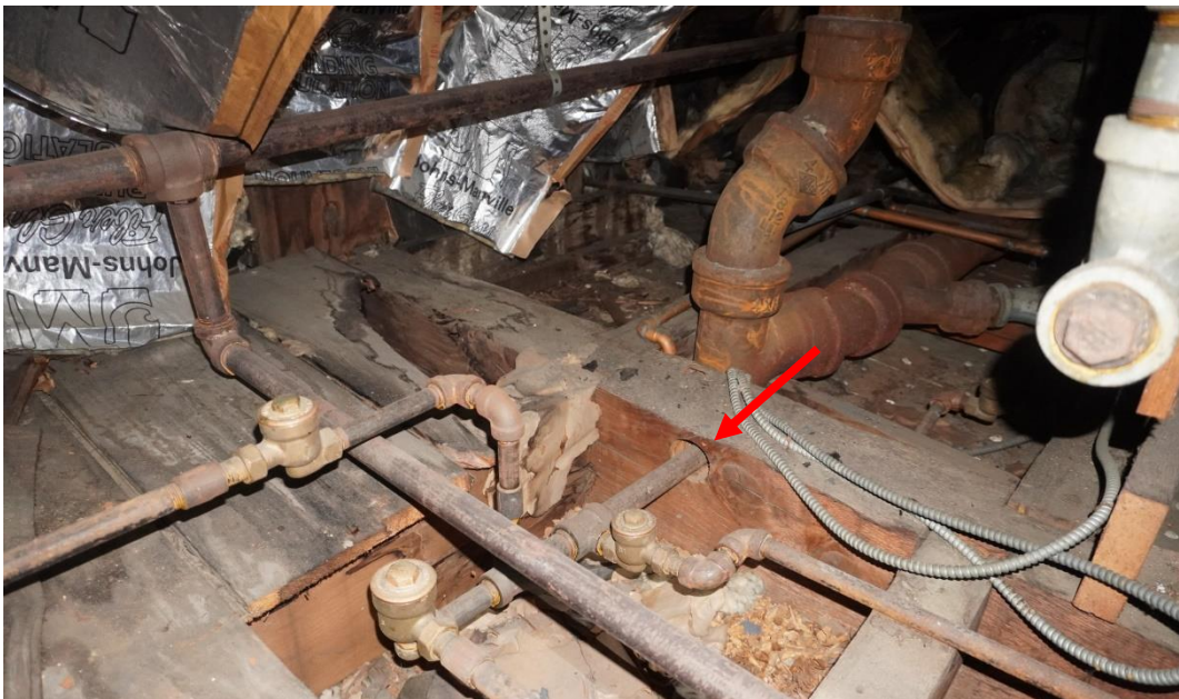
Photo #110: Pipe penetration drilled through girder drilled above its neutral axis. Observed in unfinished attic area, north side of original structure.
