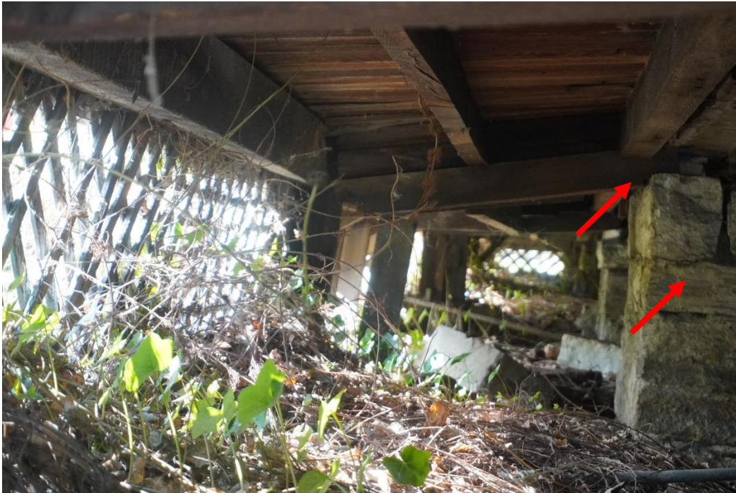
Photo #34: Rear porch sitting on stone pillars that are showing signs of deterioration.
