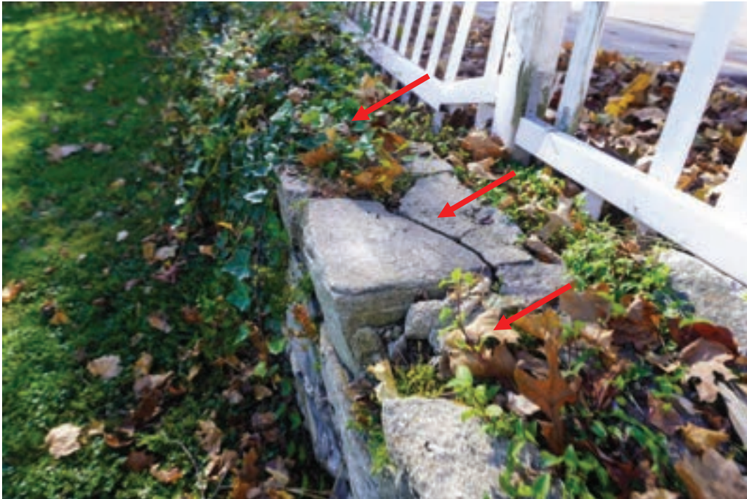
Photo #11: Retaining wall that runs between rear yard and adjacent sidewalk deteriorating throughout. Broken stones and joints between stones have filled with dirt/ organic growths.
