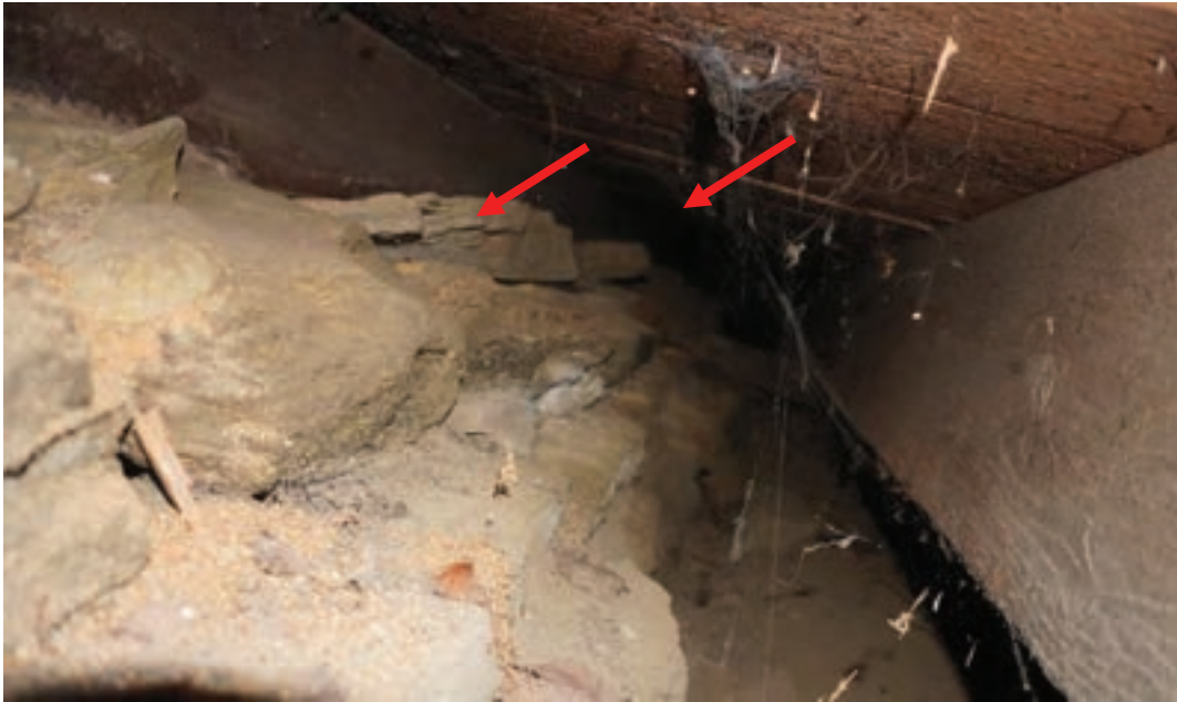
Photo #73: Exterior foundation along north side of home below sill beam is deteriorating and observed to have displaced. (Probe #1)
