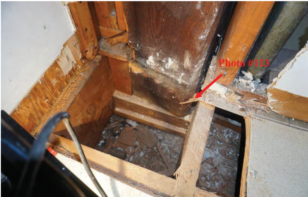
Photo #112: Post in attic space has moved out of place. Mortise and tenon joint that was connecting post to girder below has failed allowing member to rotate (Probe #11).
