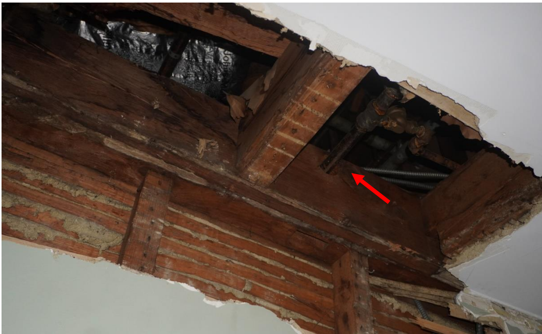
Photo #100: Floor joists supporting attic above observed at second floor level are oriented east to west. Large hole drilled through girder for pipe penetration (Probe #7).
