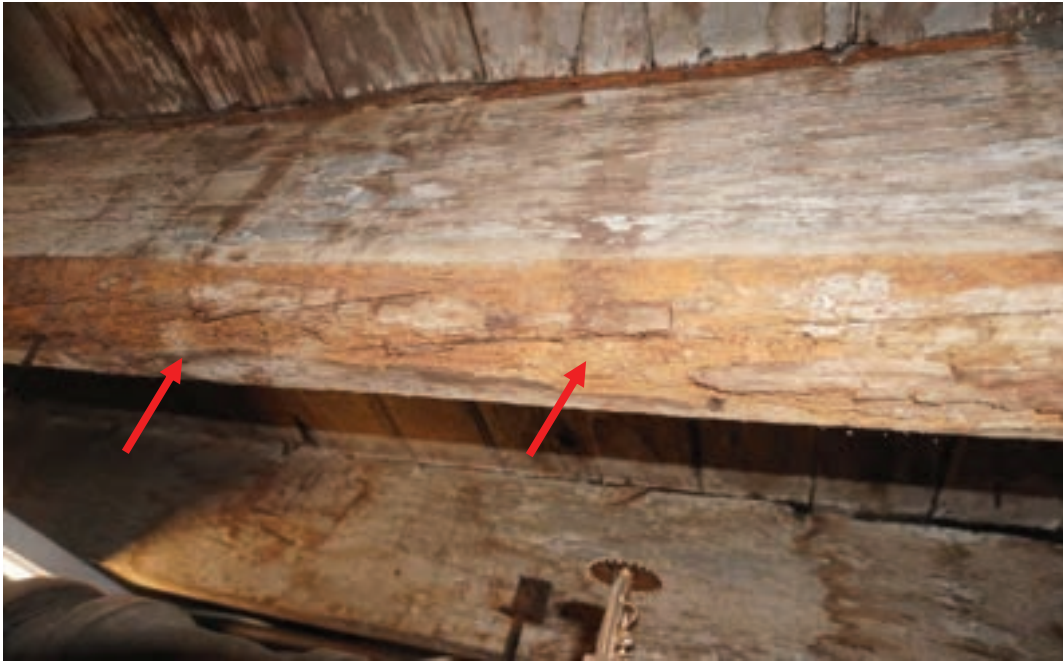
Photo #61: Wood joist observed to have a large extent of termite damage. need to determine if remaining section in this species meets the load; most members are significantly oversized
