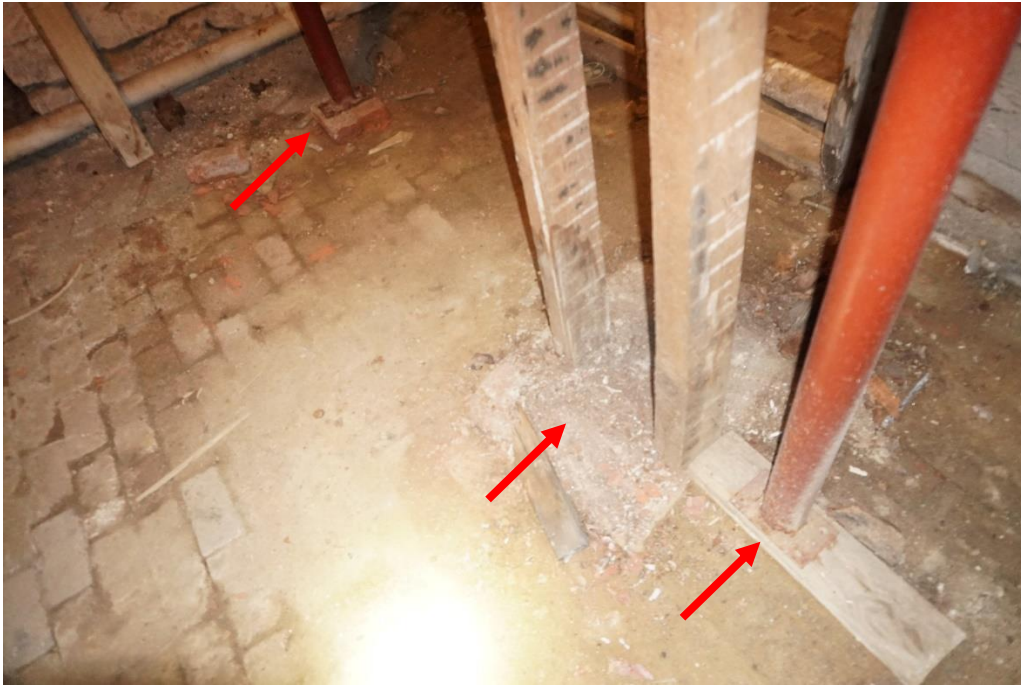
Photo #44: Concrete footings were never poured beneath temporary support columns that were added to prop of both failing girders in the cellar.
