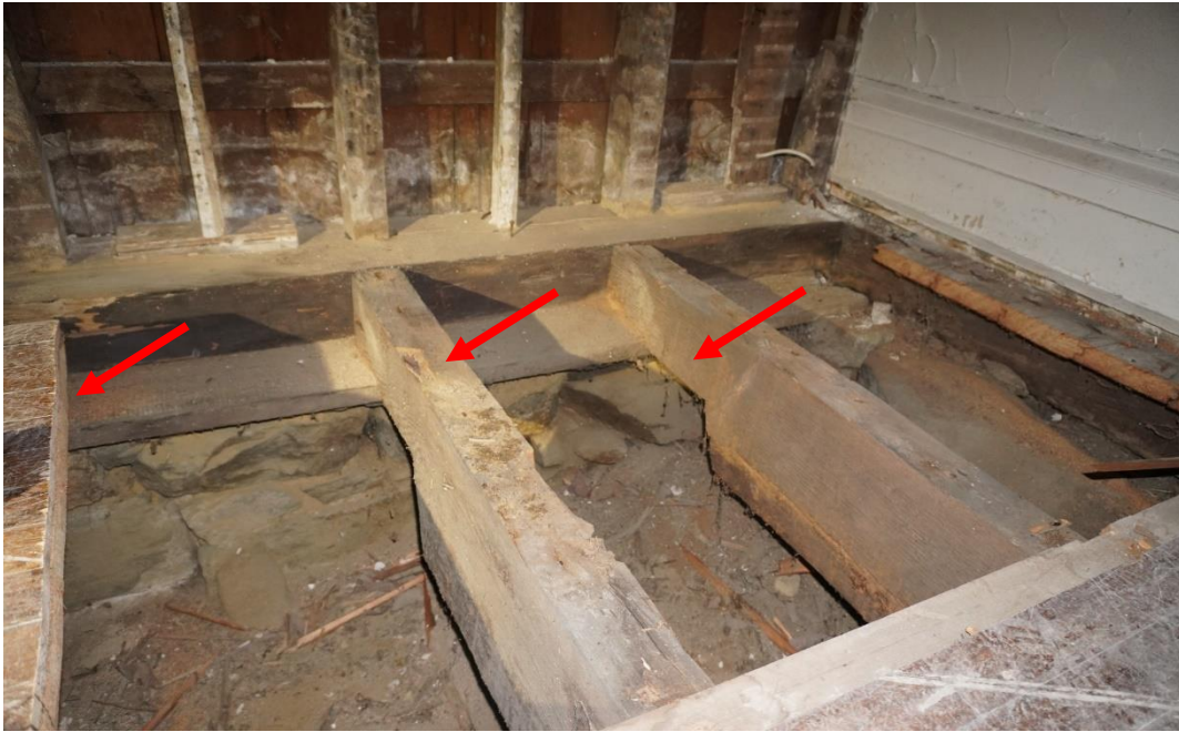
Photo #67: Joists spanning crawlspace sit on a thin sill plate which is not a standard timber framing technique. Typically, wood joists would be notched into the sill beam with use of a mortise and tenon connections (Probe #1).
