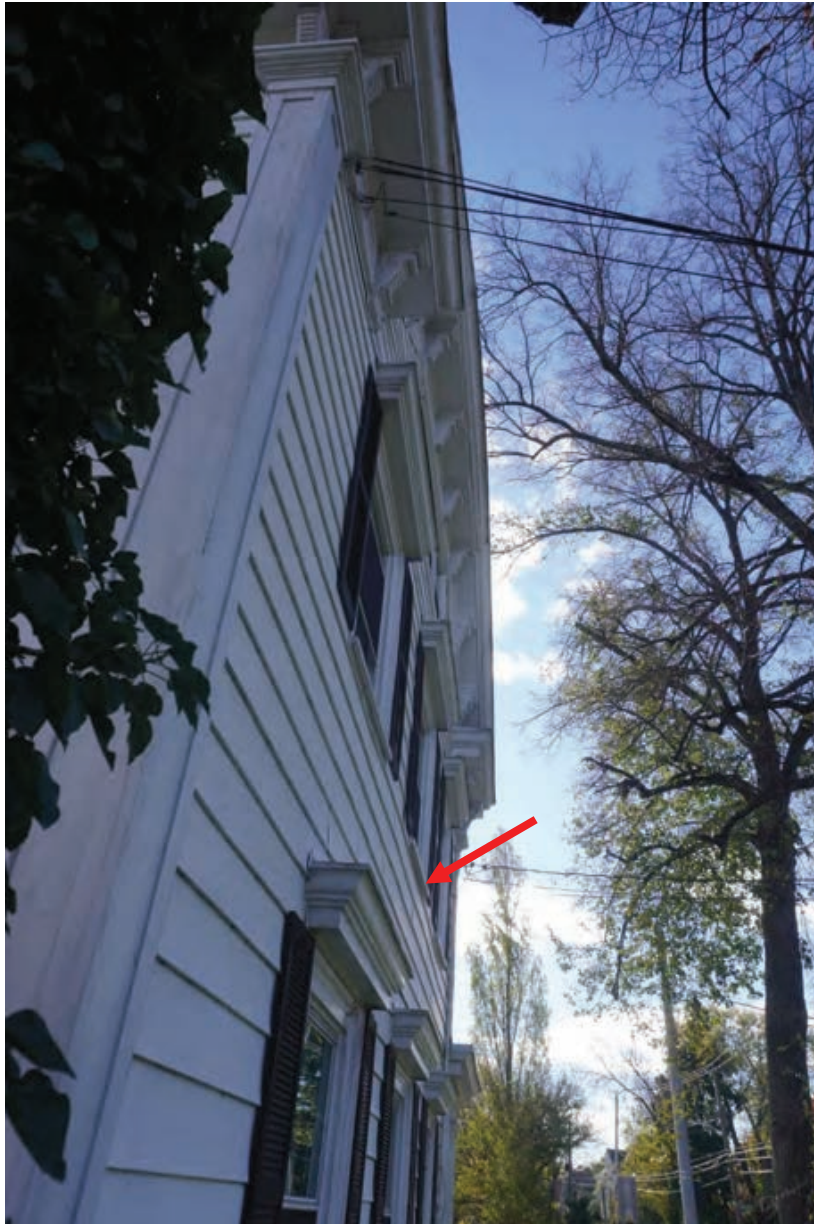
Photo #22: Bulge noticed between first and second floors, west façade of home. Cause unknown. Further investigation required.
