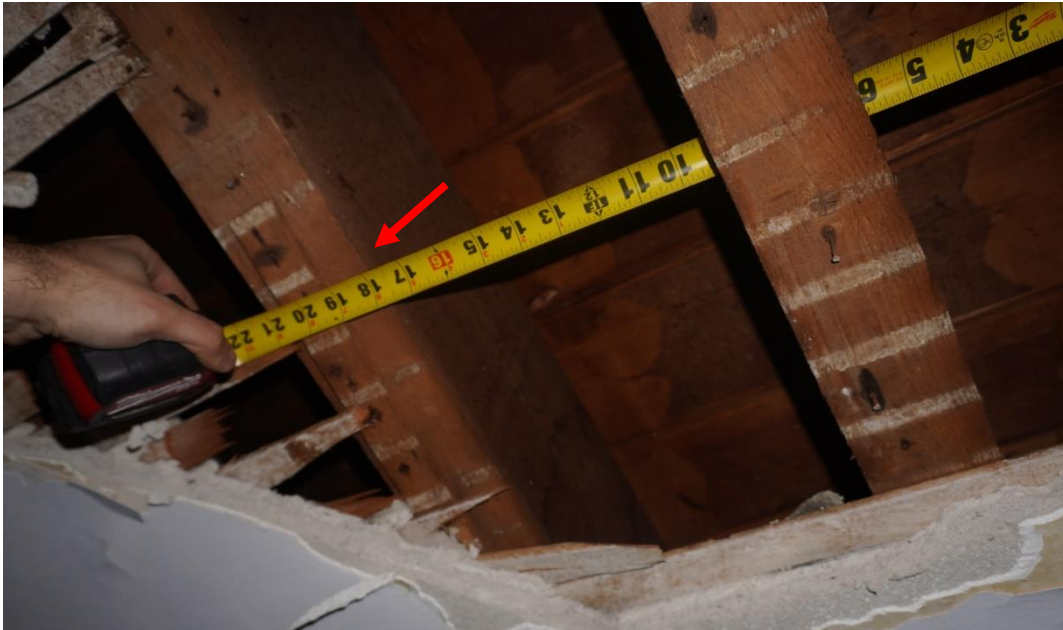
Photo #85: Joists above faux soffit are running north to south and are spaced at 18” inches apart. All other floor joists observed in the original structure above the ground level are running perpendicular to these joists (Probe #3). Further investigation required.
