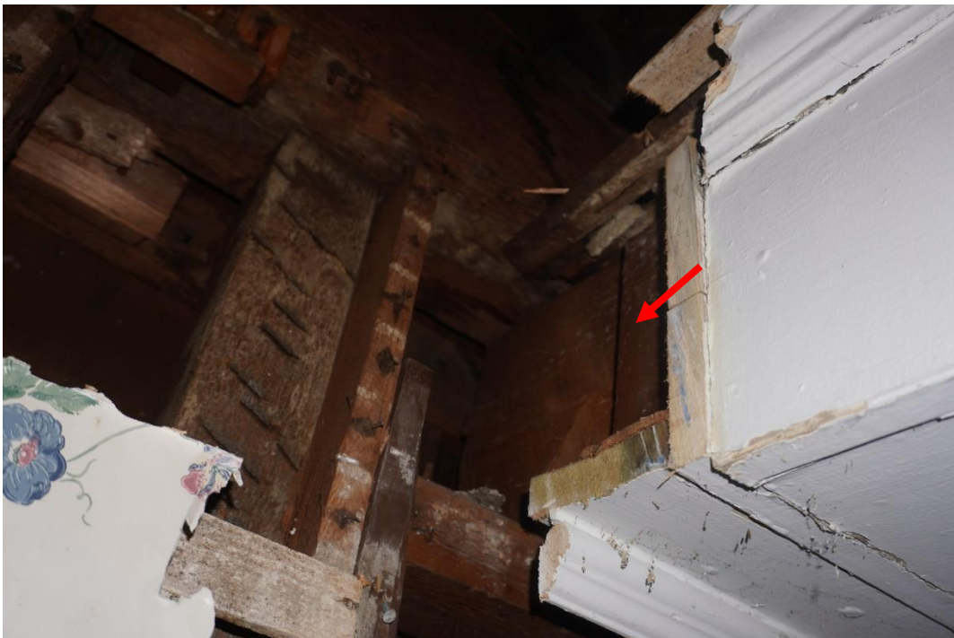
Photo #80: Large beam observed in ceiling soffit spanning east to west. Beam is acting as a midspan support for floor joists above that span north to south (Probe #2).
