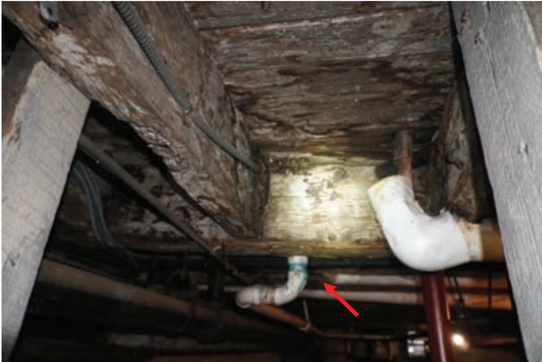
Photo #63: Plumbing pipe drilled directly through main girder in the vertical direction, west end of cellar. plumbers again; often redundant load paths compensate; does not appear to be movement here.
