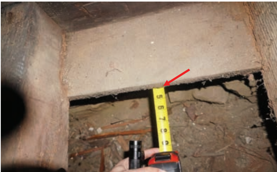
Photo #72: Crawl space joists sit on a 7-inch sill plate that is only bearing 3 inches onto deteriorating foundation below. Sill plate has a four-inch unsupported overhang (Probe #1).
