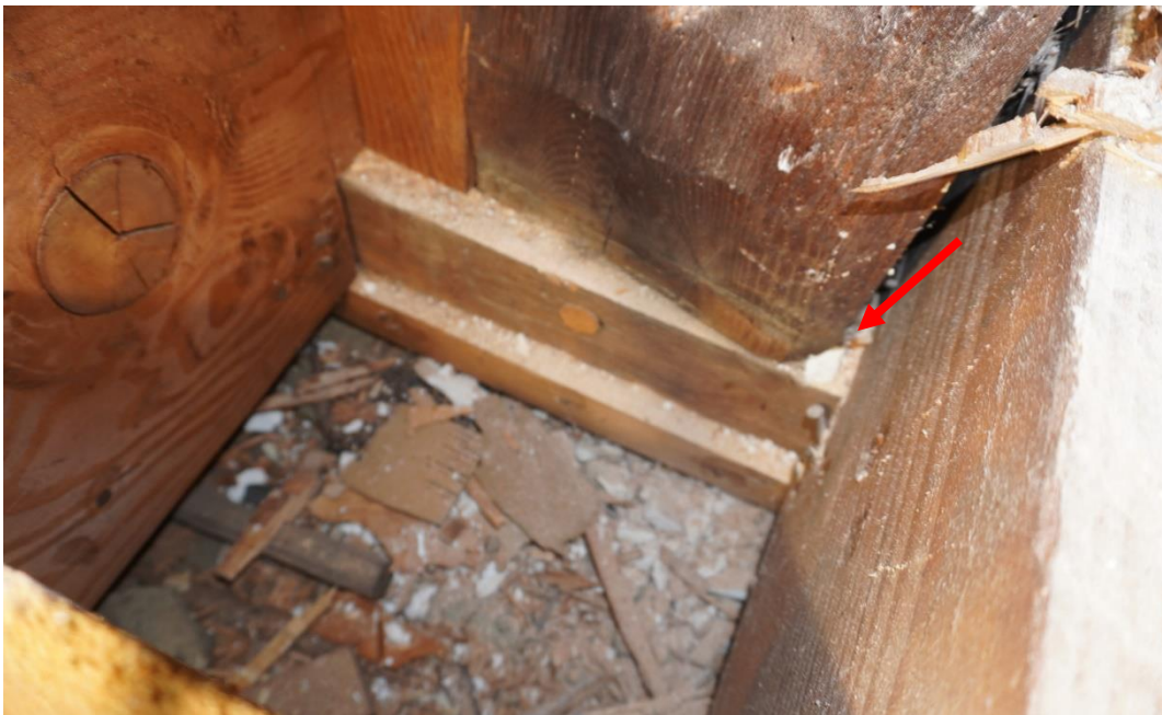
Photo #113: Post in attic space has moved out of place. Mortise and tenon joint that was connecting post to girder below has failed allowing member to rotate (Probe #11).
