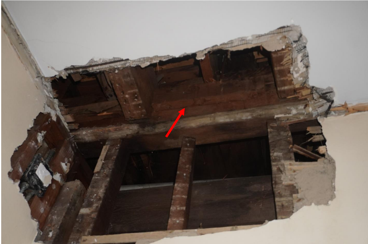
Photo #103: New joists running east to west have been installed at higher level than original joists and are resting on a 2x4 wood ledges that have been nailed to girder to support attic floor above. It is unclear why these joists were installed. Most likely to add additional space for piping below showers and toilets in attic. Further investigation required. Original joists left in place and still supporting ceiling below (Probe #8).
