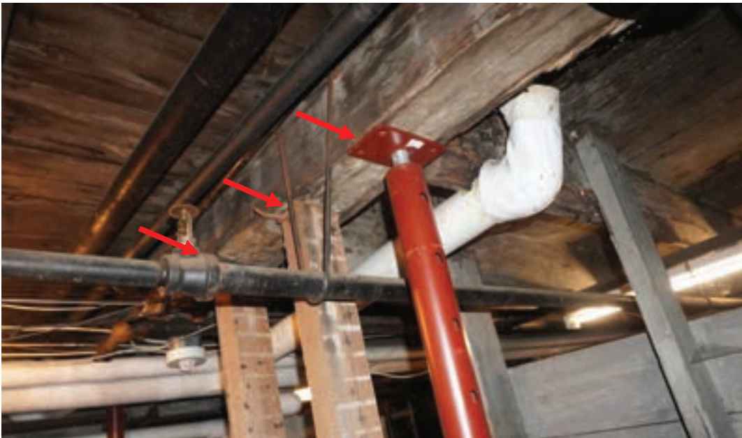
Photo #64: Temporary support columns being used to hold failing 6-3/4"x10-1/2" girder in place west end of cellar. Columns are not mechanically attached to girder above and do not have proper footings.
