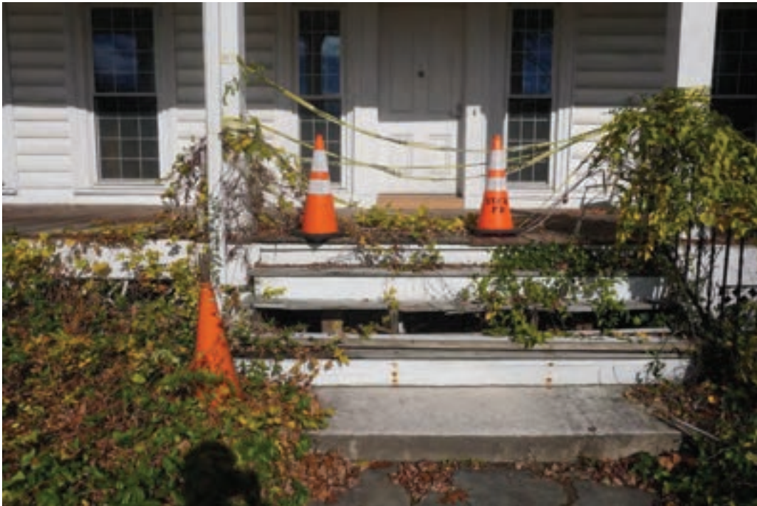
Photo #35: Rear porch stairs deteriorated. No longer usable. Unsafe condition. agree; porches and exterior wood steps need periodic TLC!
