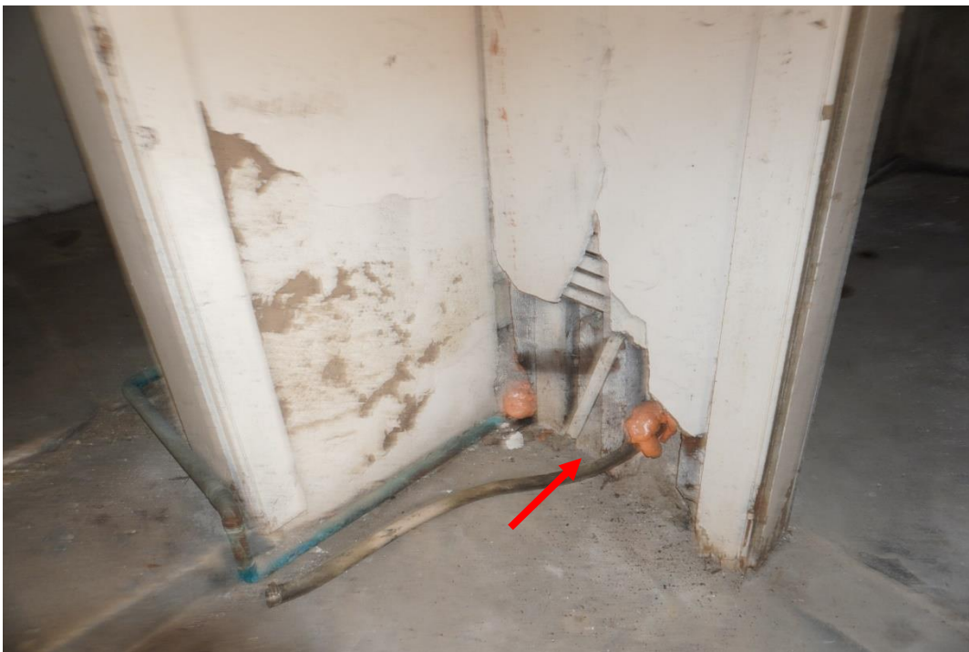
Photo #39: Mold formation and deteriorating damp plaster interior walls at cellar level due to water wicking up through cellar floor.
