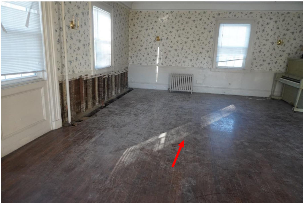
Photo #76: Location of west chimney that was relocated at some point in the past. Foundation still in place and can be observed in cellar below.
