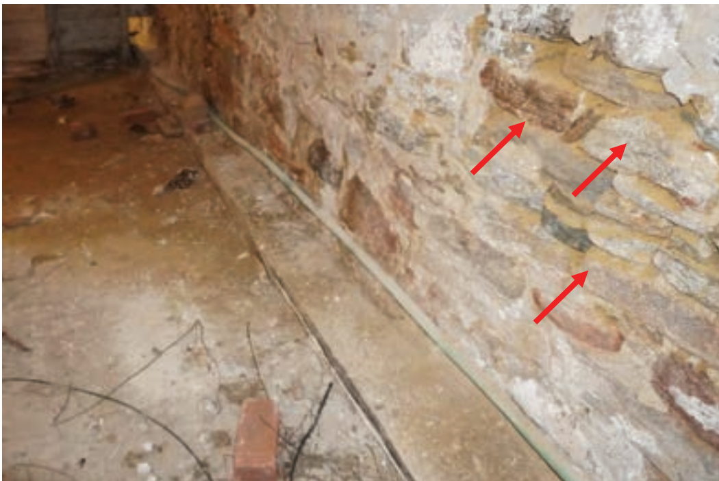
Photo #47: Water infiltrating through foundation is bringing in soil through spaces between dry laid rubble stone walls. Soil piling along inside of foundation walls.
