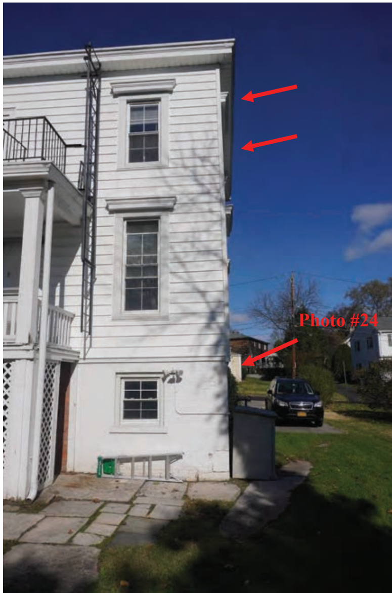
Photo #23: Southeast corner of structure showing signs of inwards movement towards the top. Cause unknown. Further investigation required.
