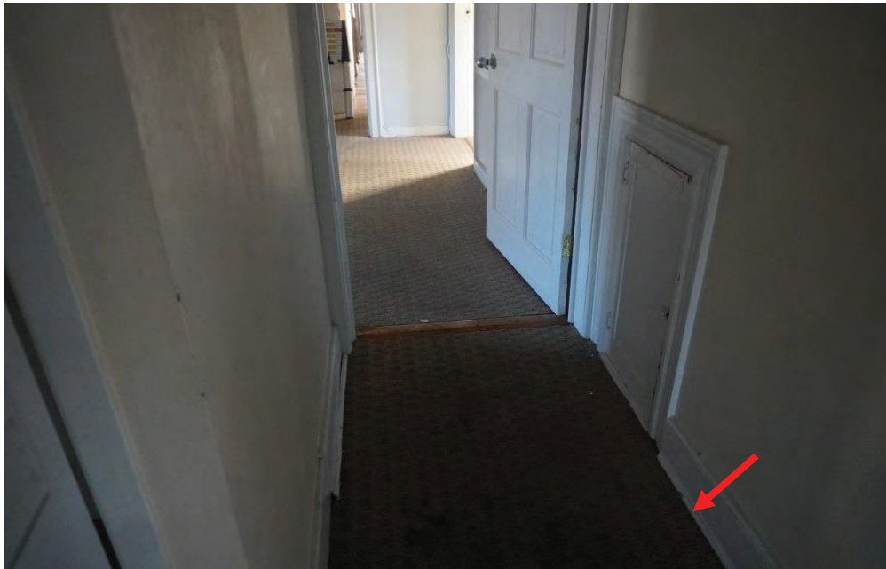
Photo #99: Depression in second floor hallway. Most likely due to weight of walls and bathroom added in this area. Further investigation would be required to figure out exact cause.
