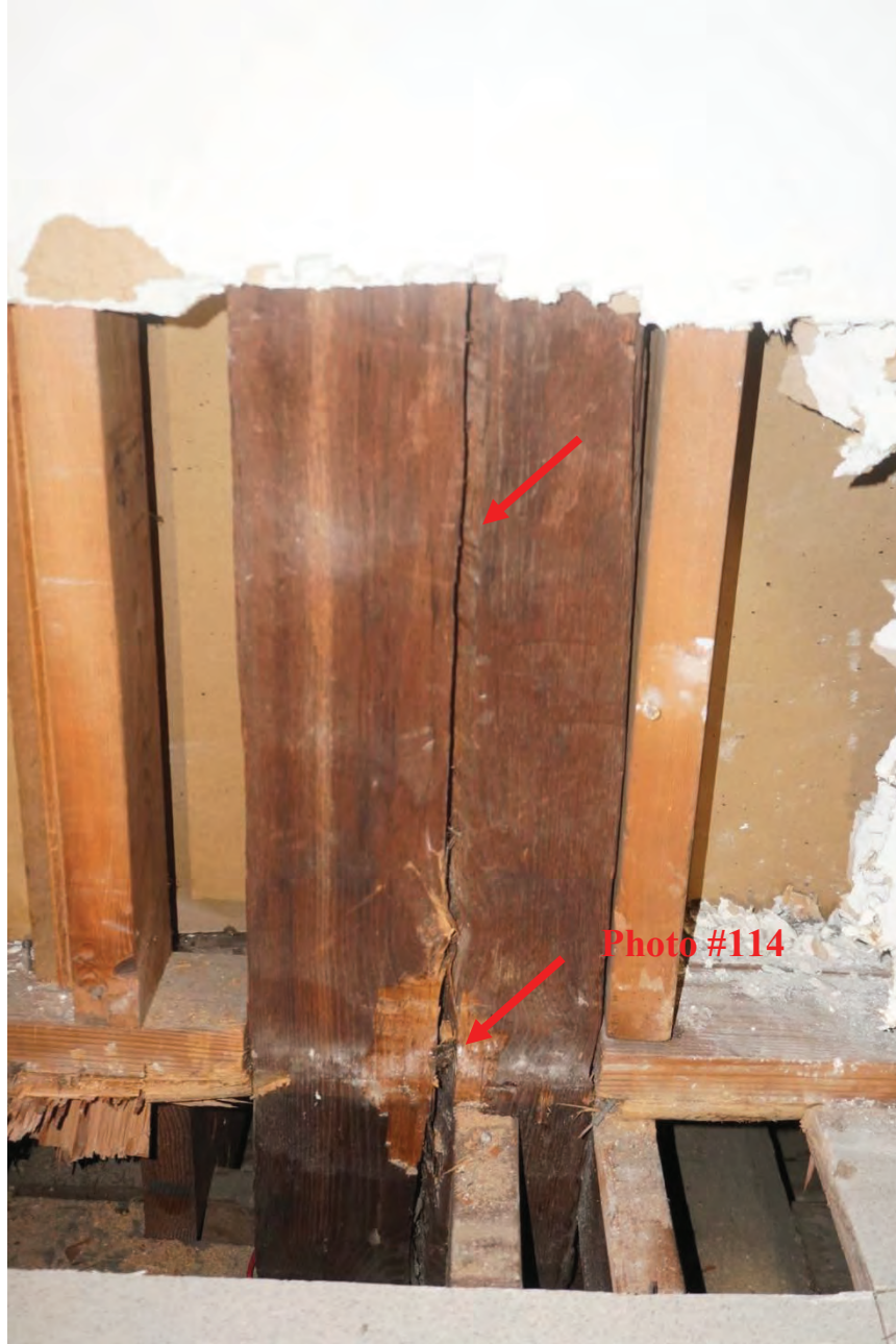
Photo #114: Vertical crack that has opened more towards the bottom observed, attic post Unclear why this has occurred. Further investigation required (Probe #12).
