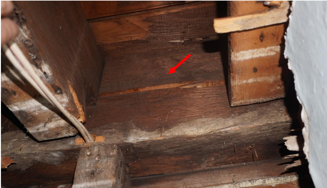
Photo #93: Interior girder running north to south is splitting along the mortise and tenon joint connections (Probe #4).
