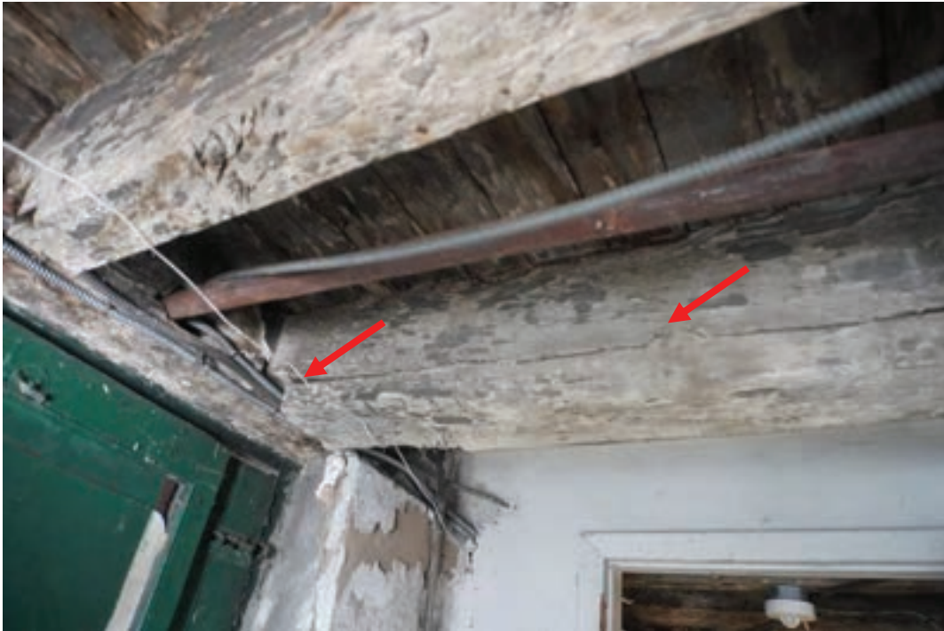
Photo #50: Horizontal crack from shear stress resonating down entire member from notch at end of beam.
