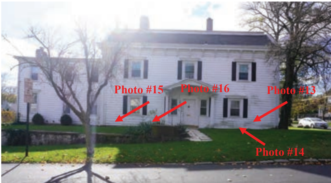
Photo #12: Foundation along front façade of original structure is low and at same level as grading. Water can infiltrate above foundation wall and rot out wood sill beam that runs along top of foundation.
