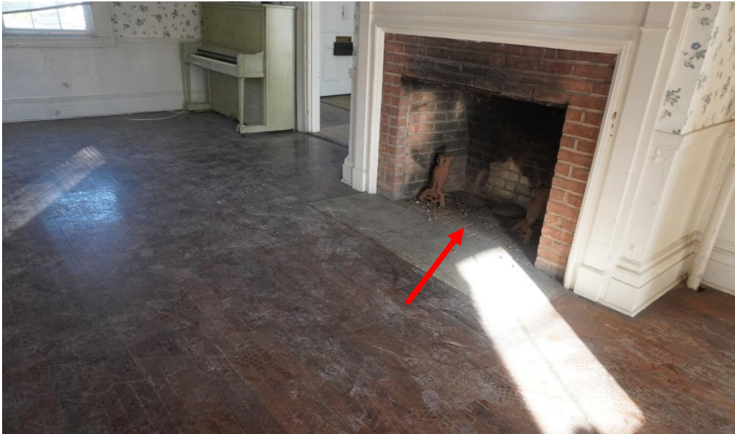
Photo #77: Chimney was added to this location at some unknown point in the past. Presumably when the original west chimney was demoed.
