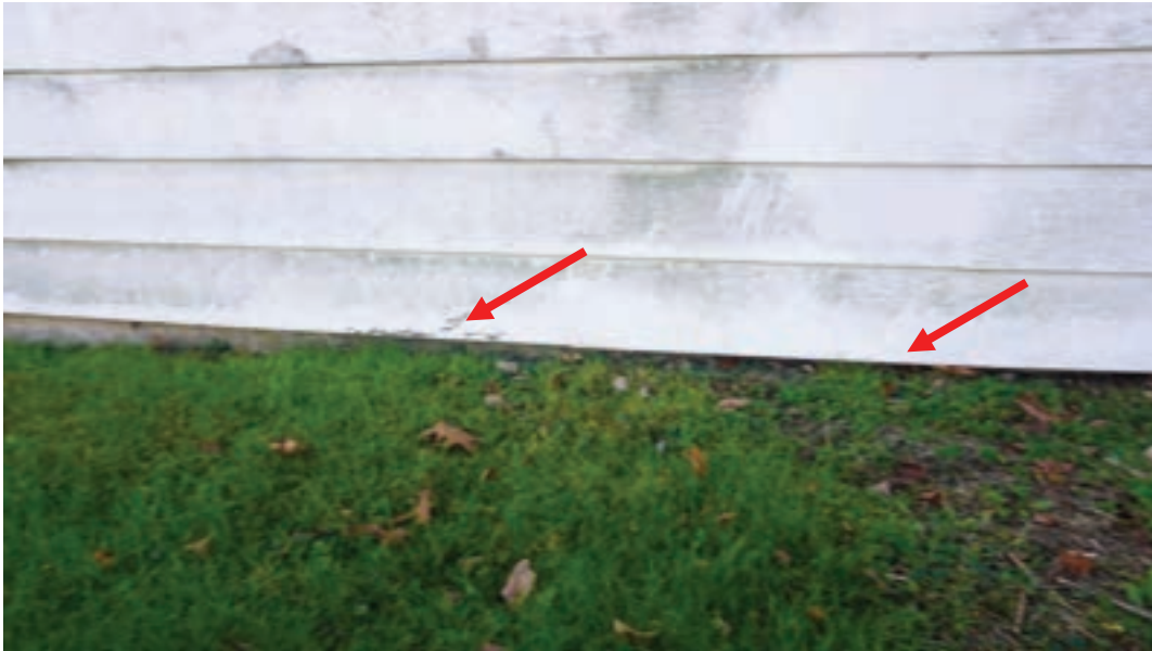
Photo #15: Foundation along front façade of original structure is low and at same level as grading. Water can infiltrate above foundation wall and rot out wood sill beam that runs along top of foundation.
