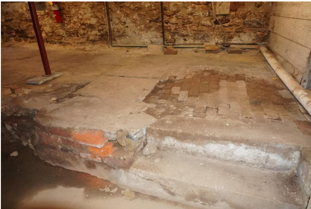
Photo #45: Cellar floor observed to be composed of bricks with a cement stucco layer that is deteriorating.
