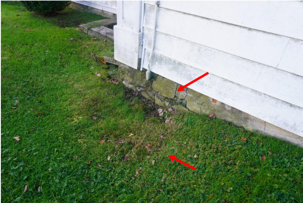
Photo #5: Negative grading front of home between entrance and northeast corner of home. Water pooling up against foundation wall and most likely infiltrating into crawlspace. Signs of foundation deterioration.
