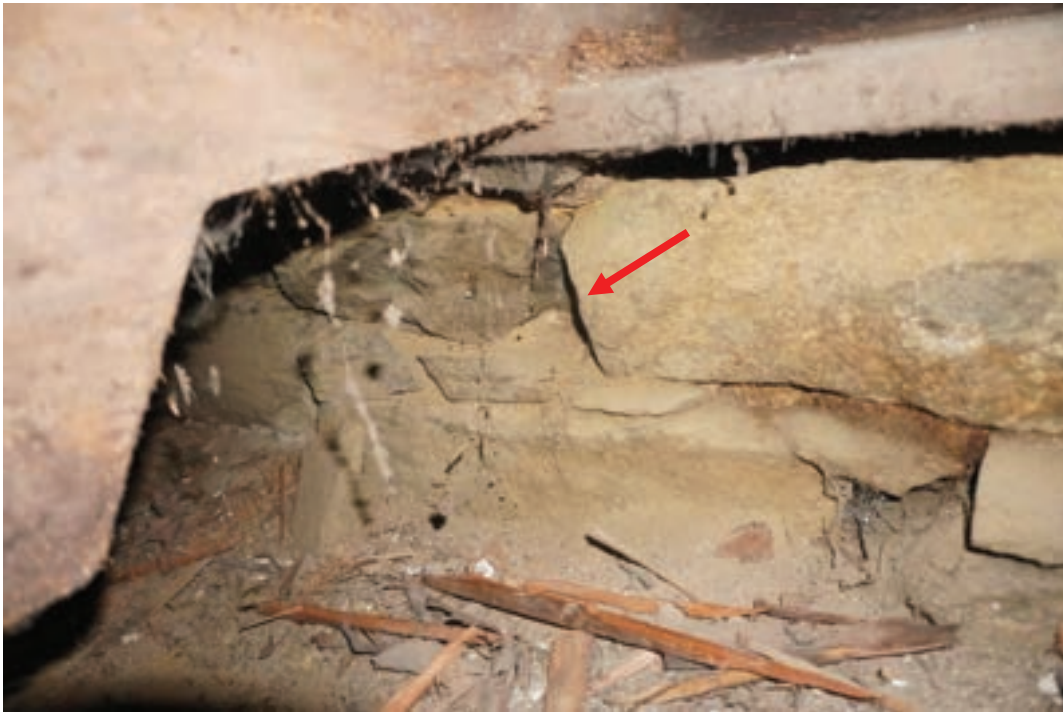
Photo #68: Thin sill plate, joists spanning crawlspace are sitting on, is being supported by a rubble stone foundation wall that is coming apart (Probe #1).
