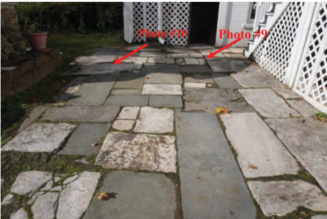
Photo #8: Stone slabs have settled/ heaved creating multiple trip hazards, stone patio rear yard.
