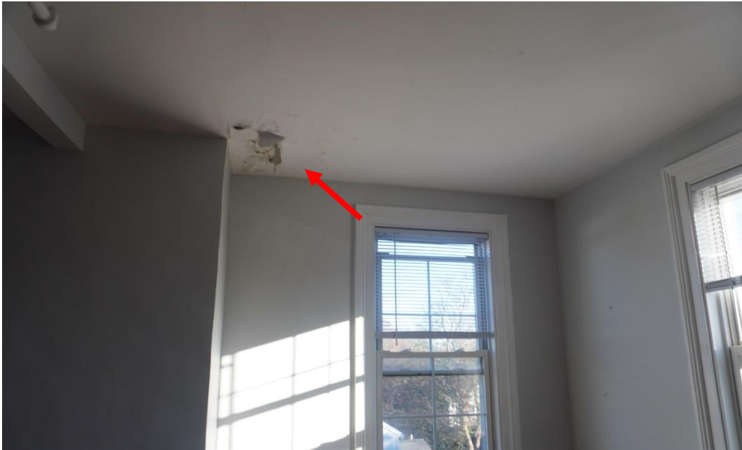
Photo #107: Water damage adjacent to east exterior wall of addition. Cause unknown, further investigation required.
