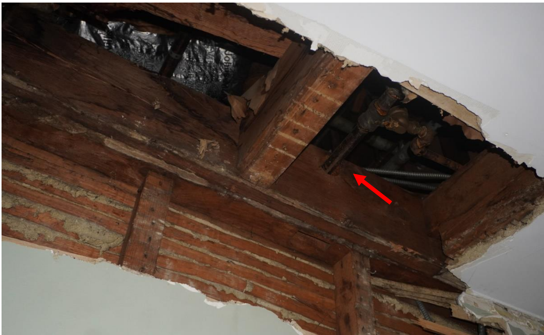
Photo #100: Floor joists supporting attic above observed at second floor level are oriented east to west. Large hole drilled through girder for pipe penetration (Probe #7).
