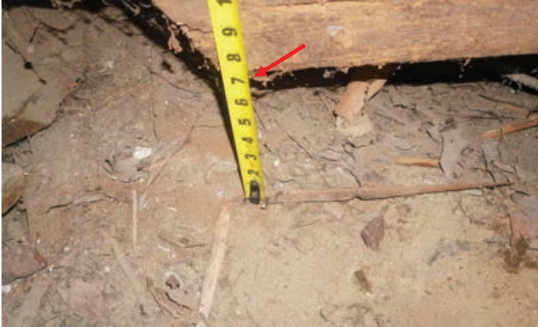
Photo #74: Wood joists in crawlspace are sitting 7 inches above exposed dirt beneath crawlspace. Crawlspace is inaccessible. Crawlspace foundation most likely does not extend below the frost line (Probe #1). Further investigation required.
