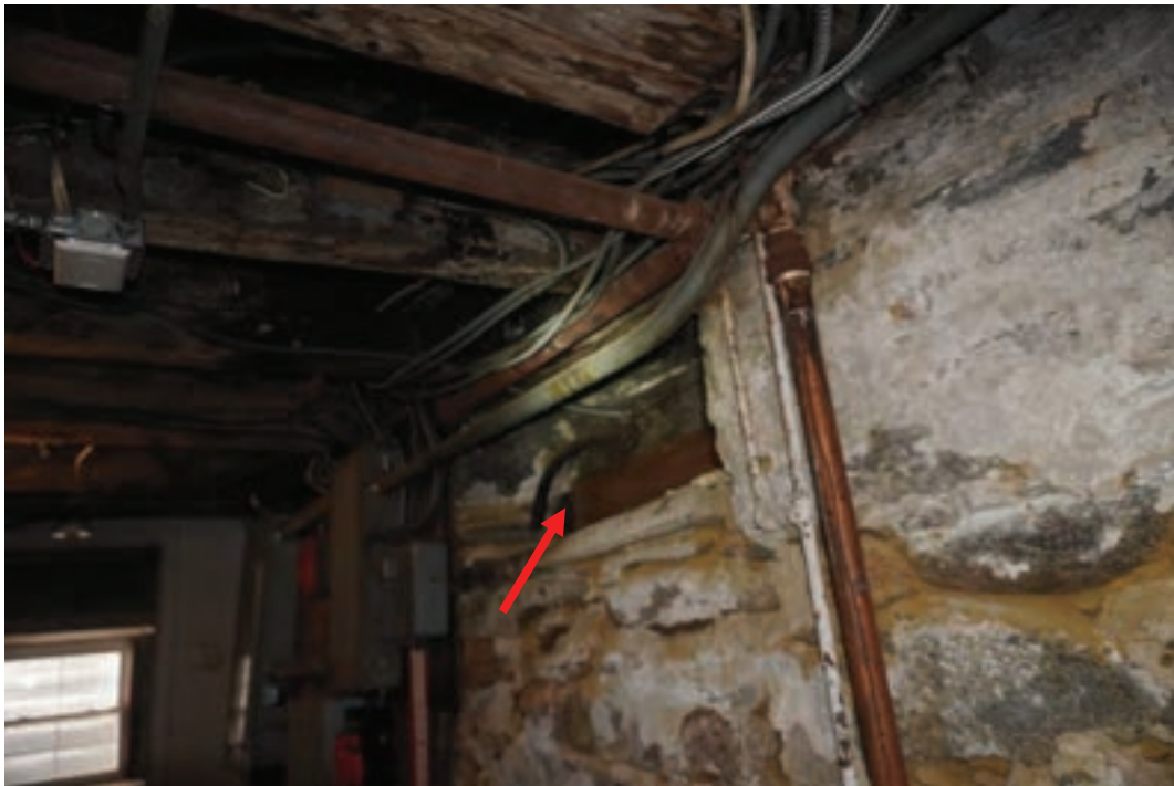
Photo #58: Cellar window at boiler room south foundation wall has been covered up when porch was added to the rear of the home.
