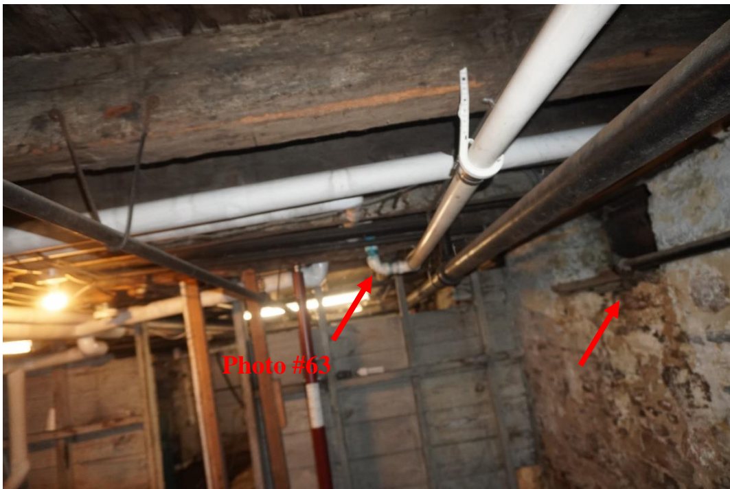
Photo #62: Cellar window (second location) at west end of home on south foundation wall has been covered up when porch was added to the rear of the home. Plumbing pipe drilled directly through main girder in the vertical direction, west end of cellar.
