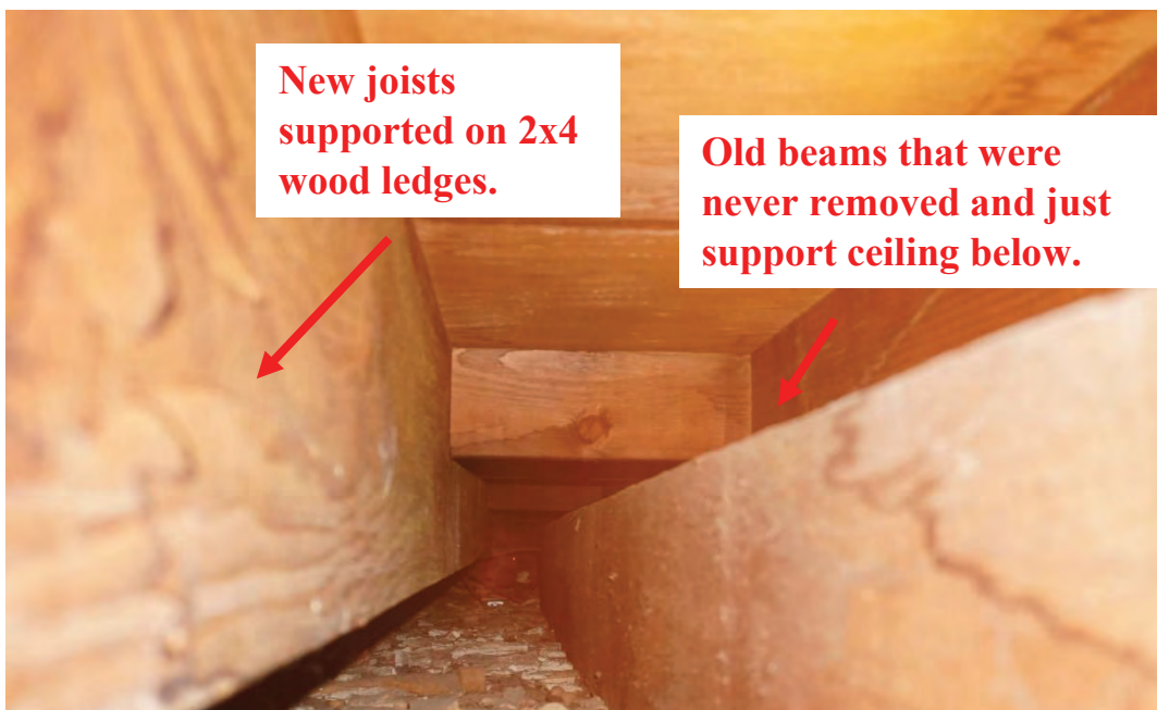
Photo #106: New joists running east to west have been installed at higher level than original joists and are resting on a wood ledge 2x4s that have been nailed to girder to support attic floor above (Probe #8). (Probe #8)
