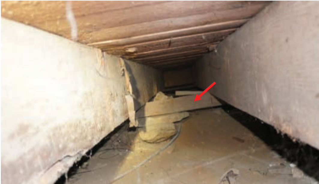
Photo #75: Wood joists spanning crawl space are being inadequately supported at midspans by wood members that are balanced above unstable pieces of stone (Probe #1).
