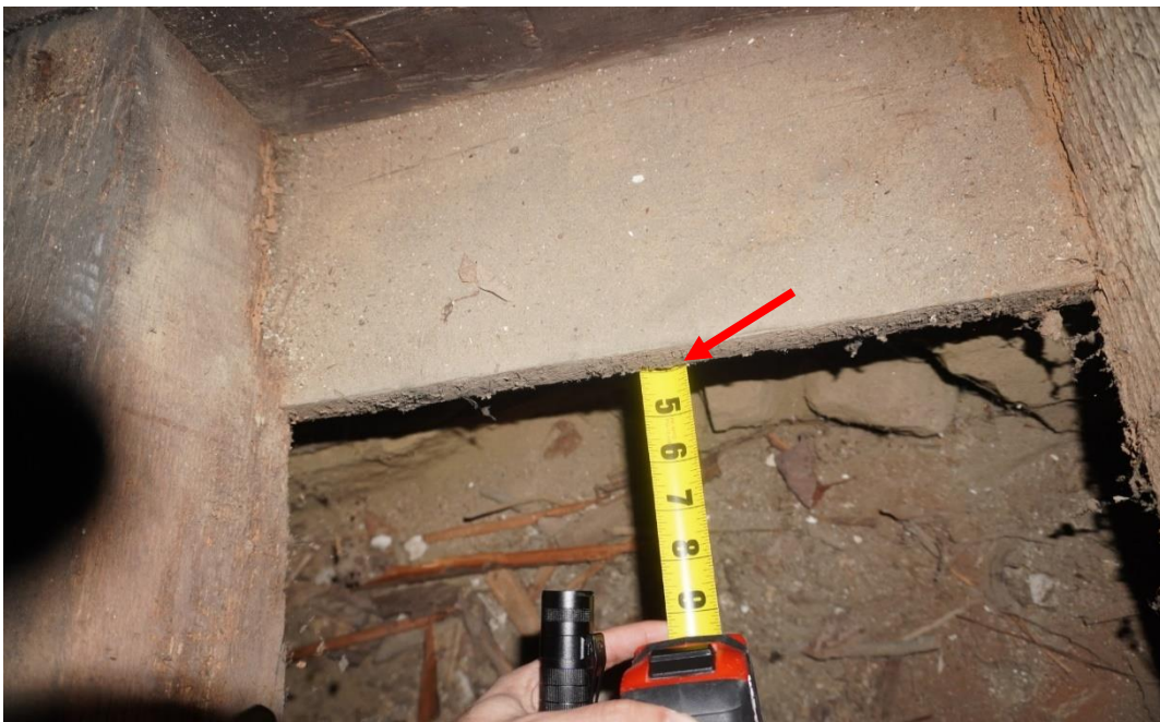
Photo #72: Crawl space joists sit on a 7-inch sill plate that is only bearing 3 inches onto deteriorating foundation wall below. Sill plate has a four-inch unsupported overhang (Probe #1).
