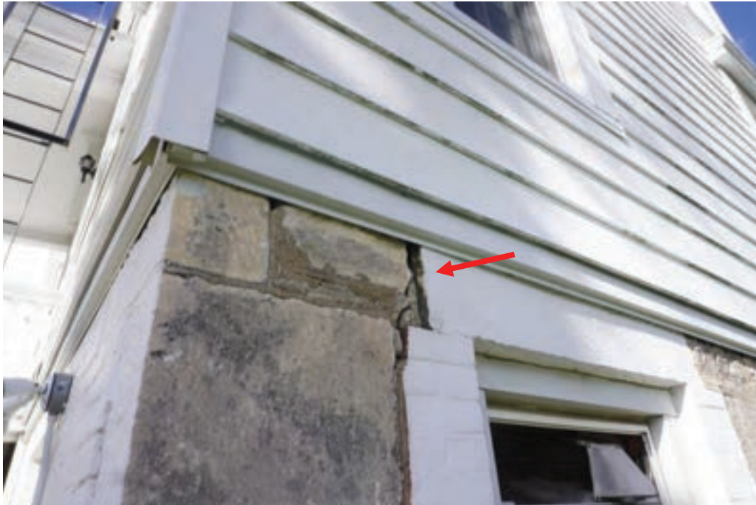
Photo #24: Vertical crack ground level stonework east façade, southeast corner of structure at addition.
