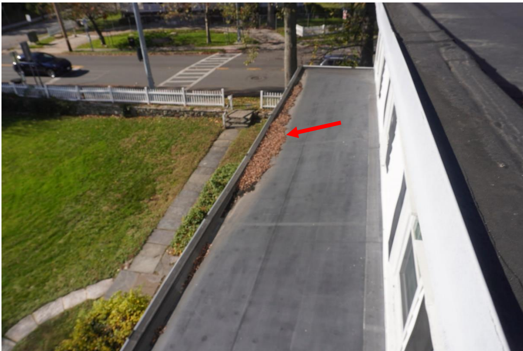
Photo #27: Rear porch roof deflecting over stairs causing water to pool and leaf build up.
