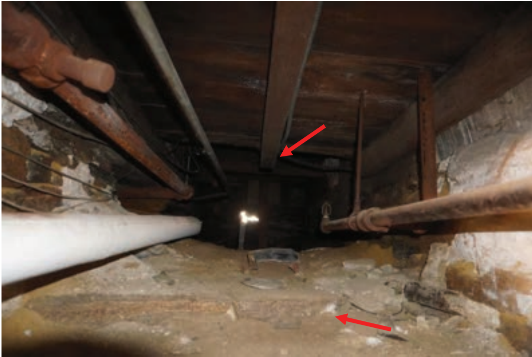
Photo #53: Joists connections in crawlspace observed to be coming apart. Piping was run into crawlspace through what potentially was an old window in original foundation wall.
