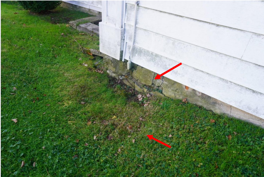
Photo #5: Negative grading front of home between entrance and northeast corner of home. Water pooling up against foundation wall and most likely infiltrating into crawlspace. Signs of foundation deterioration.
