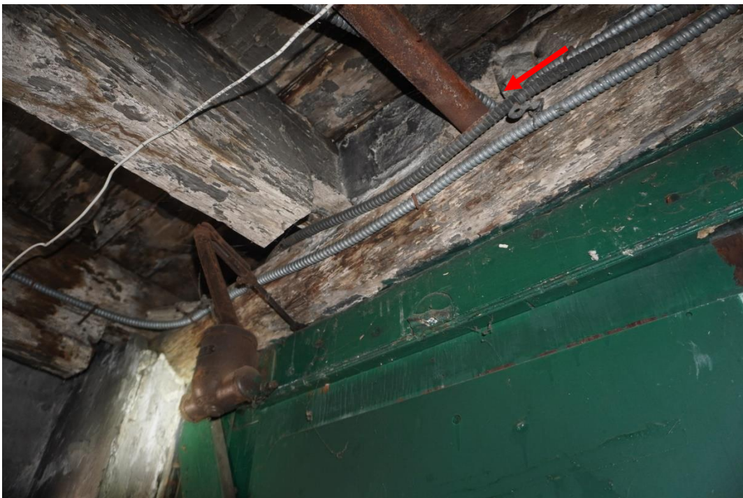
Photo #49: Pipe penetration drilled through door header leading out to rear yard.
