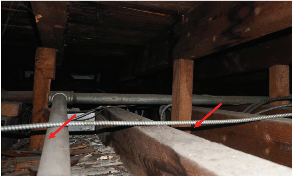
Photo #109: View facing northeast in roof void between 2 nd floor ceiling joists and roof joists in the addition. Roof joists do not align with ceiling joists and are being supported at midspan with blocking that is resting right onto plaster ceiling (Probe #9).
