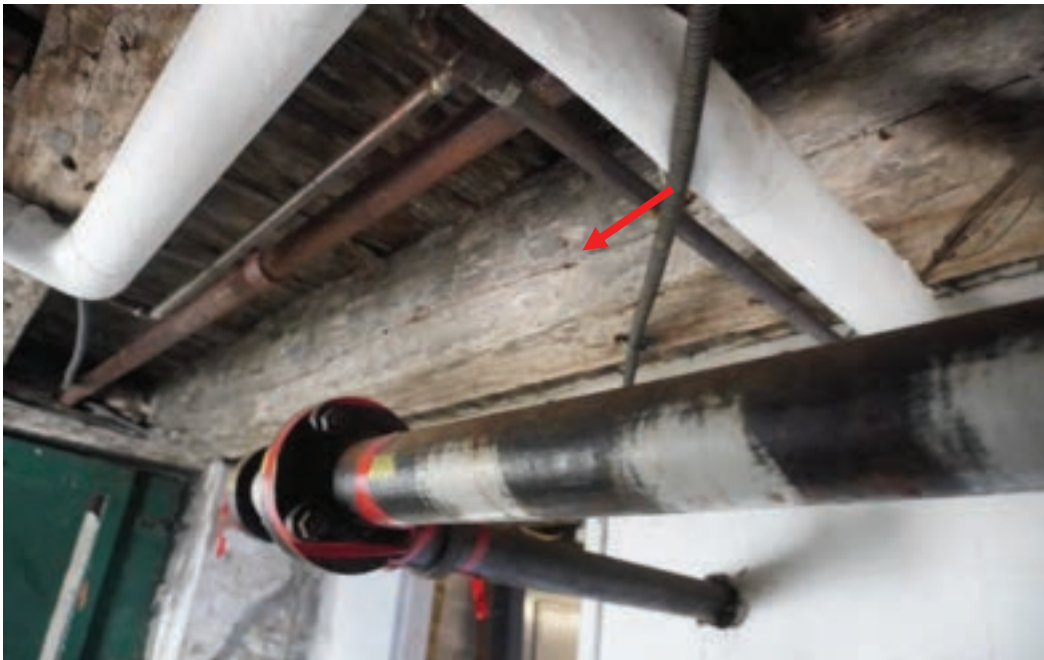
Photo #51: Horizontal crack from shear stress resonating down entire member from notch at end of beam.
