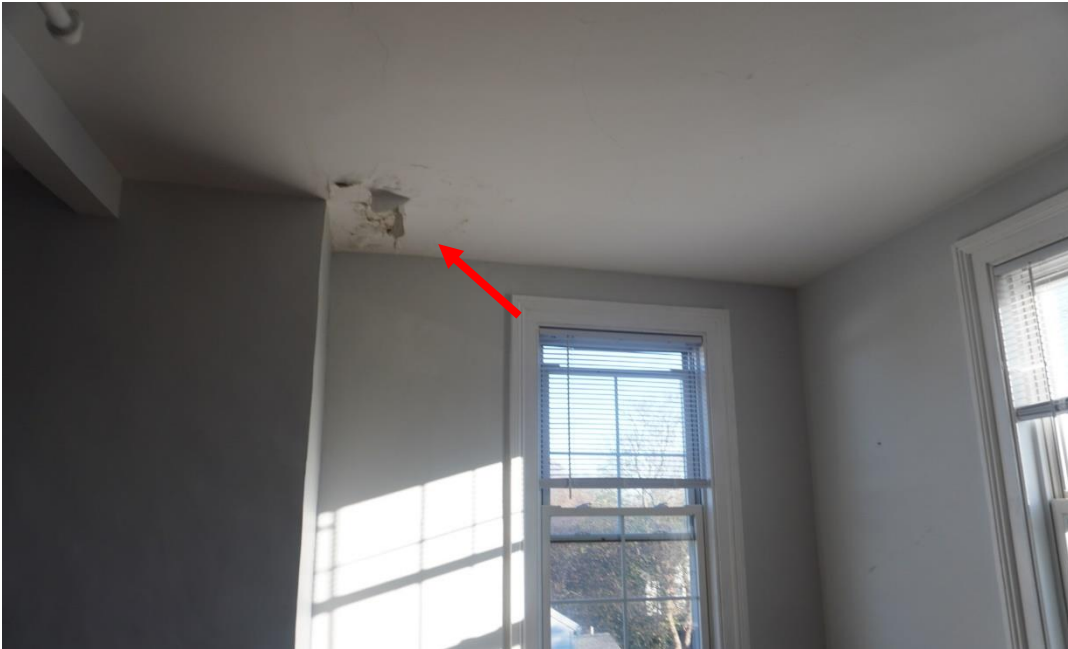
Photo #107: Water damage adjacent to east exterior wall of addition. Cause unknown, further investigation required.
