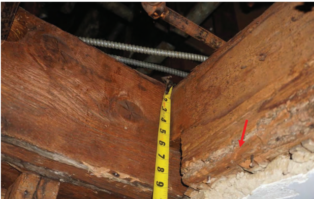
Photo #102: Past termite damage was observed in floor joist supporting attic level (Probe #7). not uncommon but surviving section appears adequate
