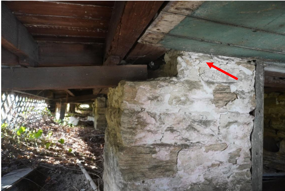
Photo #32: Rear porch sitting on stone pillars that are showing signs of deterioration.
