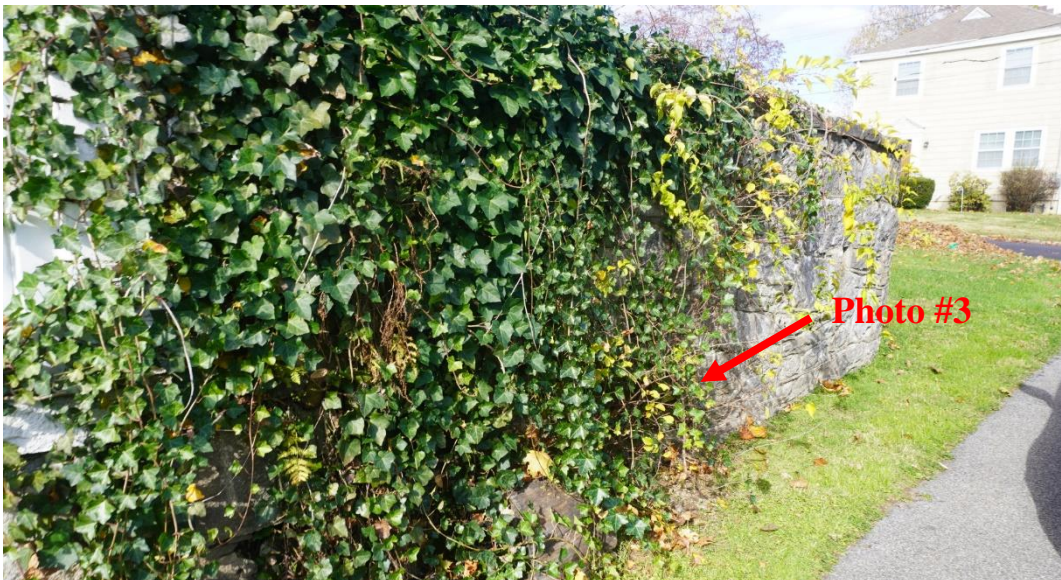
Photo #2: Retaining wall that runs from between front entrance and driveway is deteriorating throughout. Roots/ large weeds growing through joints of walls multiple locations.
