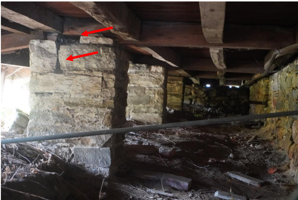
Photo #31: Rear porch sitting on stone pillars that are showing signs of deterioration.
