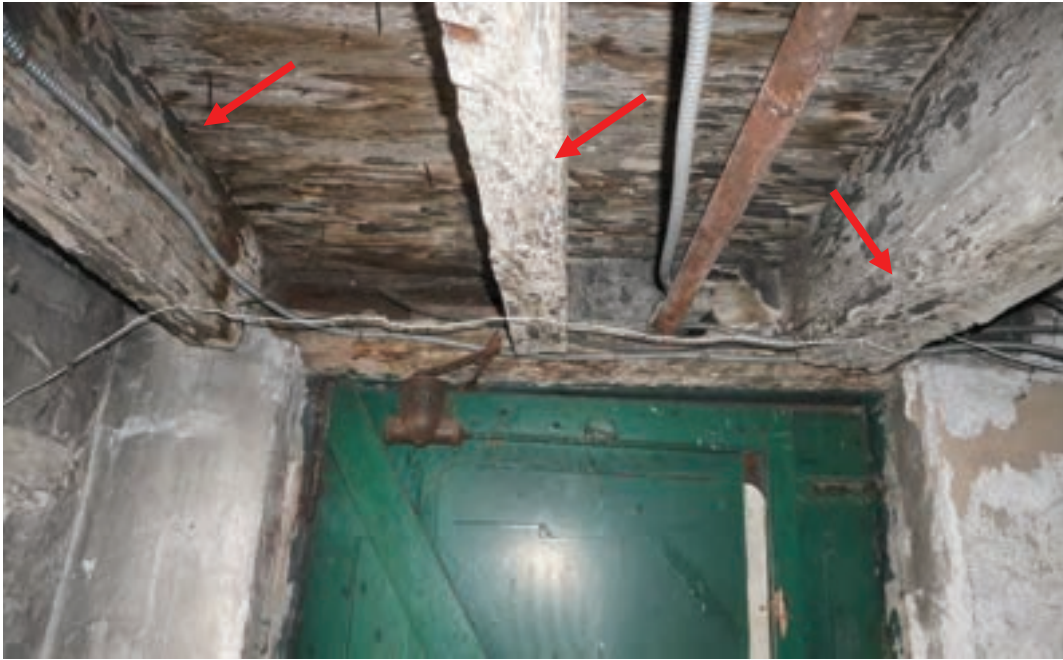
Photo #48: Two 10x3 beams spaced 16 inches apart on left are spanning 19 feet. The reason 6"x9-1/4" beam on right is sized larger than other joists is unclear. It is uncommon for such a large member to be sitting on a door header.
