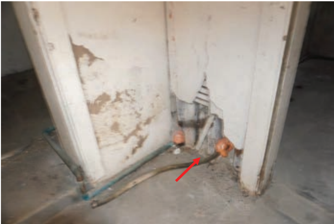
Photo #39: Mold formation and deteriorating damp plaster interior walls at cellar level due to water wicking up through cellar floor.
