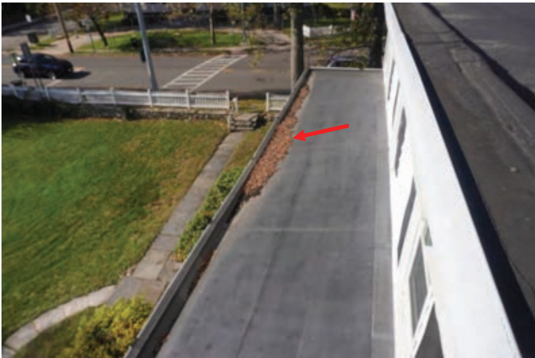
Photo #27: Rear porch roof deflecting over stairs causing water to pool and leaf build up.
