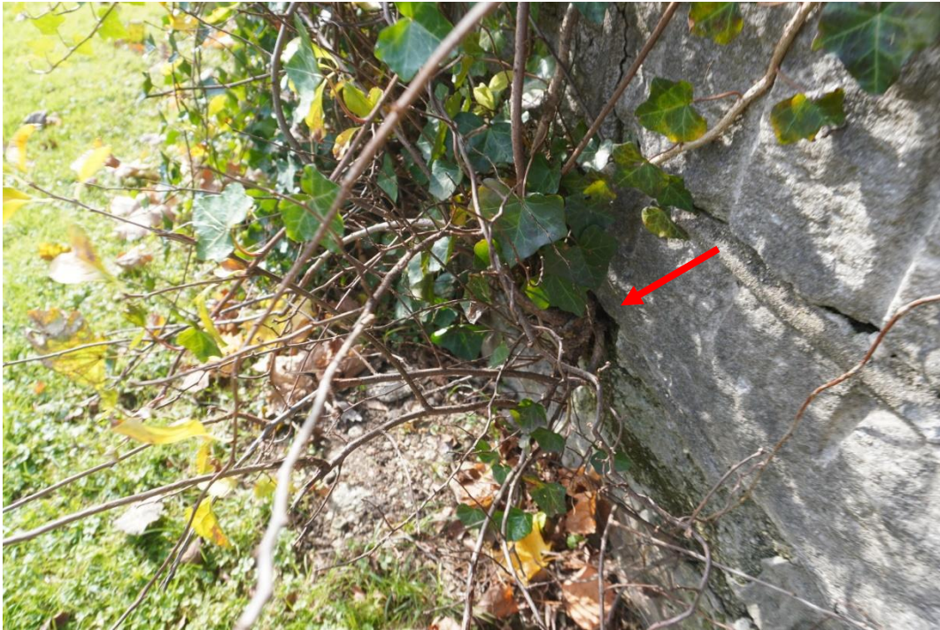
Photo #3: Retaining wall that runs from between front entrance and driveway is deteriorating throughout. Roots/ large weeds growing through joints of walls multiple locations.
