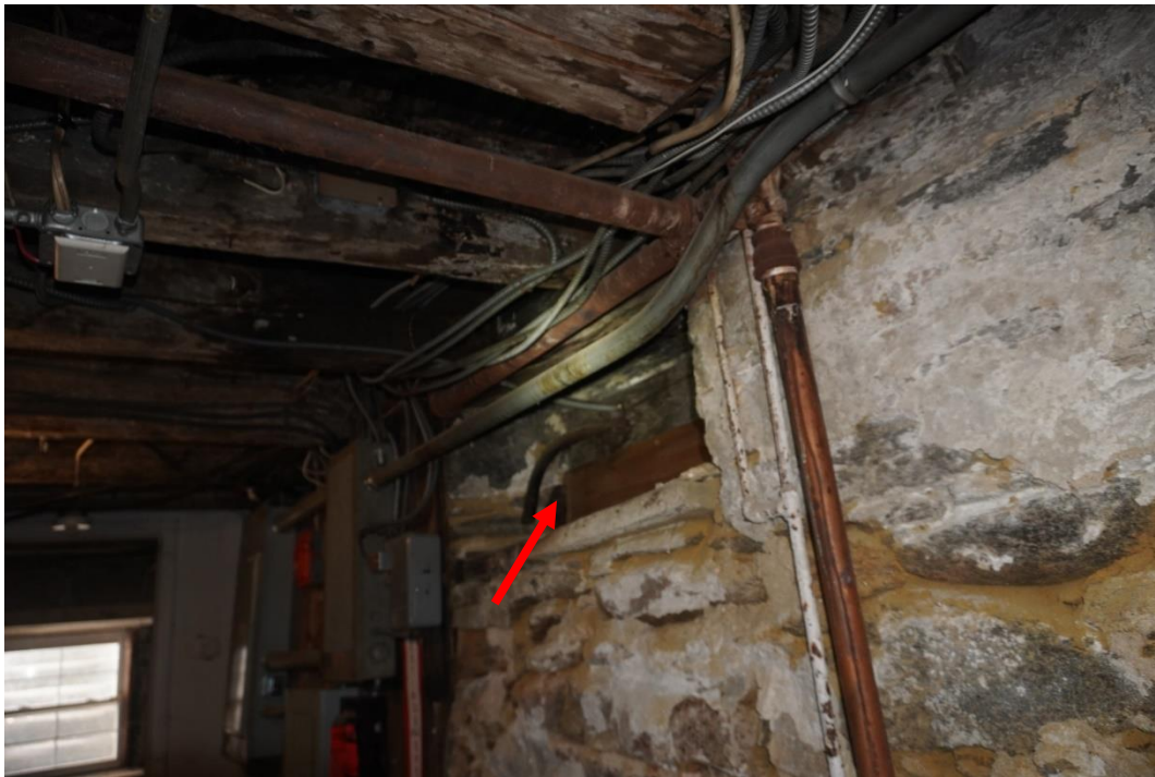
Photo #58: Cellar window at boiler room south foundation wall has been covered up when porch was added to the rear of the home.
