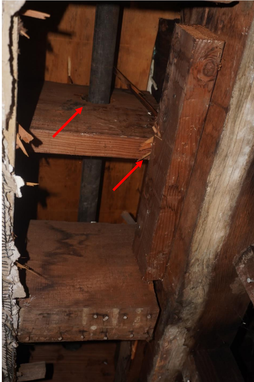
Photo #104: New joists running east to west have been installed at higher level than original joists and are resting on a 2x4 wood ledges that have been nailed to girder to support attic floor above. It is unclear why these joists were installed. Further investigation required to figure out why this was done. Original joists left in place and still supporting ceiling below. Multiple joists supporting attic floor above have holes drilled above their neutral axis at the joists ends where shear force is the highest (Probe #8).
