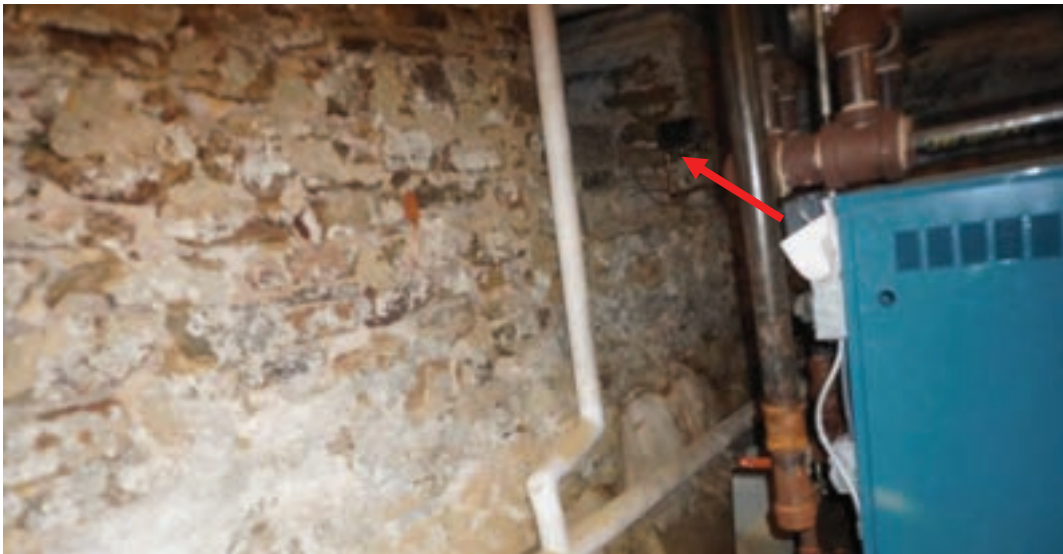
Photo #54: Piping was run into crawlspace through what potentially was an old window in original foundation wall.
