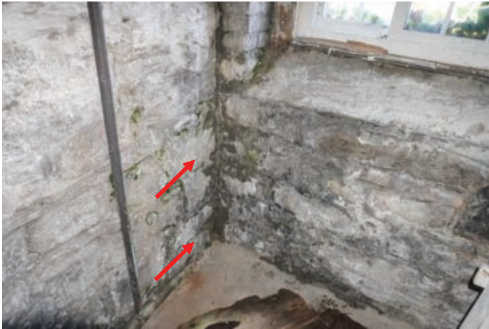
Photo #36: Water intrusion foundation wall, northeast corner of home at extension. for better or worse a feature of historic rubble stone walls; as mentioned earlier, try to send exterior water away from the building; nothing here of serious concern
