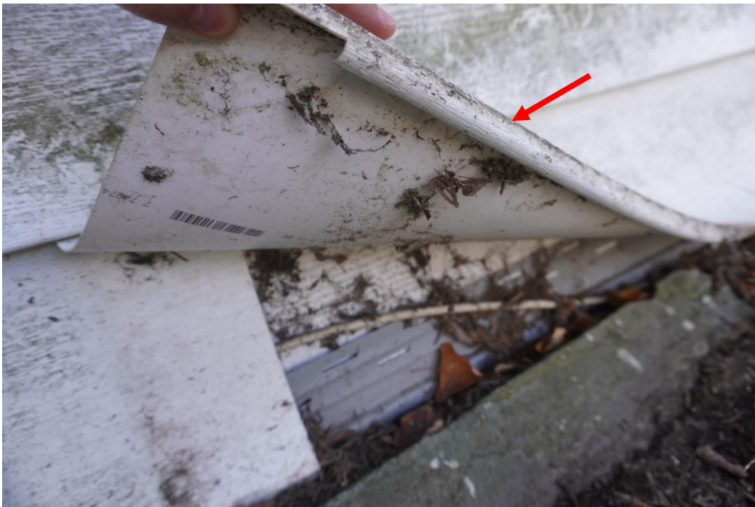
Photo #14: Exterior of building covered in vinyl siding which is not the homes original exterior building material.
