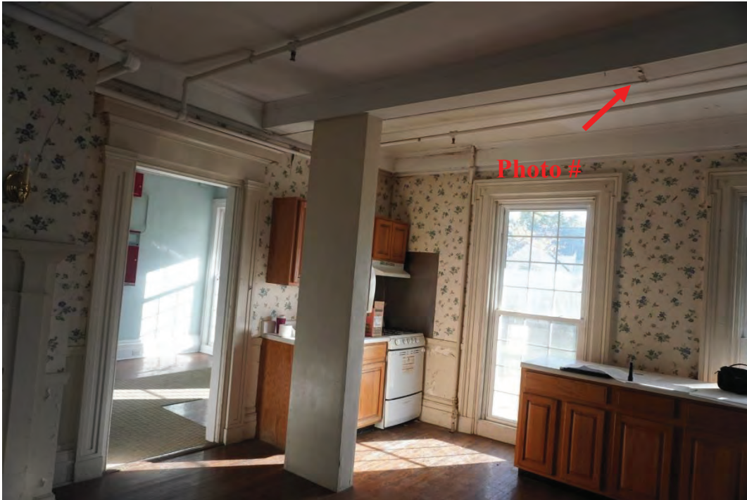
Photo #83: Soffit was opened up to further investigate crack. When soffit at this location was opened up it was empty inside and apparently was just there for aesthetic purposes (Probe #3).
