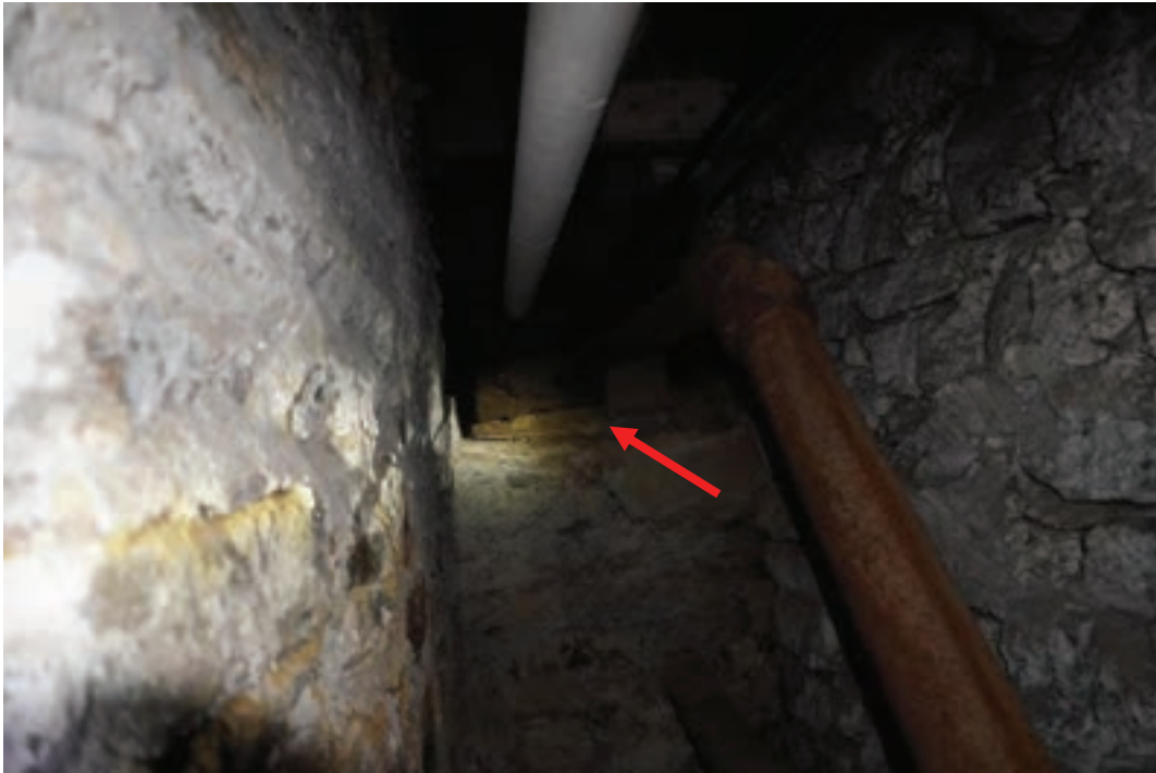
Photo #55: Piping was run into crawlspace through what potentially was an old window (second location) in original foundation wall.
