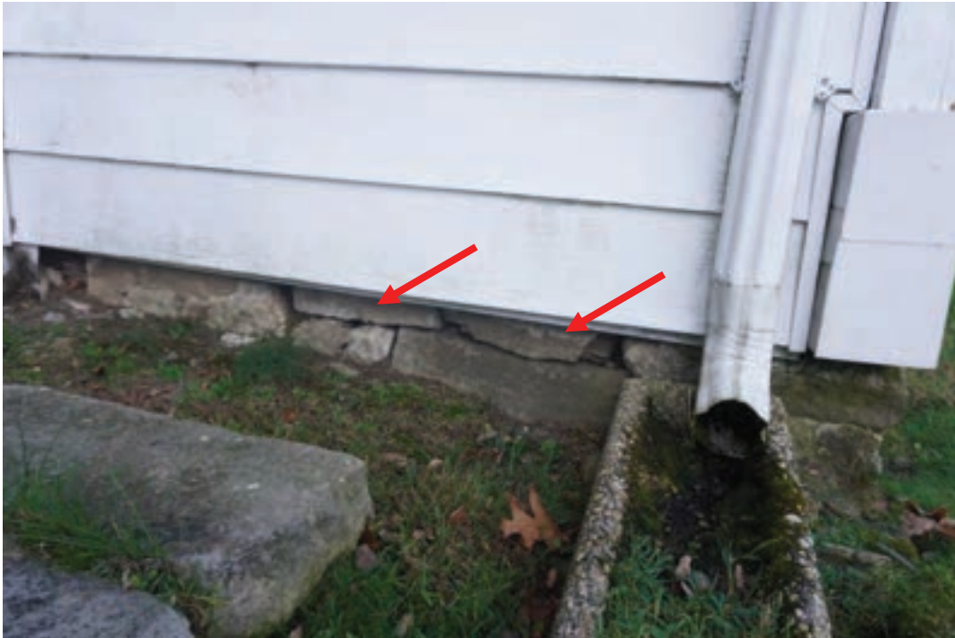
Photo #20: Exposed exterior side of rumble foundation deteriorating. No mortar between stones. loose laid footers testimony to historic foundation condition. easily addressed, repointed, if critters are entering
