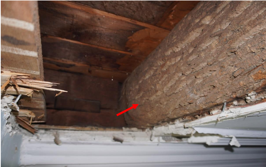
Photo #89: Ceiling joist that was never fully scored into a square framing member and still has bark exterior (Probe #4).
