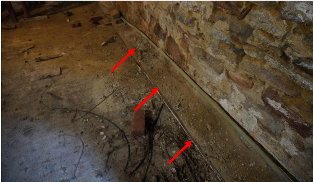
Photo #46: Water infiltrating through foundation is bringing in soil through spaces between dry laid rubble stone walls. Soil piling along inside of foundation walls.
