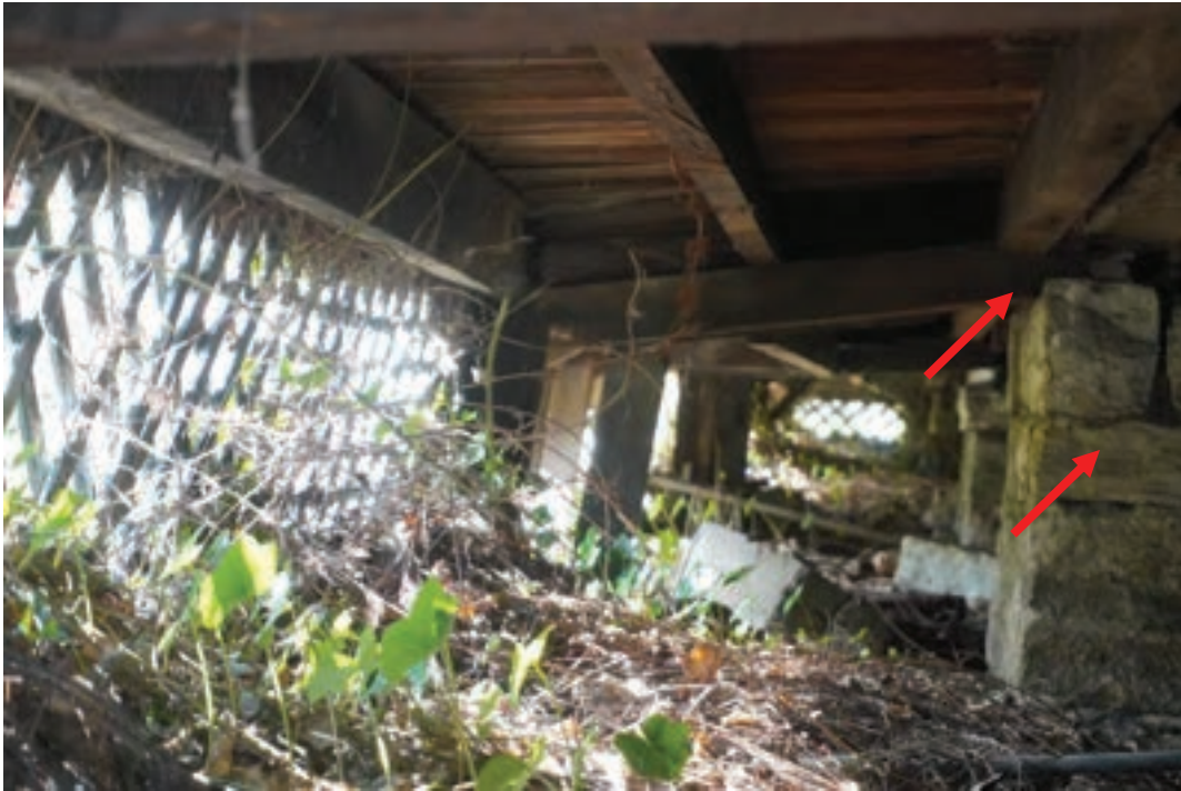
Photo #34: Rear porch sitting on stone pillars that are showing signs of deterioration. clear organic material & reset posts to maintain required slope on porch
