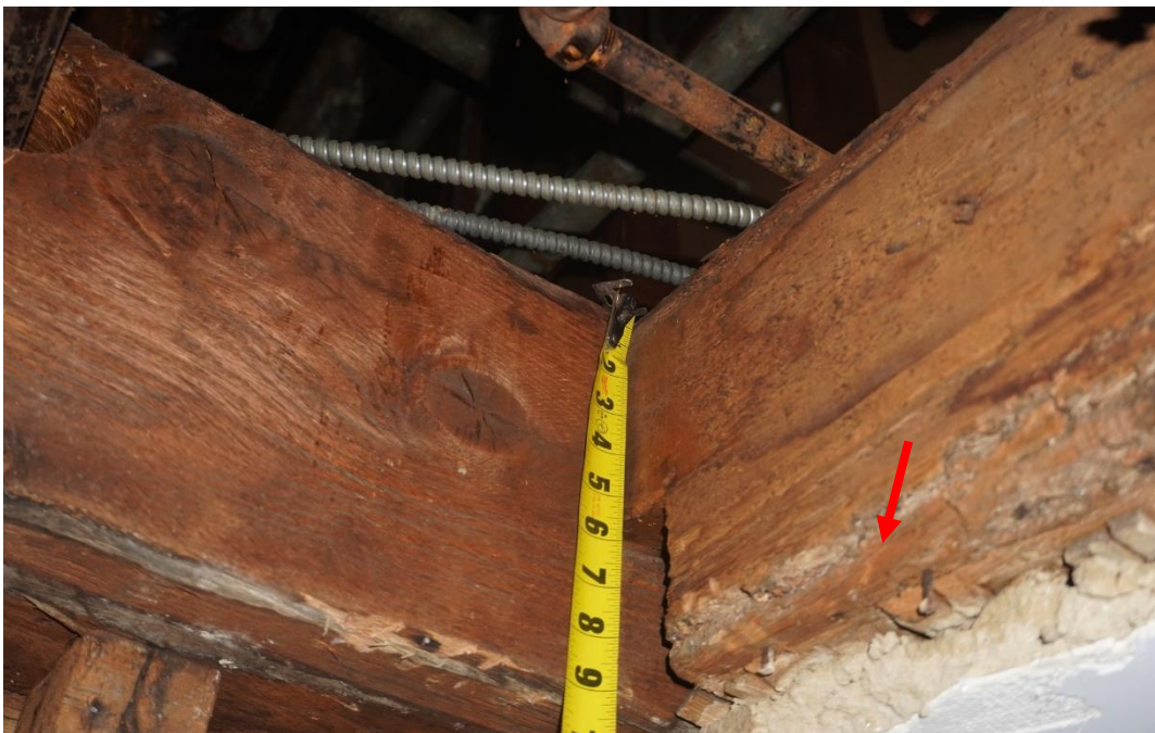
Photo #102: Past termite damage was observed in floor joist supporting attic level (Probe #7).
