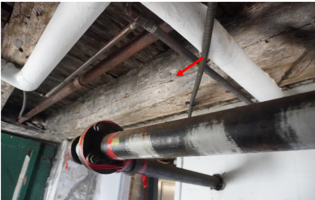
Photo #51: Horizontal crack from shear stress resonating down entire member from notch at end of beam.
