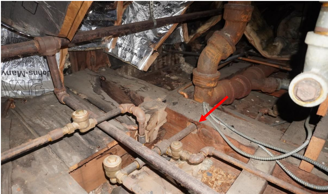
Photo #110: Pipe penetration drilled through girder drilled above its neutral axis. Observed in unfinished attic area, north side of original structure.
