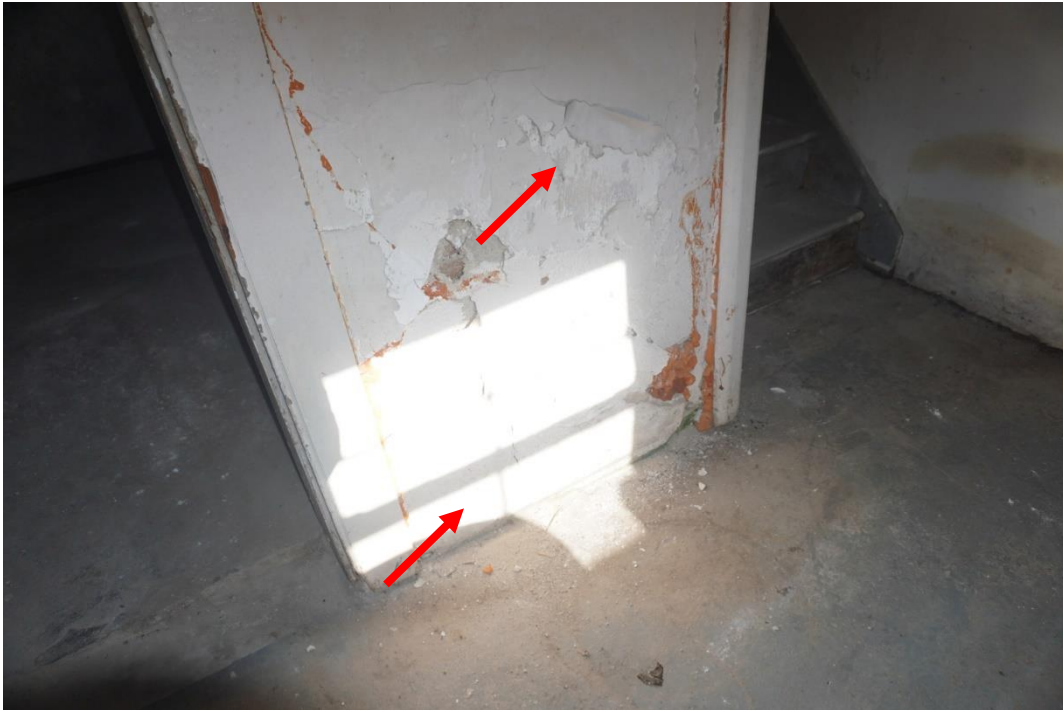
Photo #38: Mold formation and deteriorating damp plaster interior walls at cellar level due to water wicking up through cellar floor.
