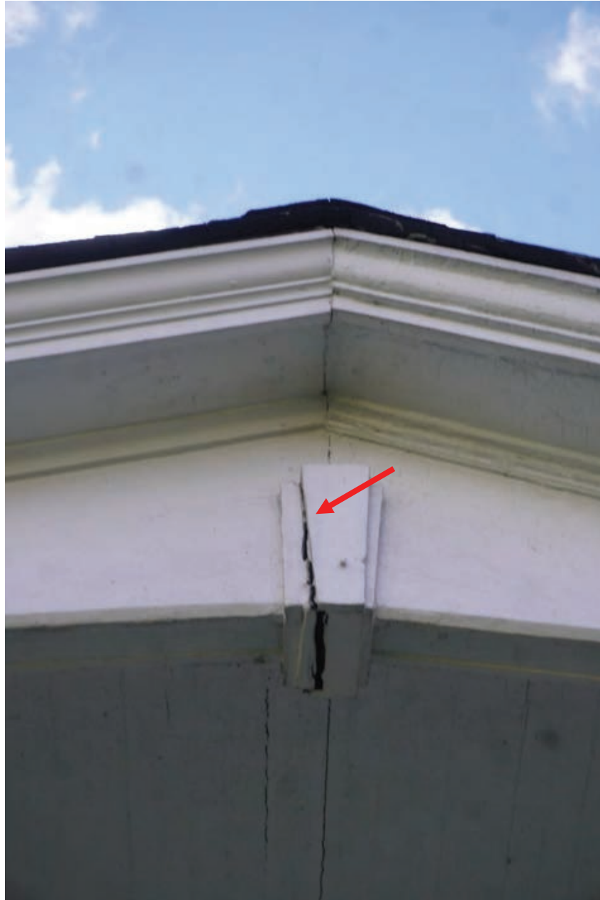
Photo #18: Vertical crack running down middle of front portico. shrinkage & expansion but not remotely more than a normal exterior repair issue
