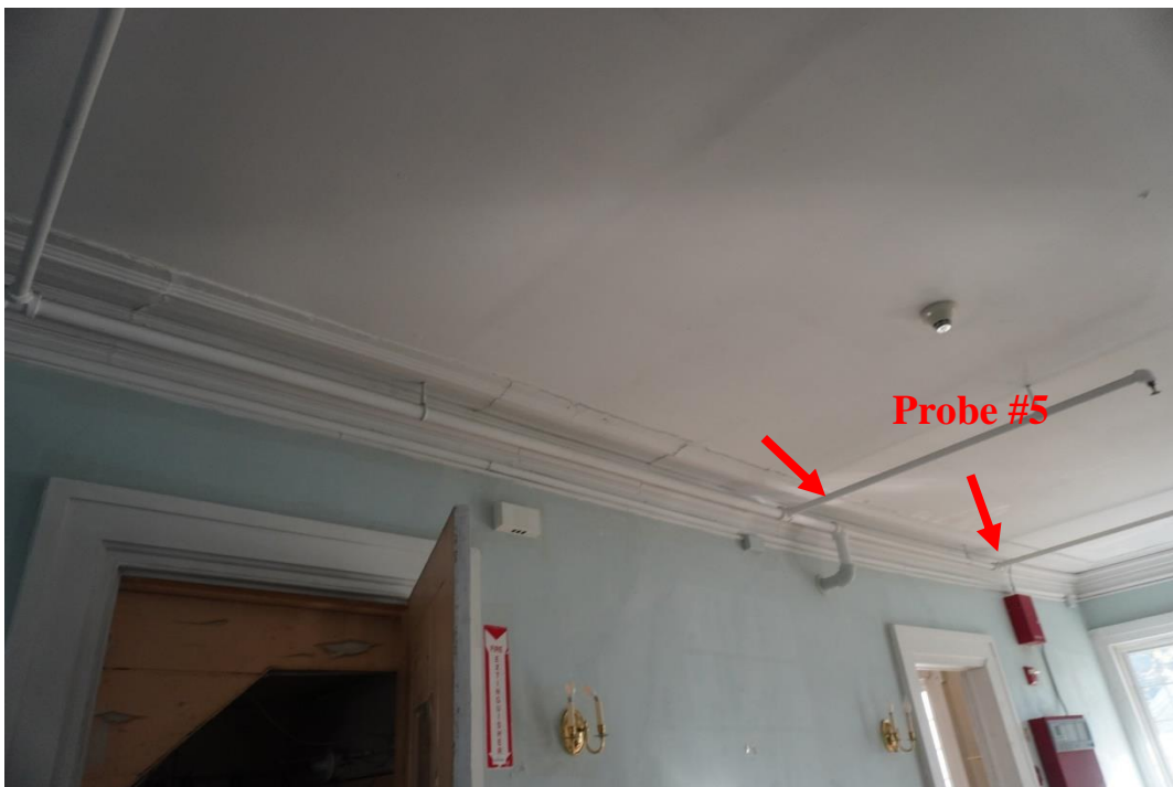
Photo #94: Wall containing girder beam showing signs of deflection. This girder is directly above girder that is failing in the boiler room area and is being propped up with temporary columns (Probe #5).
