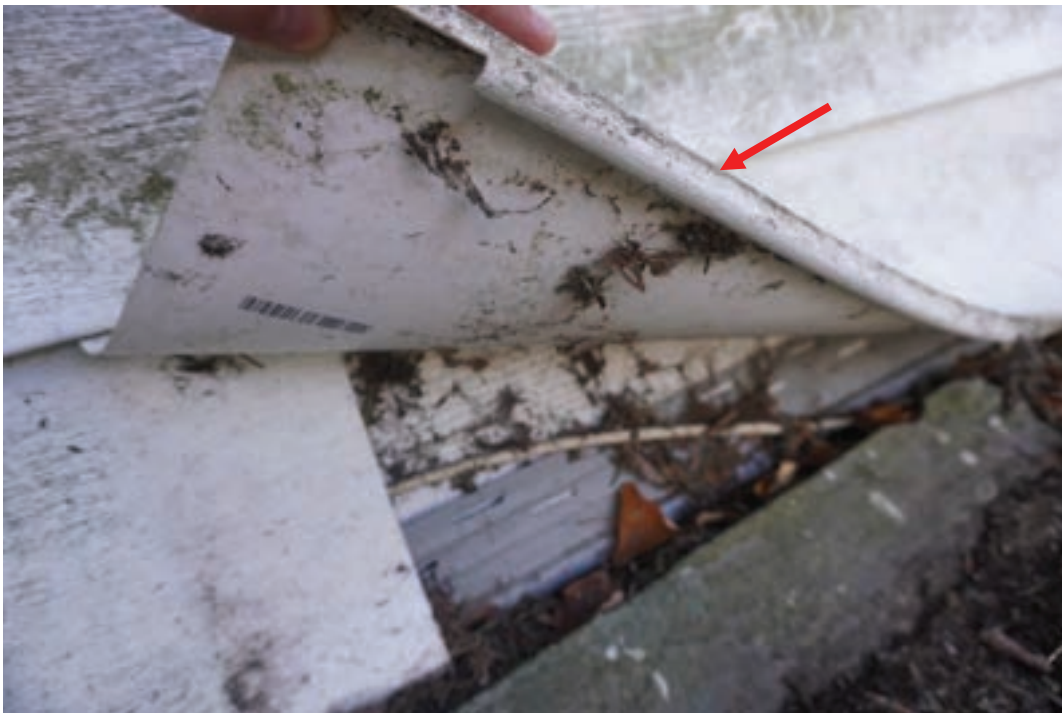
Photo #14: Exterior of building covered in vinyl siding which is not the homes original exterior building material.
