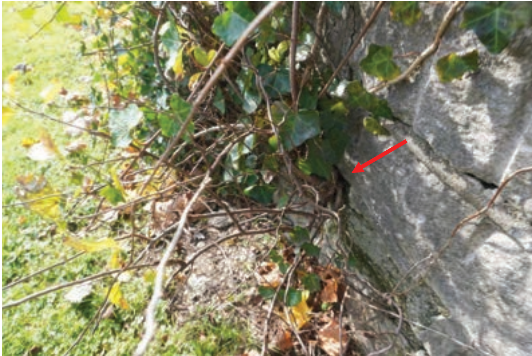
Photo #3: Retaining wall that runs from between front entrance and driveway is deteriorating throughout. Roots/ large weeds growing through joints of walls multiple locations.
