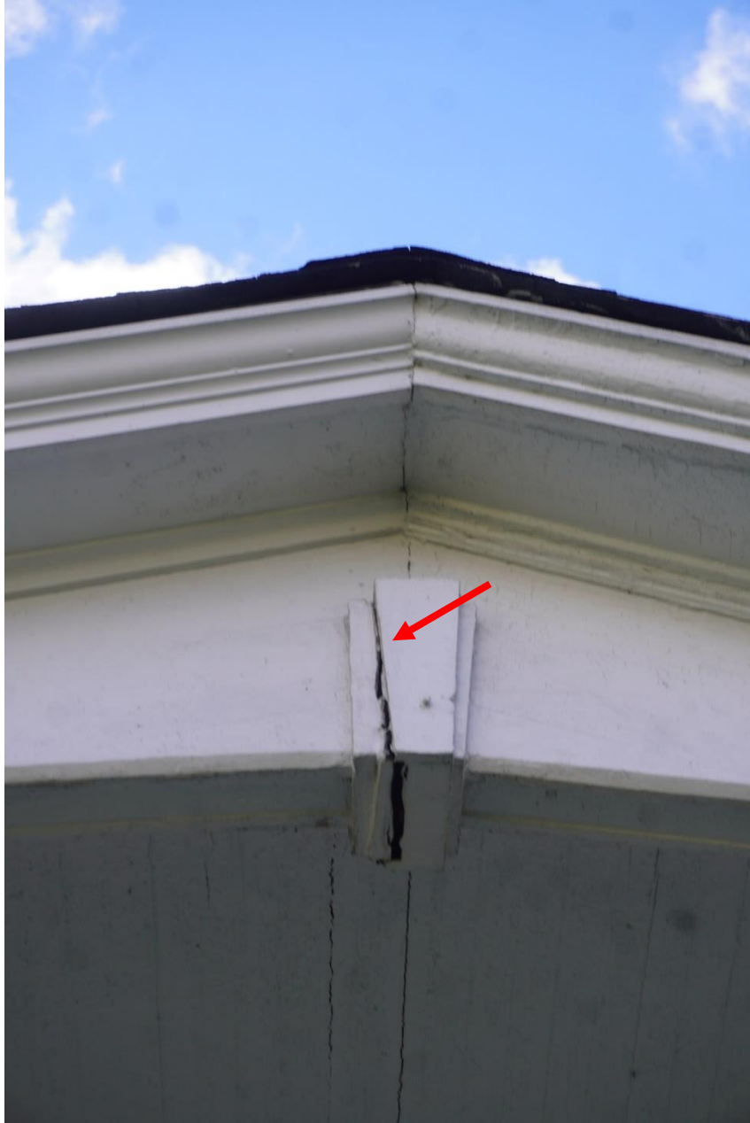
Photo #18: Vertical crack running down middle of front portico.
