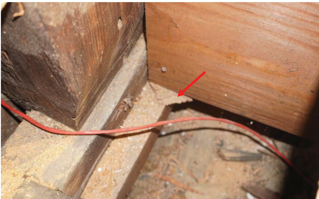
Photo #116: New wood joists have been installed going east to west bearing on wood ledge that has been nailed into girder. It is unclear why this was done. Further investigation required (Probe #12).
