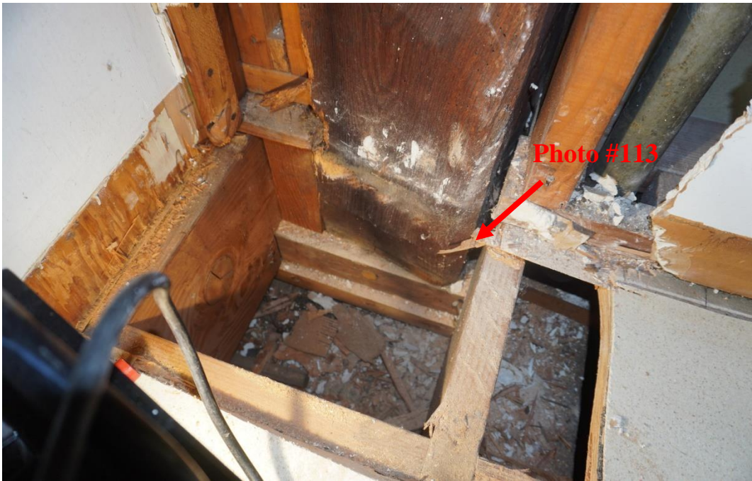
Photo #112: Post in attic space has moved out of place. Mortise and tenon joint that was connecting post to girder below has failed allowing member to rotate (Probe #11).
