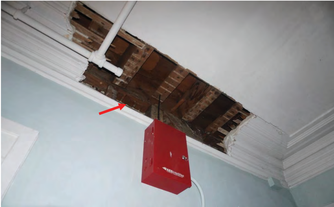
Photo #95: Interior girder that is showing signs of deflection. Girder is directly above girder that is failing in the boiler room area and is being propped up with temporary columns (Probe #5).
