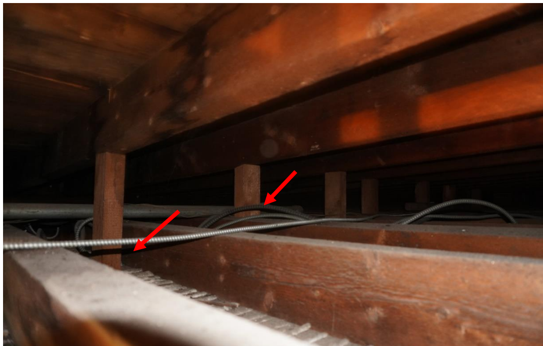
Photo #108: View facing northeast in roof void between 2 nd floor ceiling joists and roof joists in the addition. Roof joists do not align with ceiling joists and are being supported at midspan with blocking that is resting right onto plaster ceiling (Probe #9).
