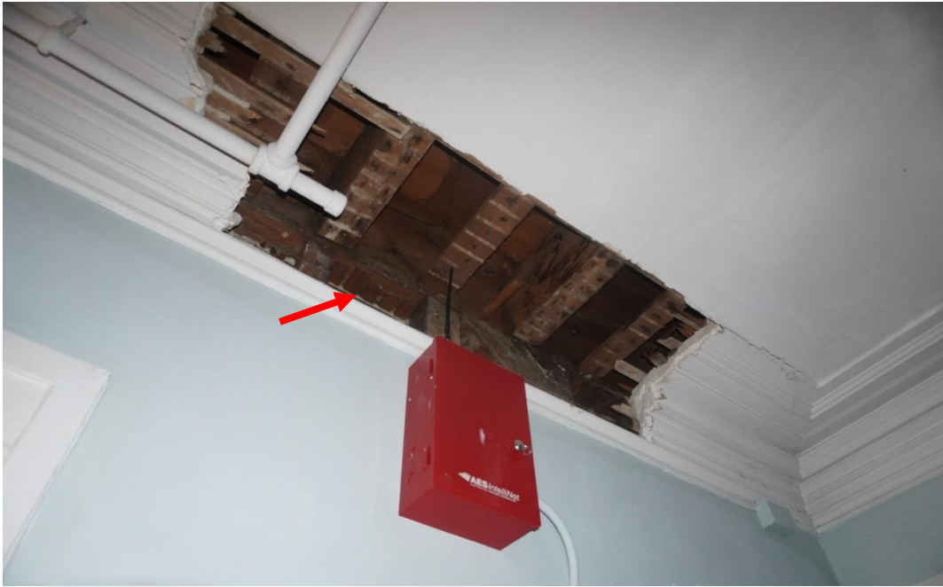
Photo #95: Interior girder that is showing signs of deflection. Girder is directly above girder that is failing in the boiler room area and is being propped up with temporary columns (Probe #5).
