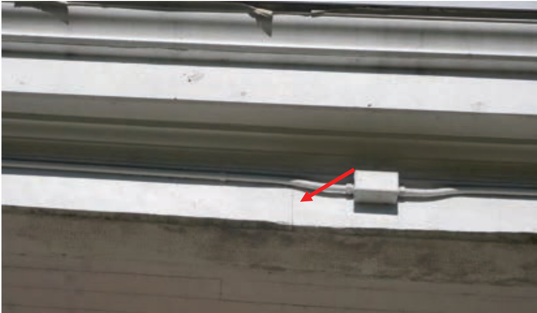
Photo #26: Rear porch roof deflecting over stairs causing water to pool and leaf build up.
