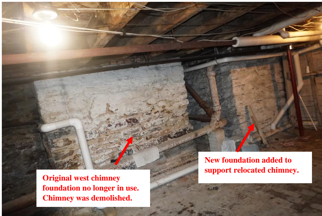
Photo #57: Original west chimney was relocated at some unknown time in the past.
