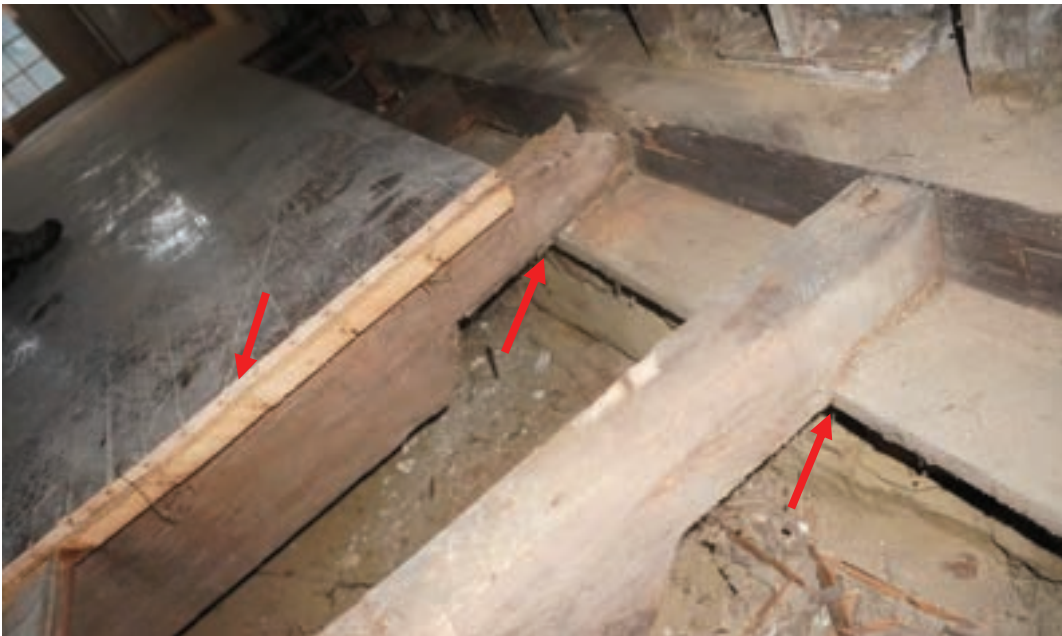
Photo #70: Original floorboards above crawlspace have been removed. New wood flooring directly attached to joists. Crawl space joists sitting on an improperly supported sill plate (Probe#1).
