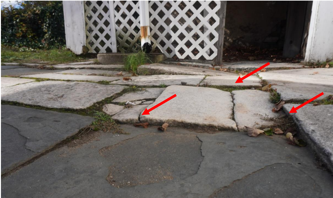
Photo #9: Stone slabs have settled/ heaved creating multiple trip hazards, stone patio rear yard.
