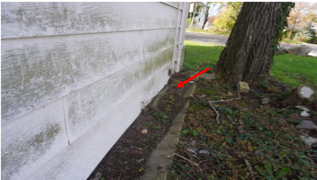
Photo #6: Negative grading front of home between entrance and northwest corner of home. Water pooling up against exterior foundation wall of crawlspace.
