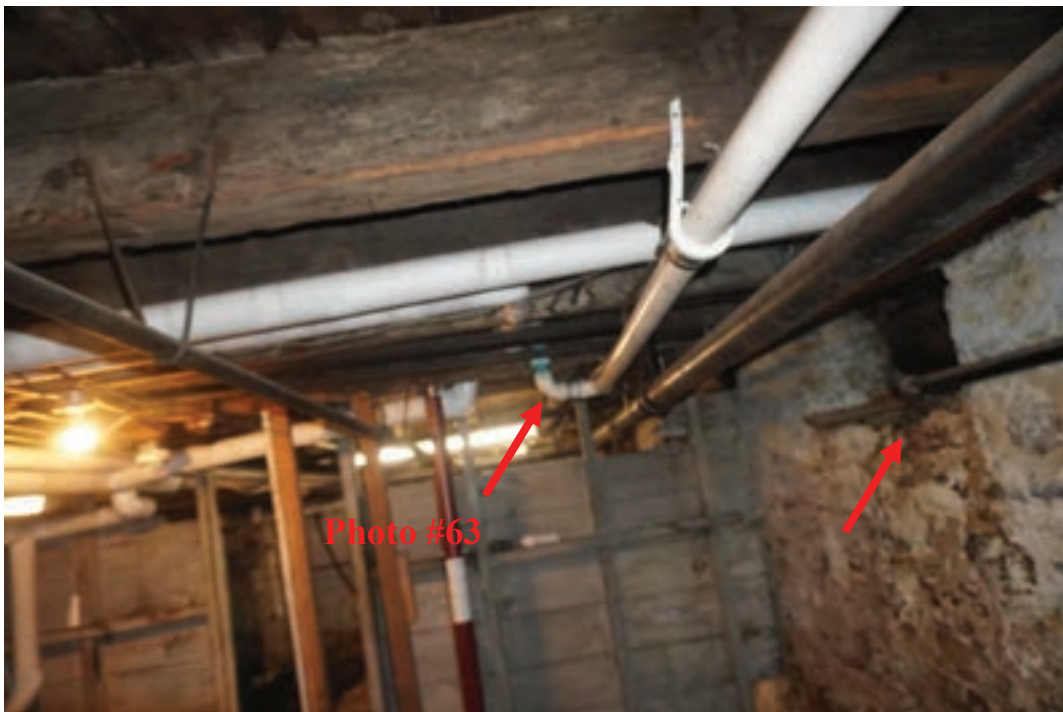
Photo #62: Cellar window (second location) at west end of home on south foundation wall has been covered up when porch was added to the rear of the home. Plumbing pipe drilled directly through main girder in the vertical direction, west end of cellar.
