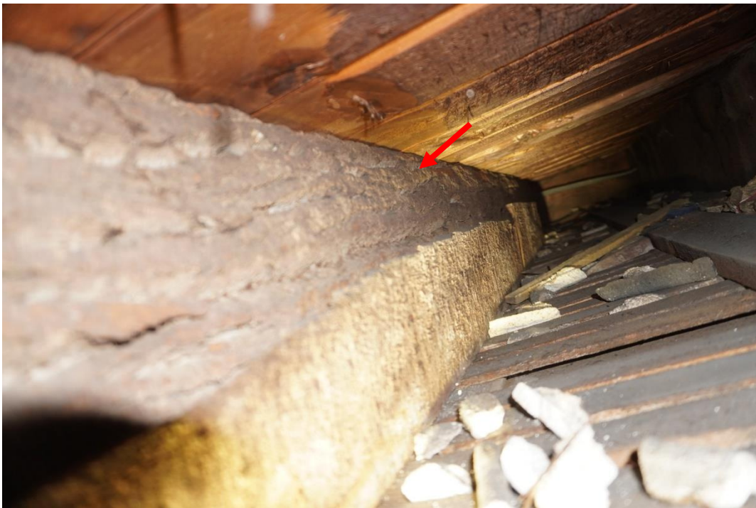
Photo #90: Ceiling joist that was never fully scored into a square framing member and still has bark exterior (Probe #4).
