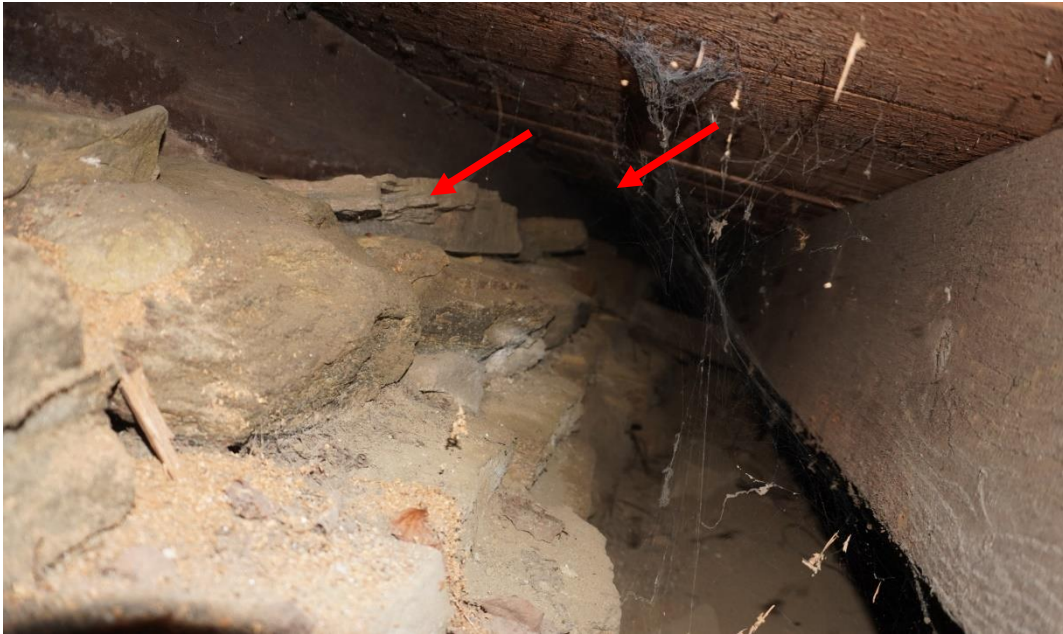
Photo #73: Exterior foundation along north side of home below sill beam is deteriorating and observed to have displaced. (Probe #1)
