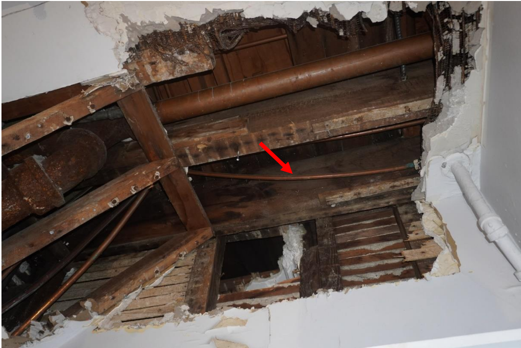
Photo #97: Girder beam that runs north to south in wall that use to be the exterior wall of the original structure (Probe #6).
