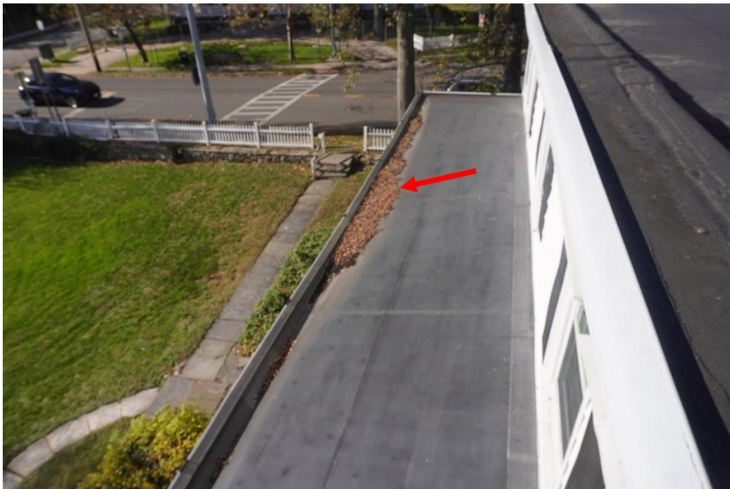
Photo #27: Rear porch roof deflecting over stairs causing water to pool and leaf build up.
