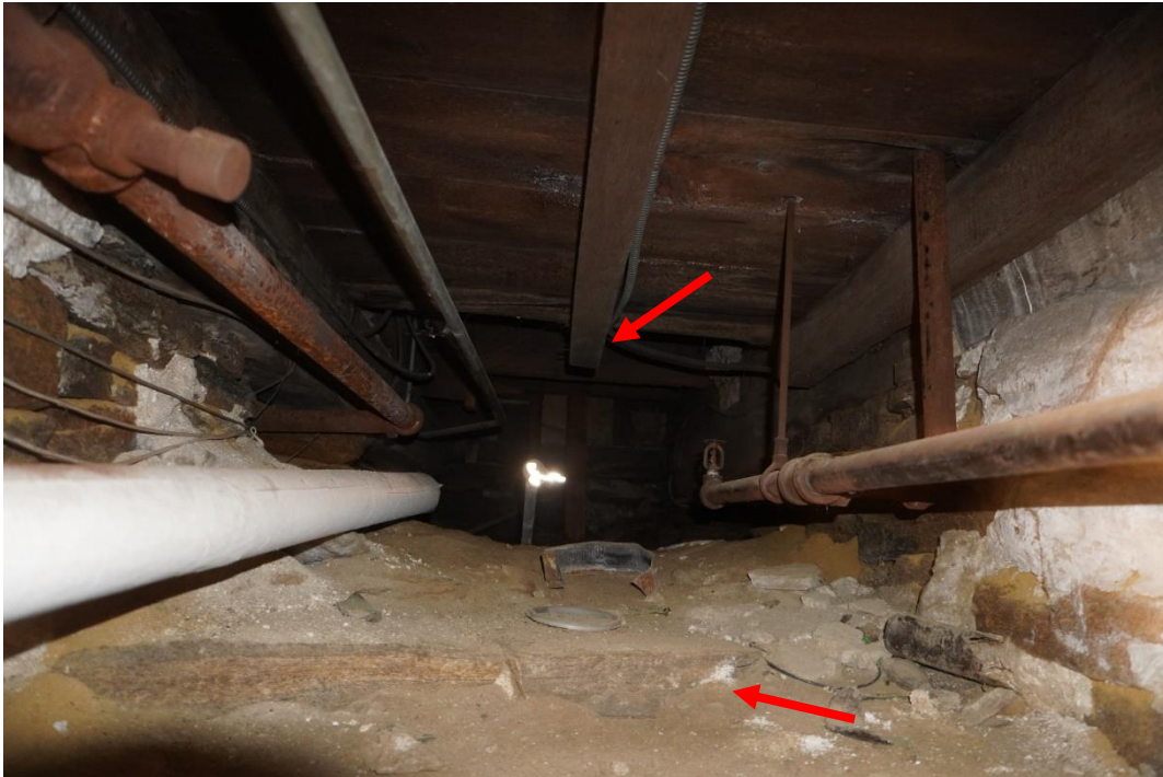
Photo #53: Joists connections in crawlspace observed to be coming apart. Piping was run into crawlspace through what potentially was an old window in original foundation wall.
