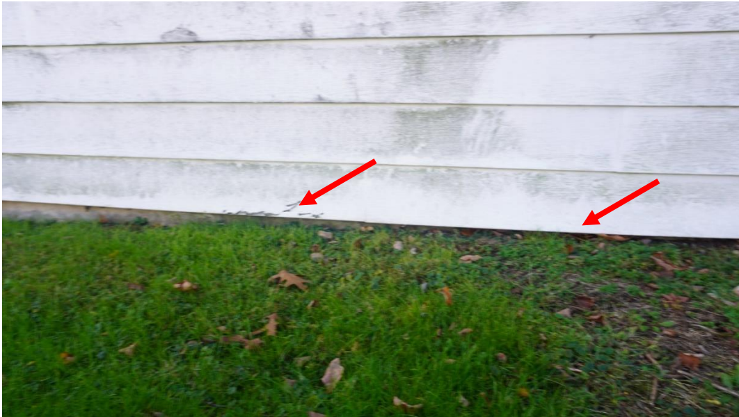
Photo #15: Foundation along front façade of original structure is low and at same level as grading. Water can infiltrate above foundation wall and rot out wood sill beam that runs along top of foundation.
