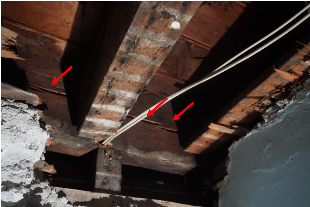
Photo #92: Interior girder running north to south is splitting along the mortise and tenon joint connections (Probe #4).
