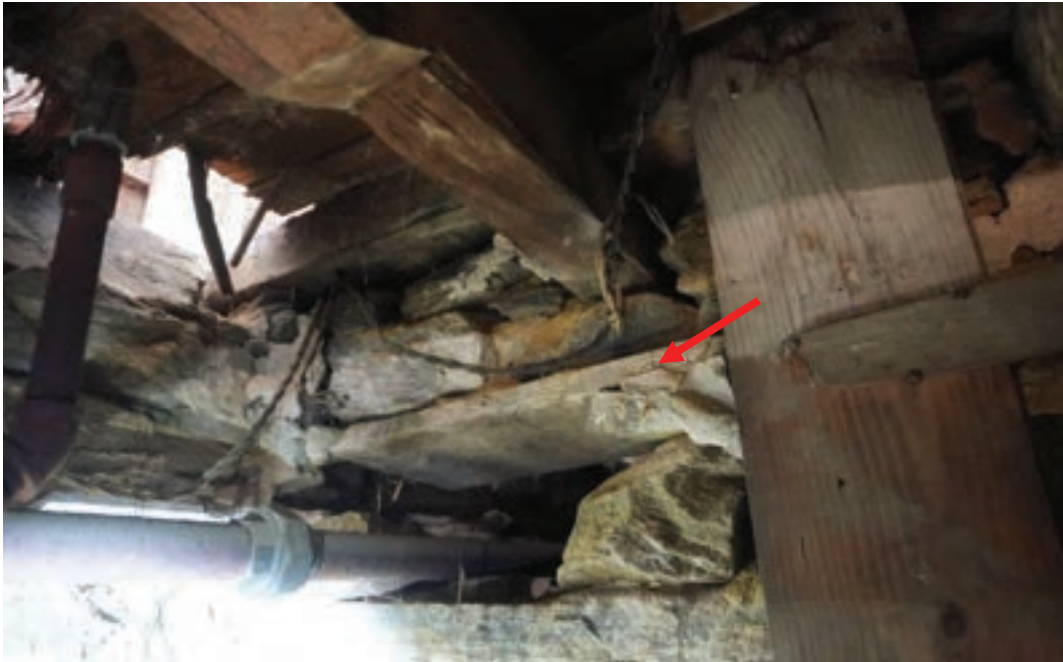
Photo #65: Joist with inadequate support resting on foundation wall that is deteriorated and that has been damaged to make a pipe penetration into crawlspace.
