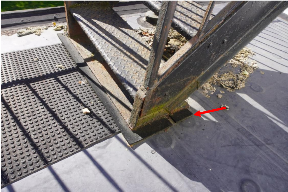
Photo #30: Exterior metal stair egress just sitting on roofing membrane and not attached to structure.
