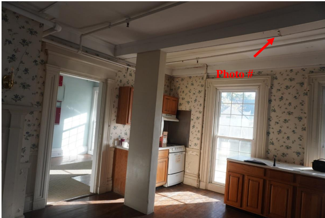
Photo #83: Soffit was opened up to further investigate crack. When soffit at this location was opened up it was empty inside and apparently was just there for aesthetic purposes (Probe #3).
