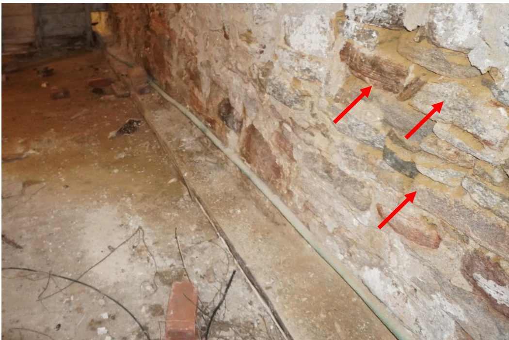
Photo #47: Water infiltrating through foundation is bringing in soil through spaces between dry laid rubble stone walls. Soil piling along inside of foundation walls.
